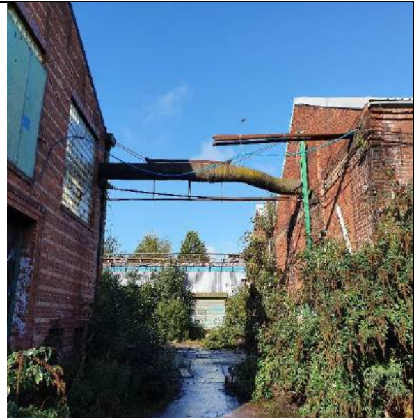
Photograph 10: Pipe connecting B2 and B3
