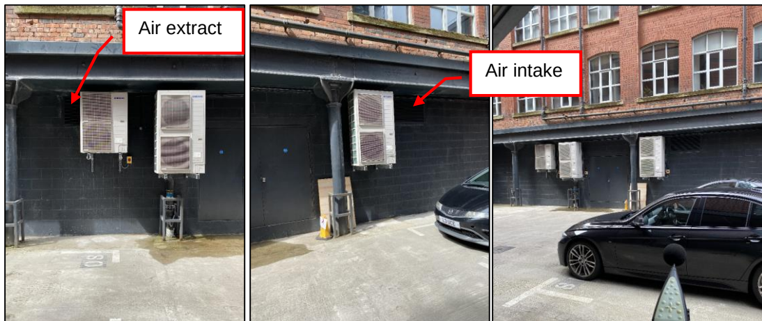
Figure 3.1 - Photographs showing outdoor condensing units and air intake/extract louvres
