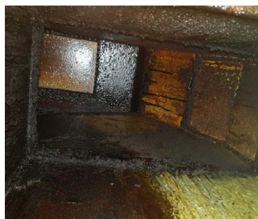
Figure 1 - Grease build-up in extract ductwork
