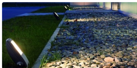
ARCHITECTURAL EXTERIOR FLOODLIGHTS
