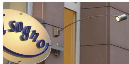
FASCIA & SIGN LIGHTS
