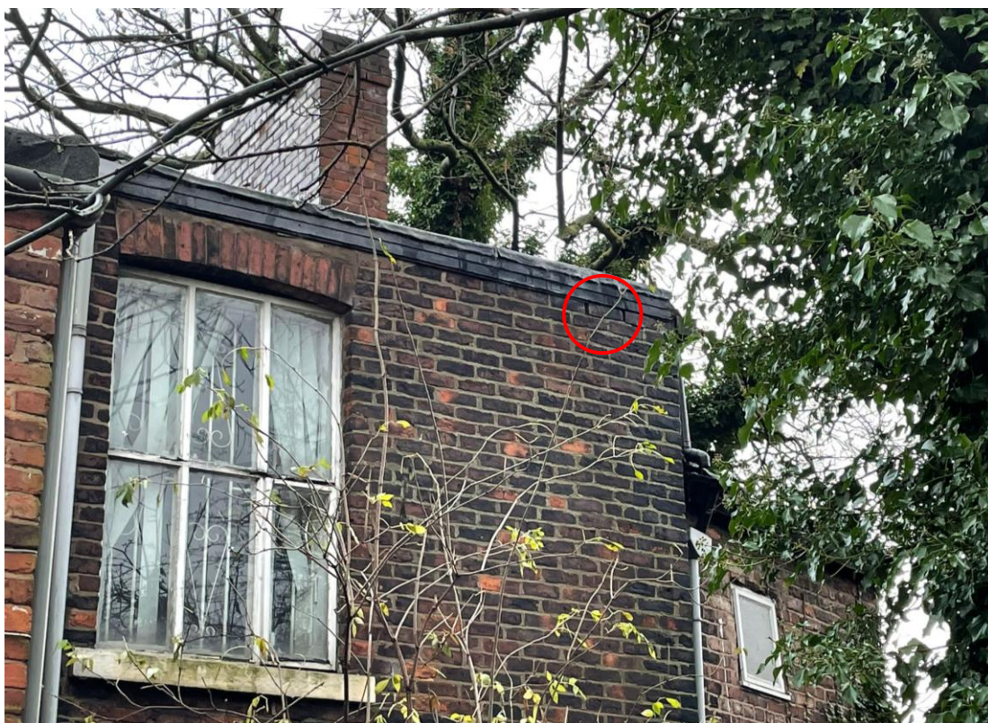
Photograph 7 – South-eastern aspect with lifted lead flashing and missing mortar between bricks.
