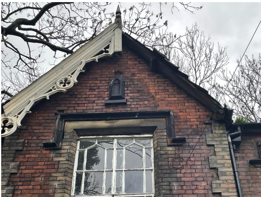
Photograph 3 – North-western aspect, where the barge board is partially missing from the gable end, with gaps present between the eaves, brickwork and lintels.
