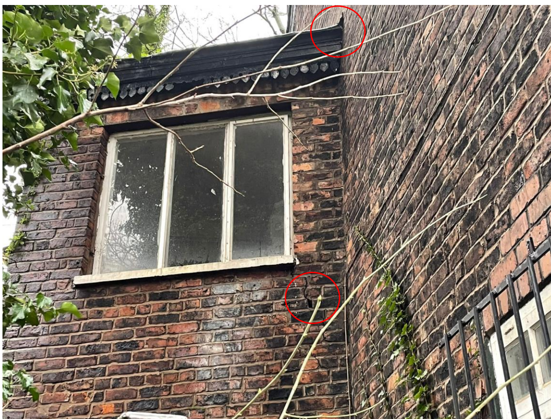
Photograph 12 – North-eastern flat-roofed extension with damaged fascia's, lifted lead flashing, timber window frame in good condition, and gaps in brickwork.
