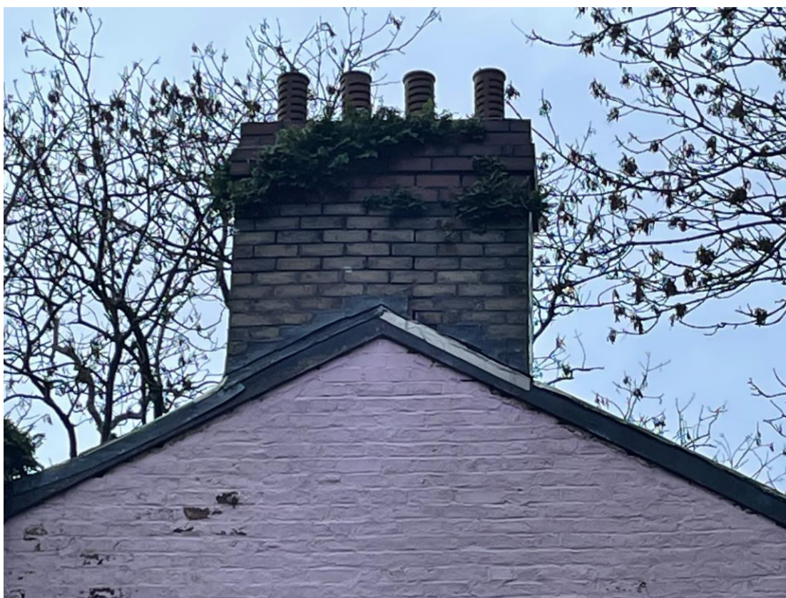
Photograph 2 – South-western aspect with established vegetation on the brick chimney, missing lead flashing, and gaps between bricks and the barge board.
