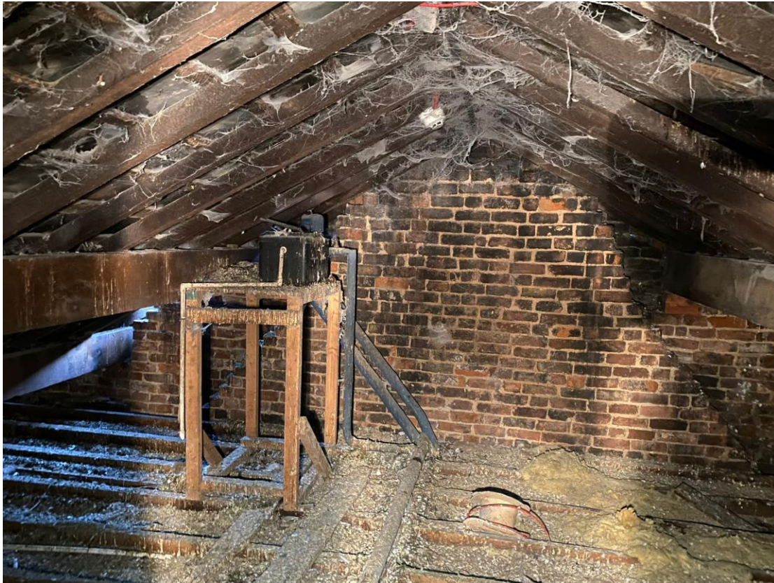
Photograph 15 – Section 1 with traditional purlin timber rafters, lined with bitumen roof felt, dense cobwebs, brick gable ends in poor condition, and guano covered insulation.
