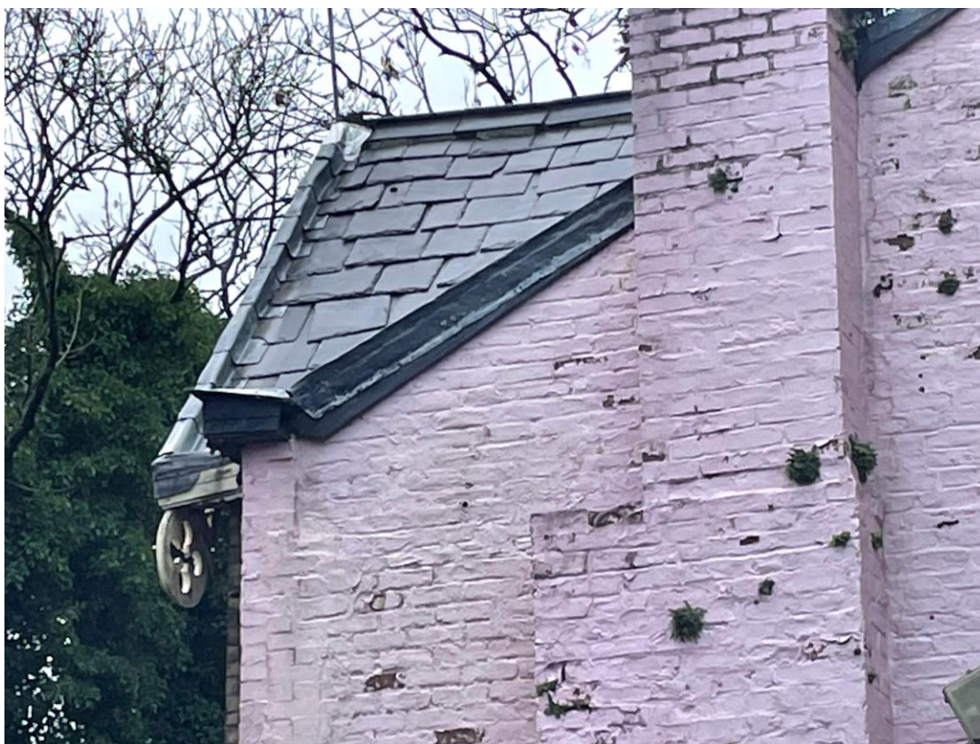
Photograph 1 – The building's south-western aspect, with raised lead flashing and barge boards, loose roof tiles, gaps present under the ridge tiles and the box soffit.
