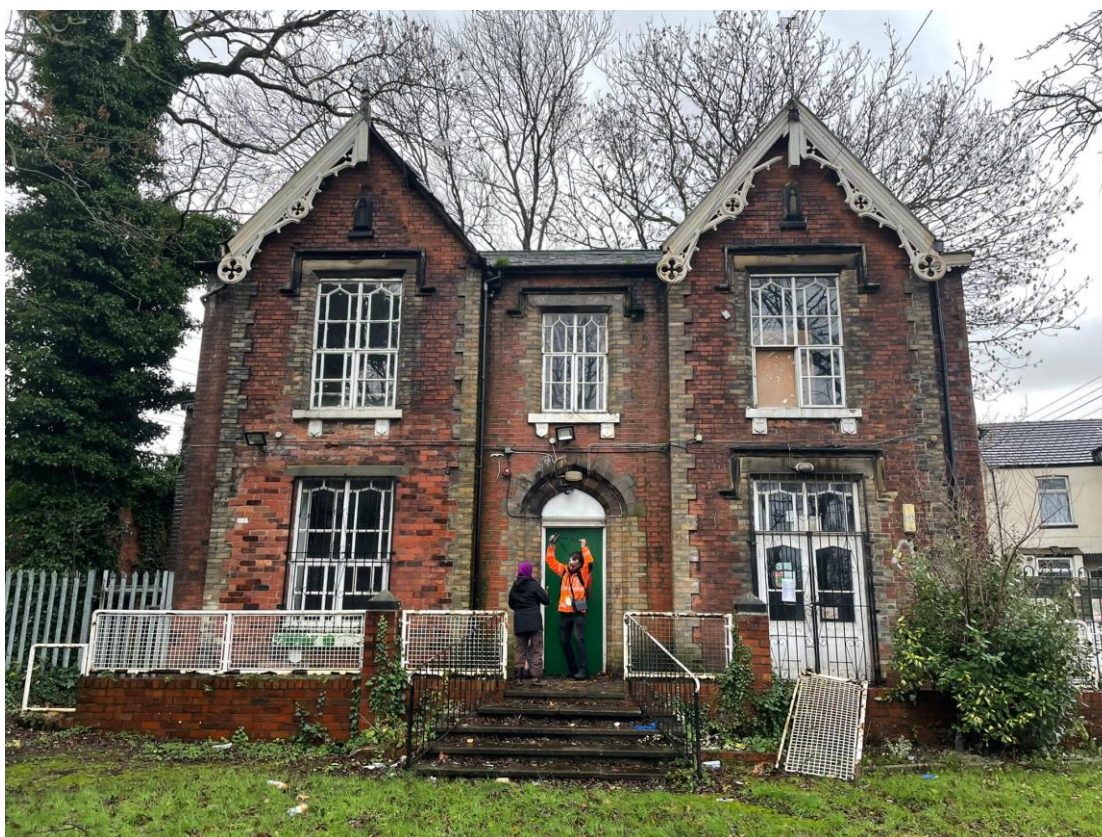
Photograph 10 – North-western aspect of Slade Lane Neighbourhood Centre twin gable ends, with damaged barge boards, several large windows and arched doorway.
