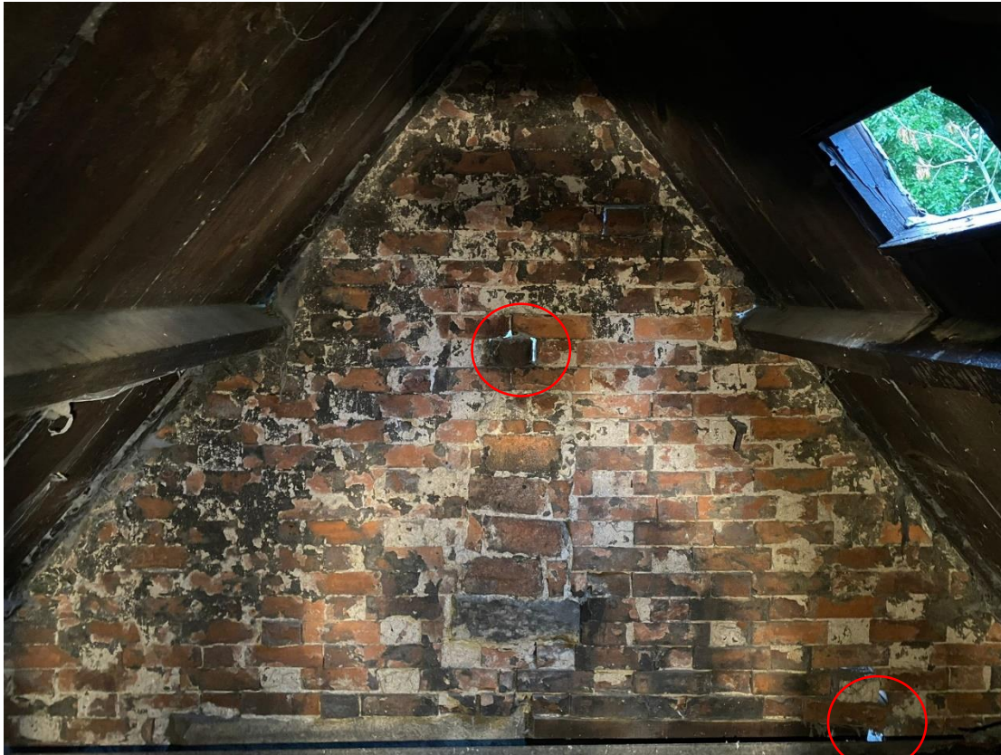
Photograph 14 – North-western gable end in section 2, with timber rafters lined with sarking boards, skylight lacking windowpane, and light entering through brick wall in poor condition.
