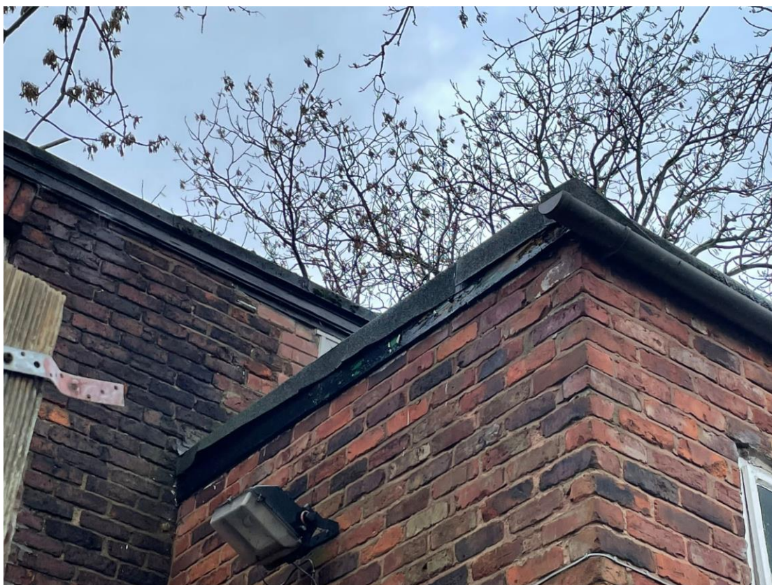
Photograph 11 – The south-eastern extension displaying the bitumen roof felt that has lifted from the flat roof, with the bonded red brick structure and timber window frame.
