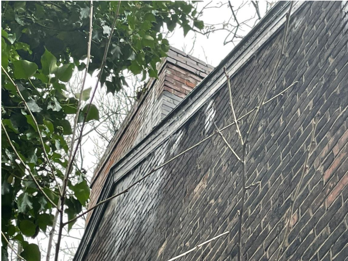
Photograph 6 – North-eastern aspect where barge boards have lifted from the brickwork.
