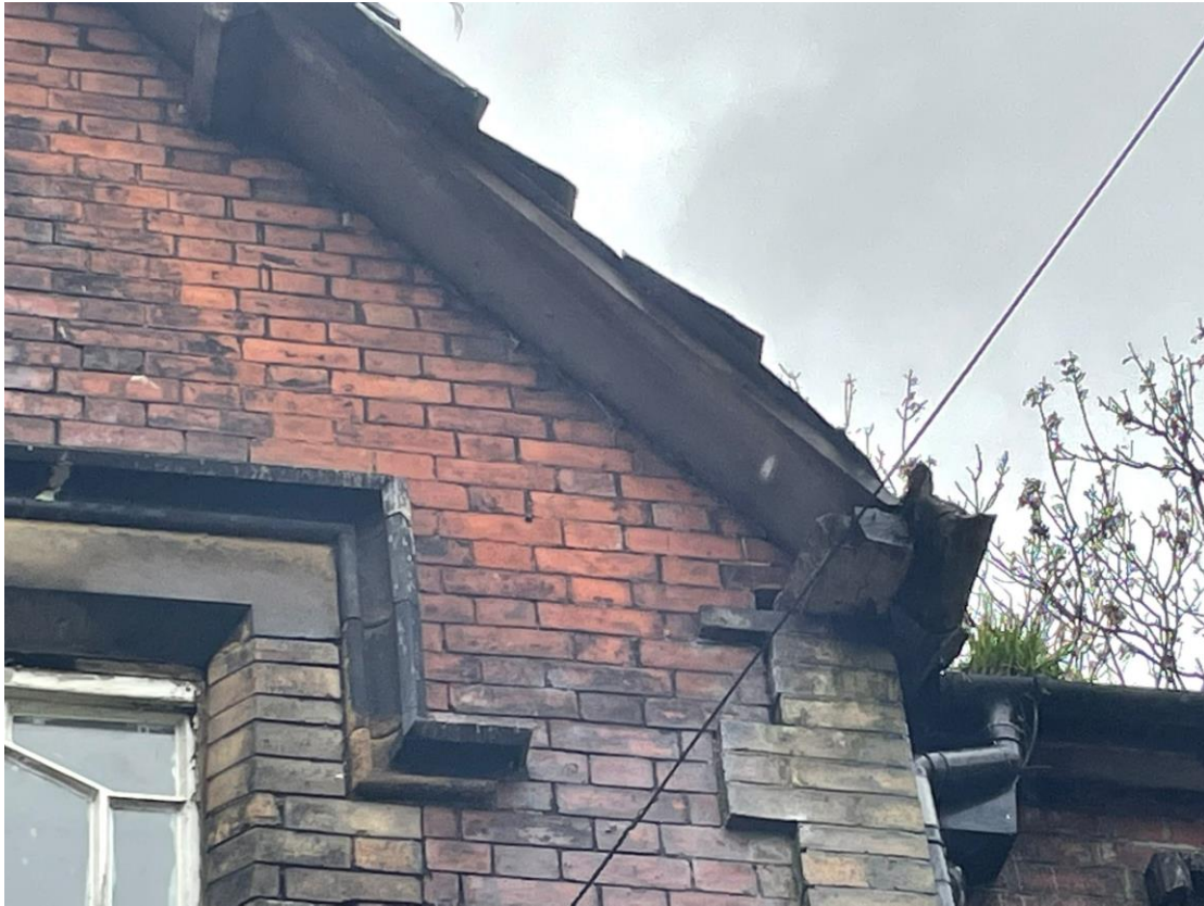
Photograph 5 – Gable-end at the north-western aspect with large gaps present under the eaves and where bricks are damaged.
