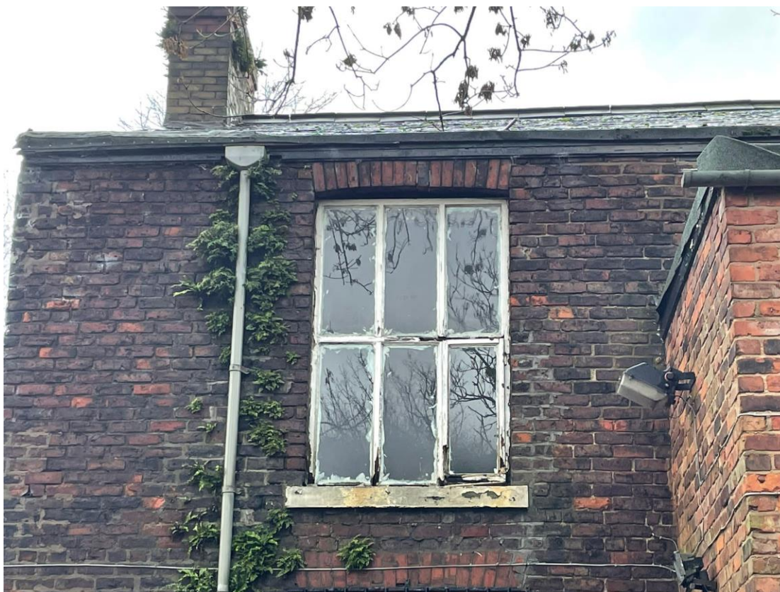
Photograph 9 – South-eastern aspect with rotten timber window frames housed by brick lintels and lifted bitumen roof felt of the southern brick extension.
