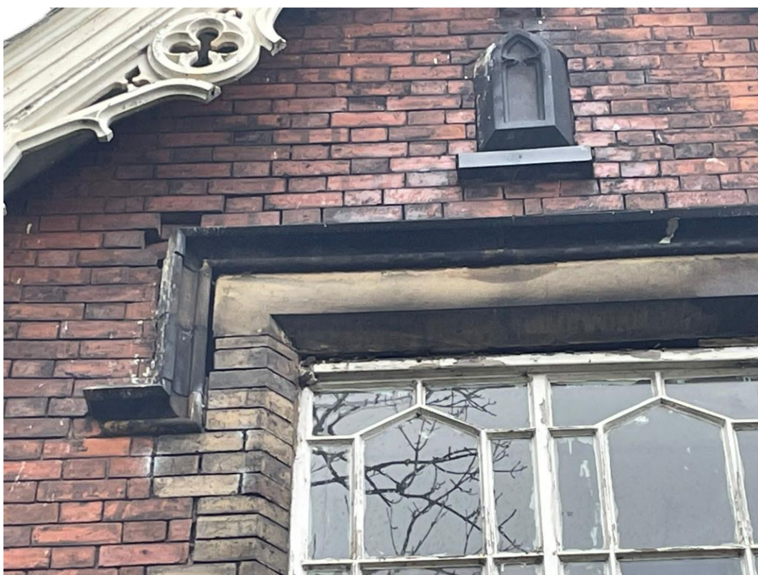
Photograph 8 – Damaged bricks and numerous gaps between the lintels, brickwork and rotten window frames.
