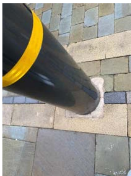
24. Condition of bollards
