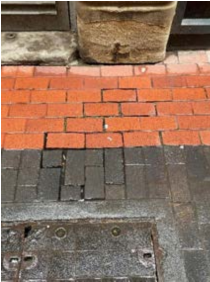
13. Missing mortar – loose bricks
