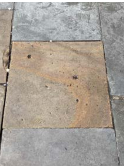
41. Two chips / damage to tile
