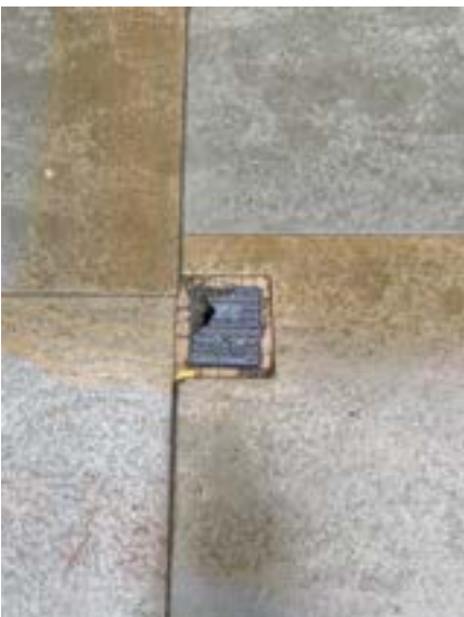
17. Cracked service chamber
