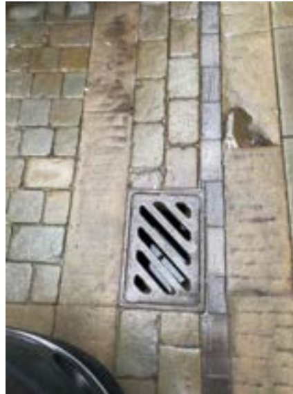
30. Blocked drainage inspection chamber
