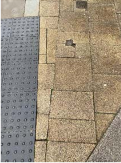
19. Cracked paving tiles
