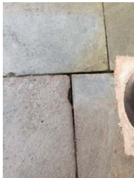
18. Slight chip to paving tile
