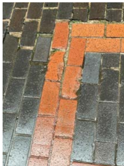
12. Significant damage to feature bricks
