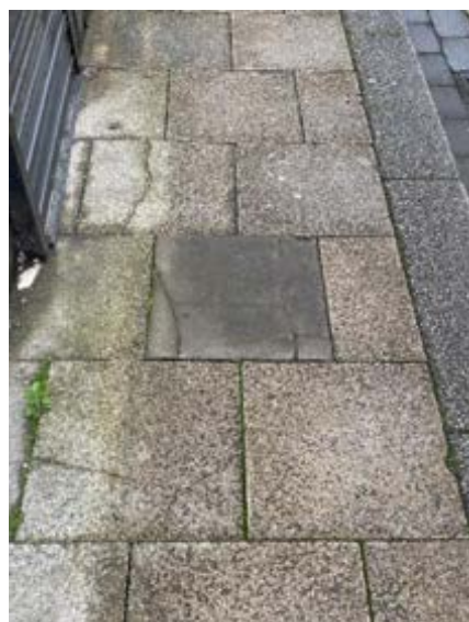
28. Replacement tile and multiple cracks
