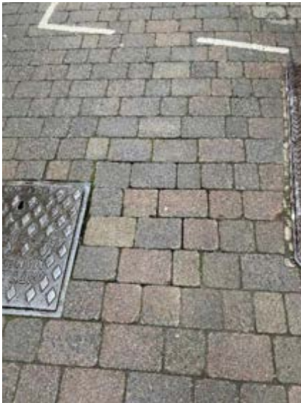
9. Section of loose bricks
