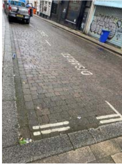
2. Disabled bay with some fading to paint
