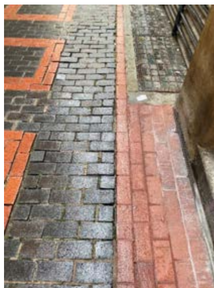
6. Loose bricks along pathway
