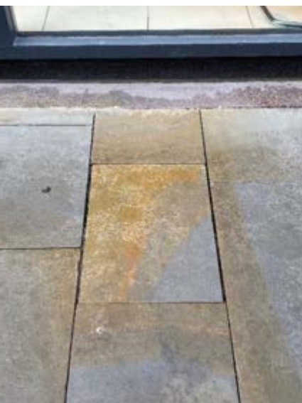
11. Loose paving stone
