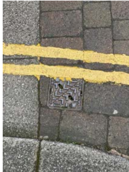
14. Water service chamber
