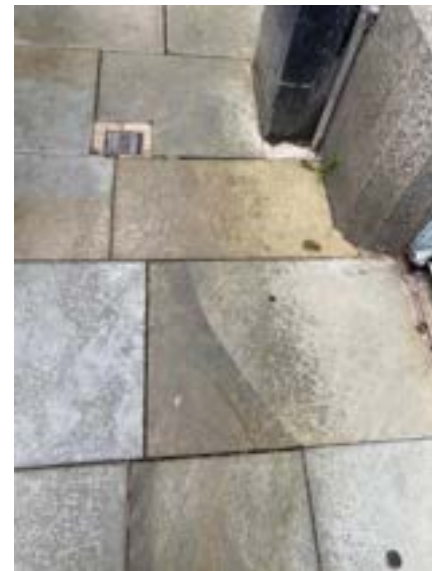
4. Crack in stone paving
