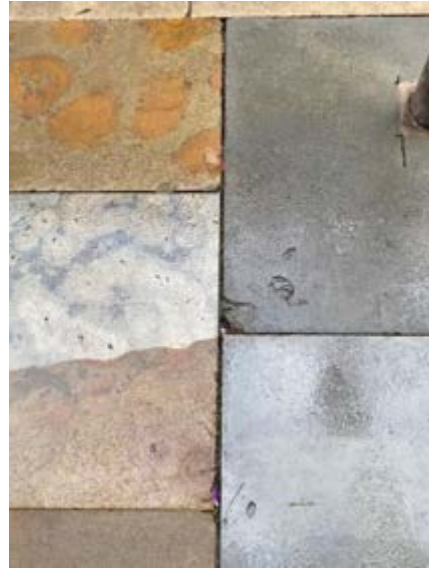
38. Damage to tile
