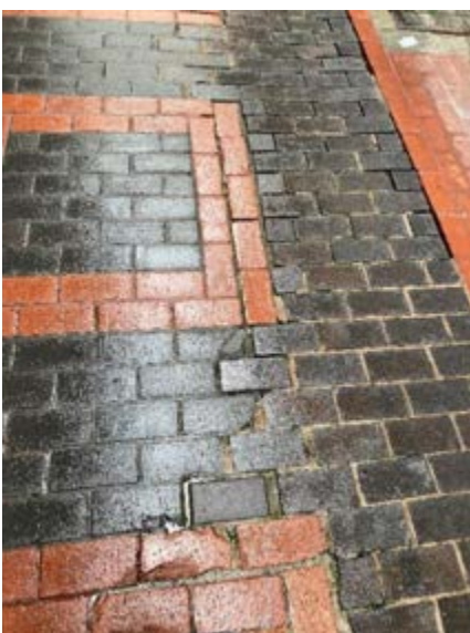
11. Change in mortar colour. Some damage to bricks
