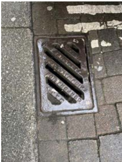
15. Partially blocked (corner) inspection chamber
