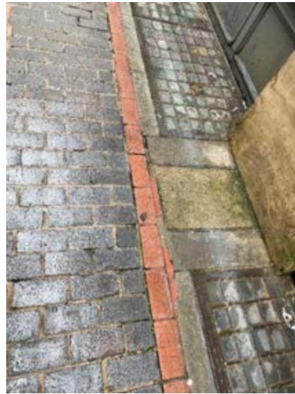
8. Loose bricks and damaged concrete infill
