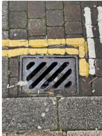
10. Blocked drainage inspection chamber
