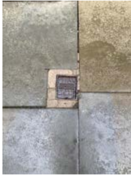
14. CATV service chamber
