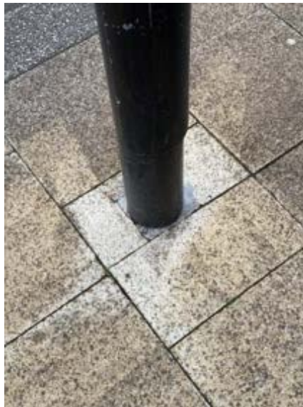
2. Cracking to tile surrounding post
