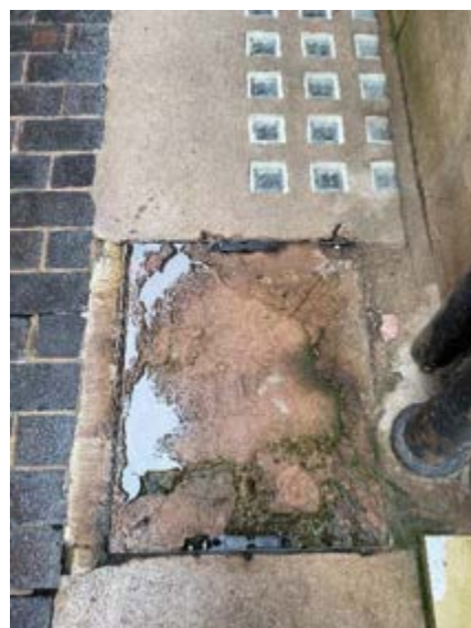
18. Damaged concrete infill with pooling
