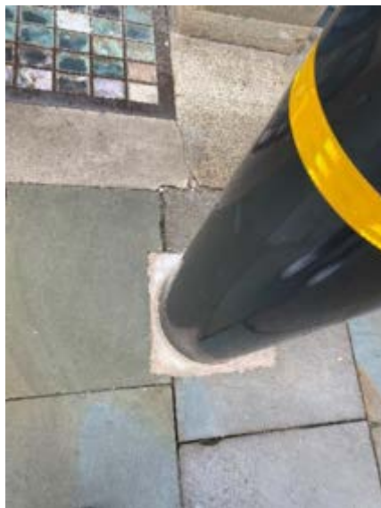
21. Condition of bollards
