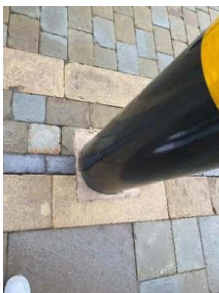
23. Condition of bollards
