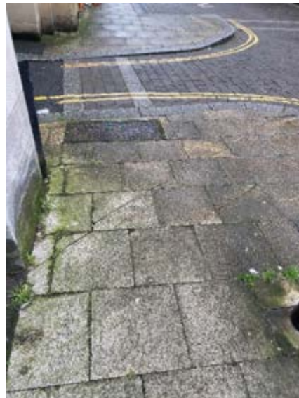
24. Some minor damage to certain tiles
