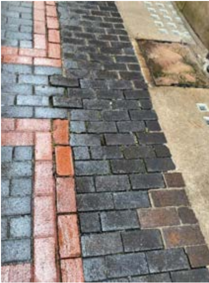
25. Loose bricks with some areas of damage
