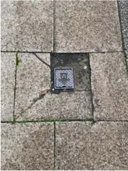
1. Water service chamber
