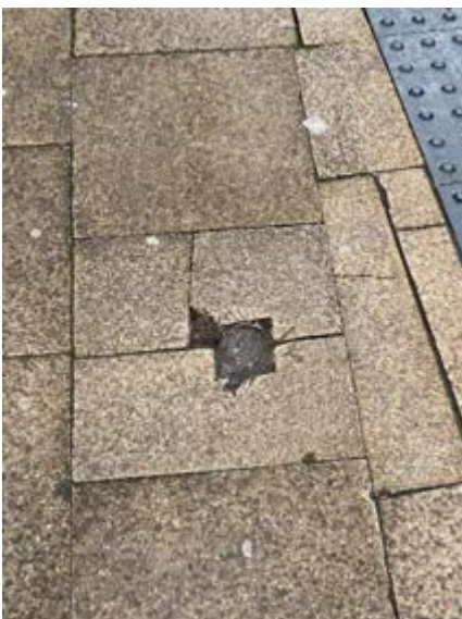
17. Damage to multiple tiles Remainder of post still between tiles
