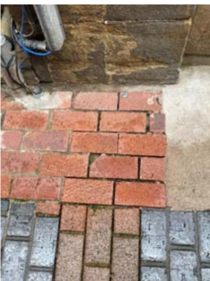
17. Chipped brick and loose mortar Exposed wires
