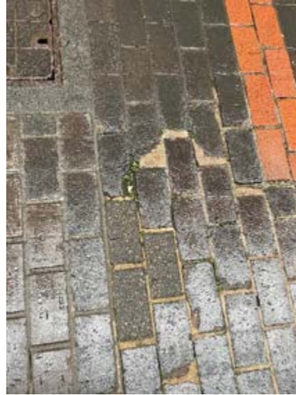
14. Damaged bricks infilled with concrete
