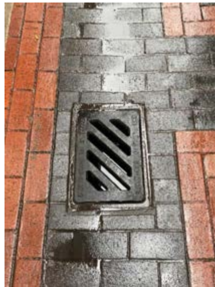
10. Blocked drainage inspection chamber
