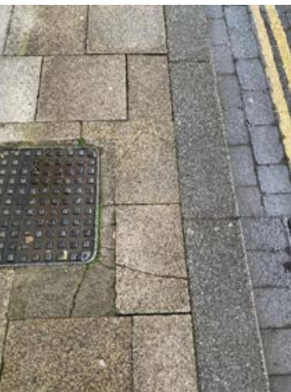
17. Multiple cracked tiles
