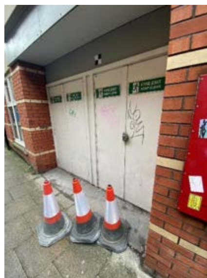
6. Graffiti damage to doors
