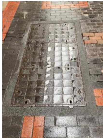
16. Three service chambers
