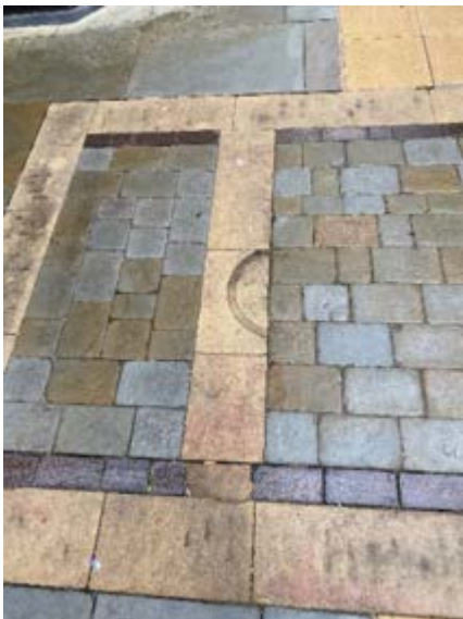
27. Overall condition of brickwork. Half moon scar in centre
