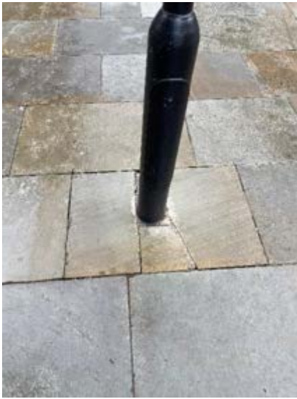
19. Cracking of tile surrounding post
