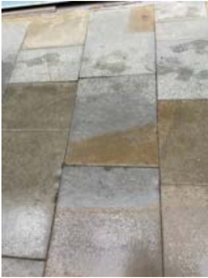
13. Damage to paving tiles
