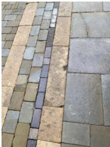
45. Cracked tile and further damage to edging tile
