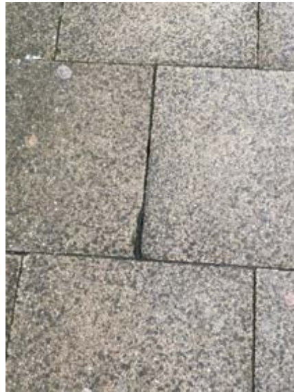
8. Small chip to paving tile
