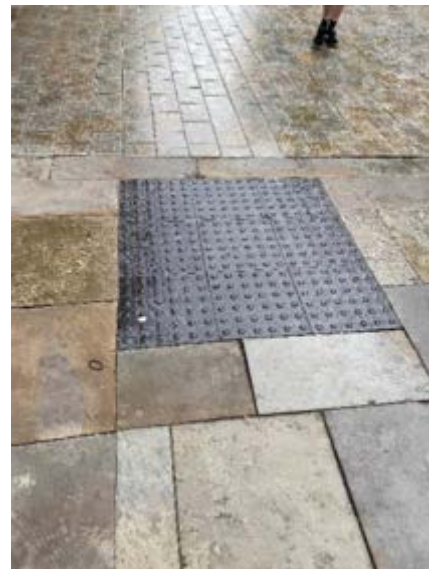
40. Condition of pedestrian crossing
