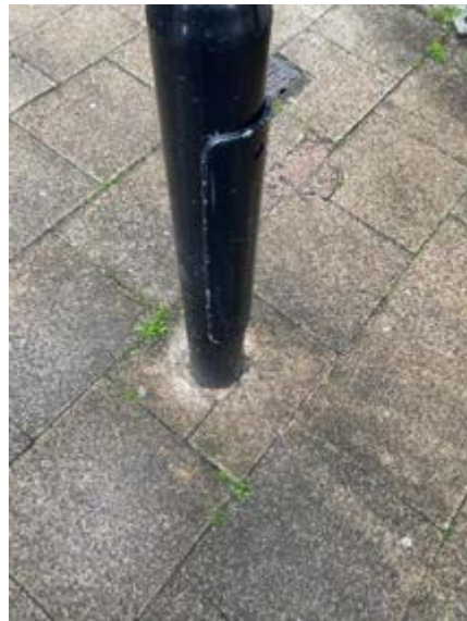
16. Cracking to tile surrounding post
