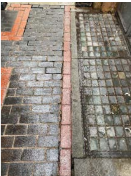
9. Missing mortar and condition of glass tiles
