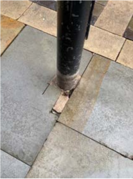
37. Cracked tile around post, issues with concrete infill
