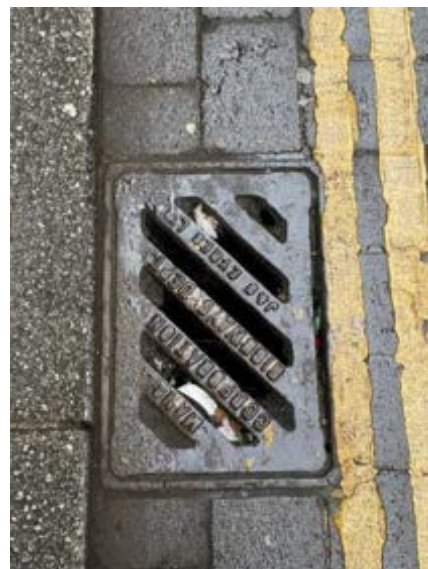
30. Blocked drainage inspection chamber
