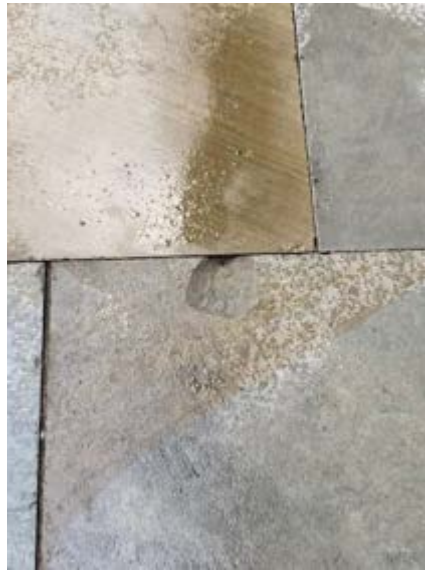
20. Significant chip in paving tile
