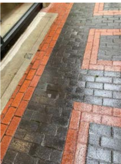
5. Pooling in sunken bricks
