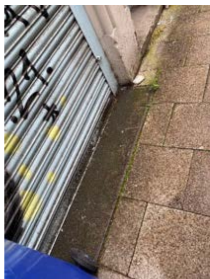
12. Condition of shutter and surrounding tiles Some chipping to tile
