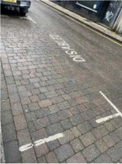
1. Disabled bay with some fading to paint
