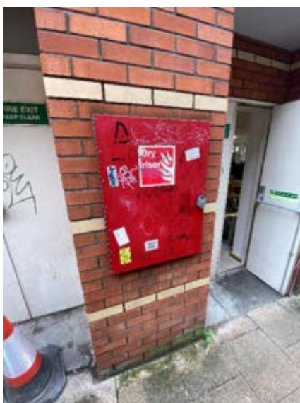
5. Graffiti damage to dry riser
