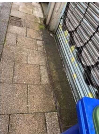
11. Condition of shutter & surrounding tiles
