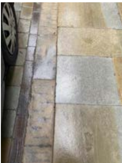
29. Pooling within edge paving damage & damage to edge stones
