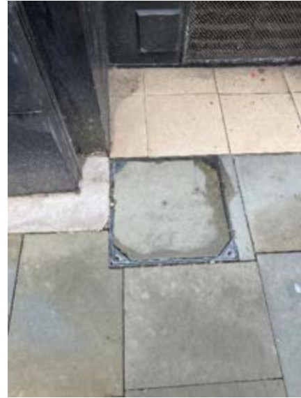
2. Service chamber to the side of the
