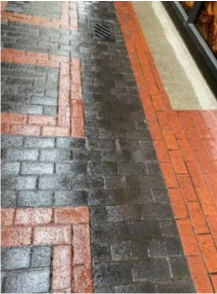
1. Significant pooling along sunken bricks
