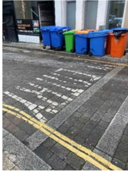
14. Faded no entry paint
