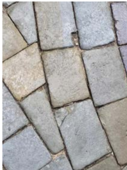
46. Damage to some bricks
