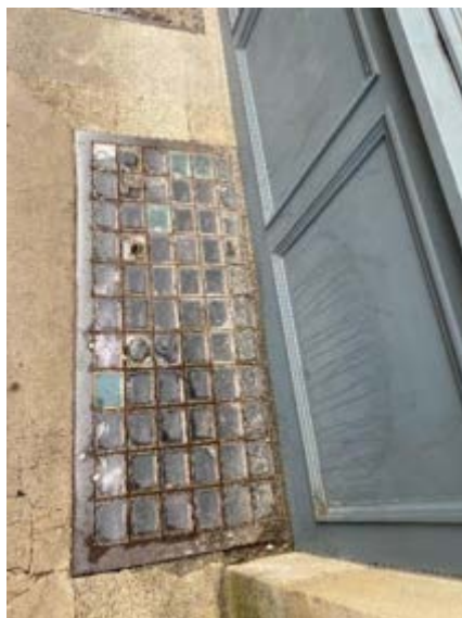
33. Glass tiles – some damage to certain tiles
