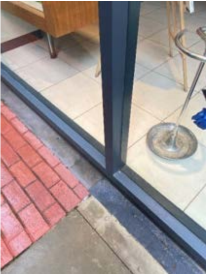
9. Tarmac infill to concrete at edge of window
