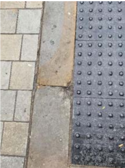
39. Corners of tiles chipped
