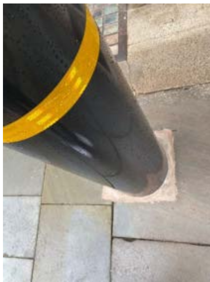
22. Condition of bollards
