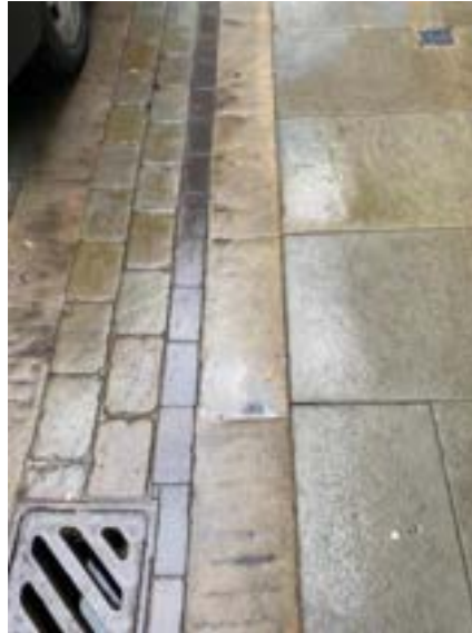
28. Scarring to edge paving.
