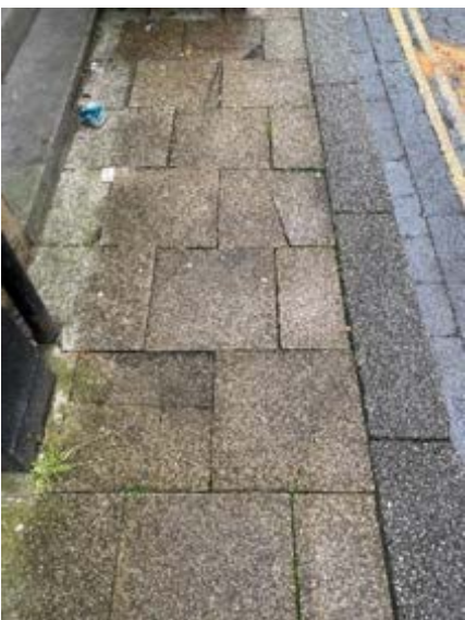
29. Multiple cracked tiles
