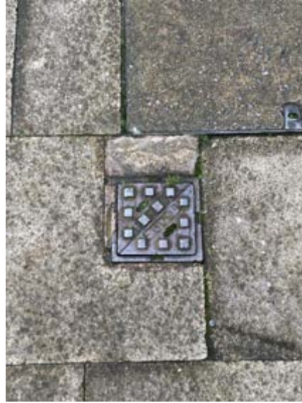
26. Gas service chamber
