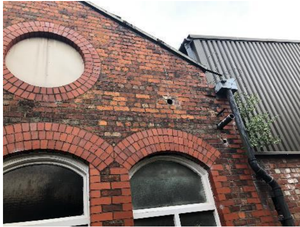
PLATE 4 SHOWING HOLES PRESENT ALONG NORTH-WESTERN ASPECT
