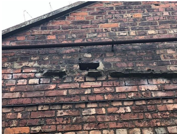
PLATE 5 SHOWING MISSING BRICKS ALONG NORTH-WESTERN ASPECT
