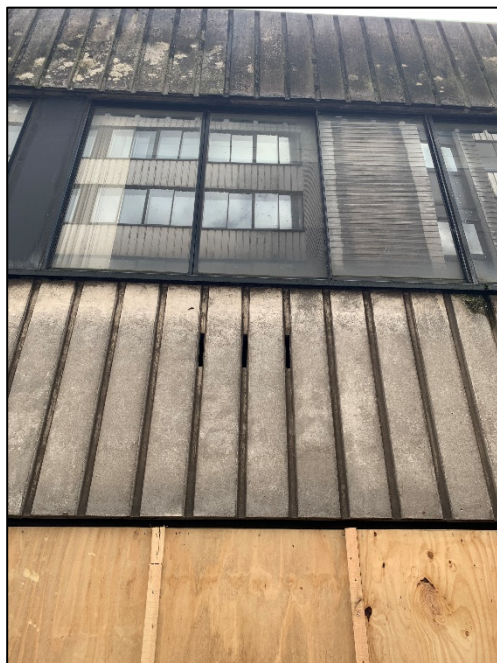
Photo 6 Gaps within concrete present on Premier House
