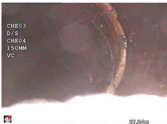
11, 00:04:56, 27.04 m Fracture, circumferential at joint from 2 o'clock to 5 o'clock, POSS PATCH REQ
