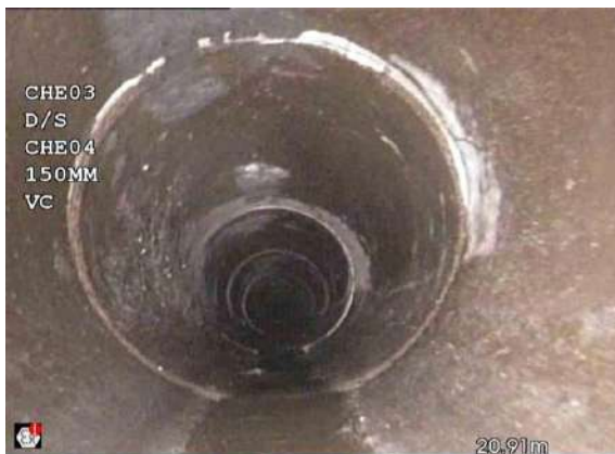
7, 00:04:02, 20.91 m Fracture, circumferential at joint from 2 o'clock to 5 o'clock, POSS PATCH REQ
