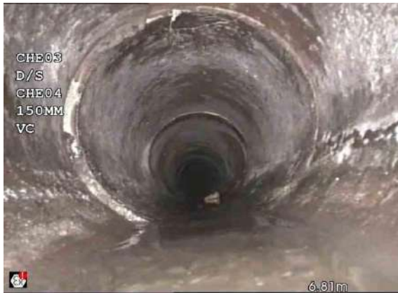
5, 00:02:00, 6.81 m Fracture, circumferential at joint from 12 o'clock to 1 o'clock, POSS PATCH REQ
