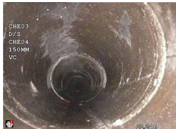
8, 00:04:15, 22.24 m Fracture, circumferential at joint from 2 o'clock to 9 o'clock, POSS PATCH REQ
