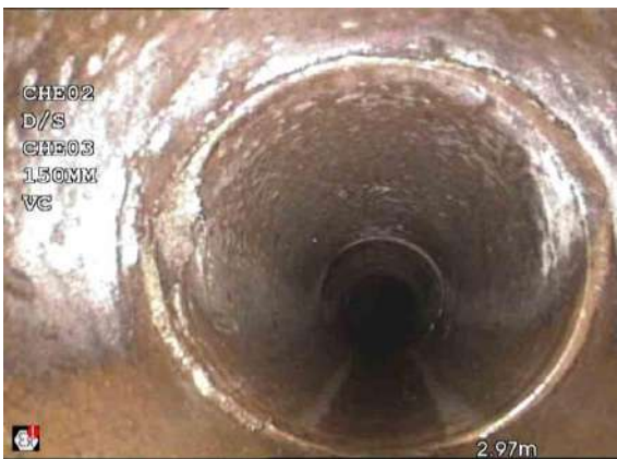
CHE02 D/S CHE03 150MM VC 2.97m Broken pipe at joint from 8 o'clock to 9 o'clock, POSS PATCH REQ
