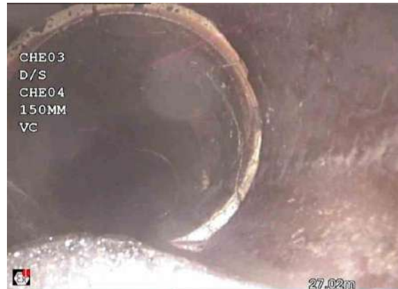
10, 00:05:04, 27.02 m Fracture, circumferential at joint from 7 o'clock to 9 o'clock, POSS PATCH REQ
