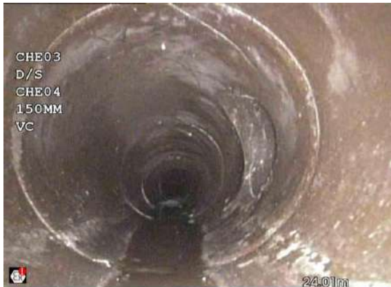
9, 00:04:29, 24.01 m Fracture, circumferential at joint from 12 o'clock to 2 o'clock, POSS PATCH REQ
