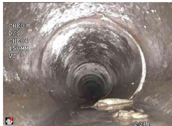
4, 00:00:57, 2.34 m Settled deposits, other, 10% cross-sectional area loss, FOUL AND RAGS
