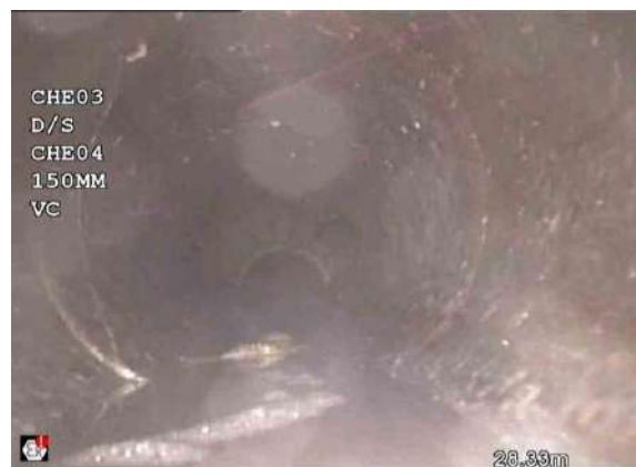
12, 00:05:20, 28.33 m Fracture, circumferential at joint from 7 o'clock to 10 o'clock, POSS PATCH REQ
