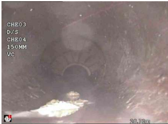
13, 00:05:29, 28.73 m Settled deposits, other, 10% cross-sectional area loss, FOUL
