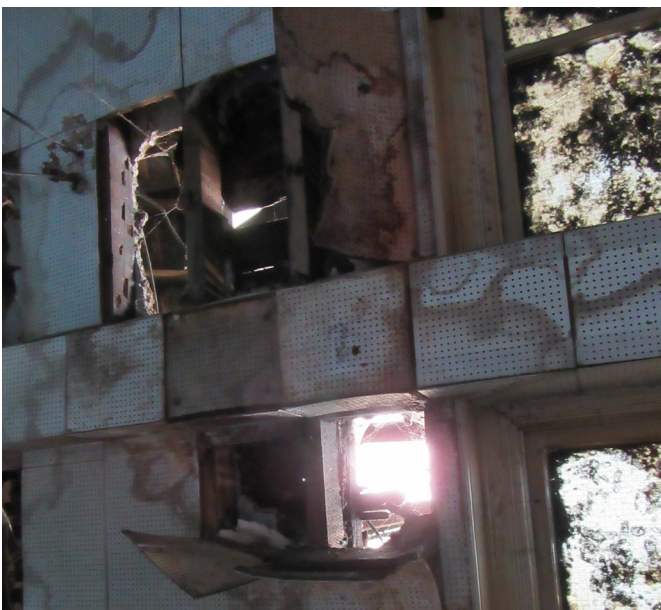
Image 16: Showing damaged and non-original ceiling with lath and plaster missing. Taken in 2018.
