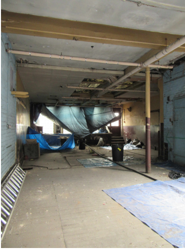
Image 17: Showing extent of non-original ceiling tiles to far end of space.
