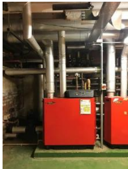
Figure 27: Current modern boilers installed post 1960.
