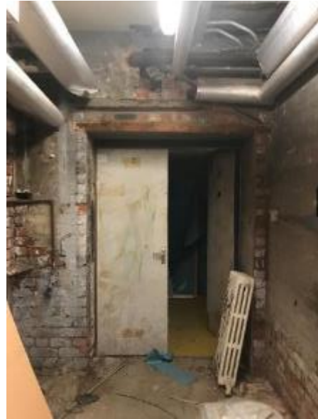
Figure 25: A non-original timber ply door to the basement.
