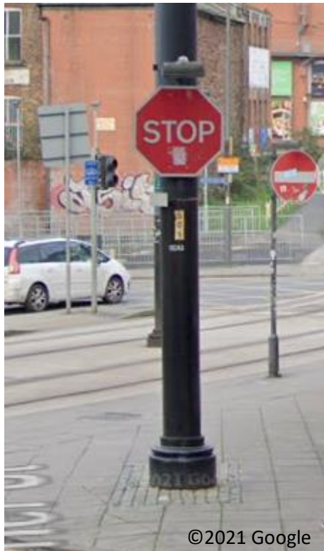
Figure 11 Illuminated stop sign Pole CC53
