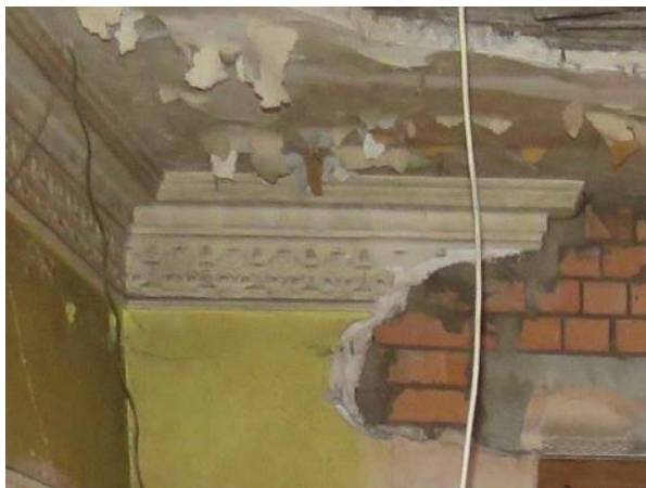
Figure 68: A closer view of the remaining piece of highly decorated plaster cornice return in Room F16. (Source: SLHA 2017)
