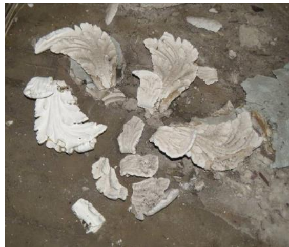
Figure 57: The current condition of the ceiling rose, which has fallen due to water ingress since 2007 and is now stored within the room. (Source: SLHA 2017)
