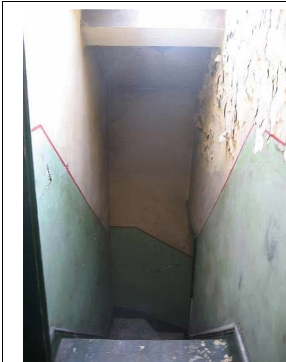
Figure 96: The eastern dwelling attic staircase from Room F26. (Source: SLHA 2007 - please note the condition of the building has significantly worsened since 2007)
