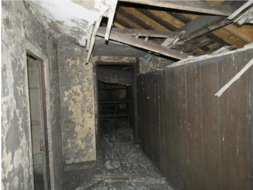
Figure 83: Room A15 (looking east) – The attic corridor is shown here looking east, and illustrates the original/early boarded partition to the right. (Source: SLHA 2020 - please note the condition of the building has significantly worsened since 2020)
