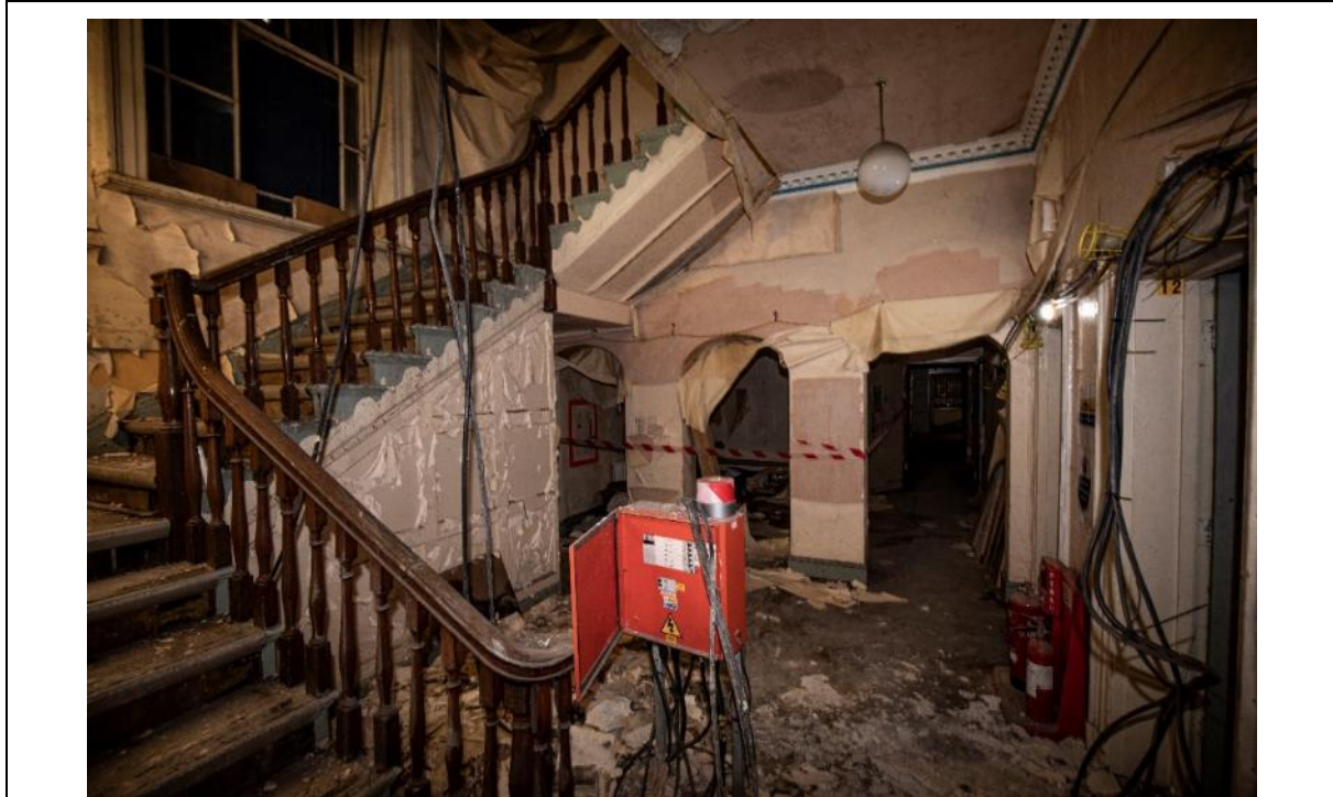
Figure 61a: The staircase and staircase hall as seen presently, showing its worsened general condition (Source: Watch This Space (Jembrana) Ltd 2022)
