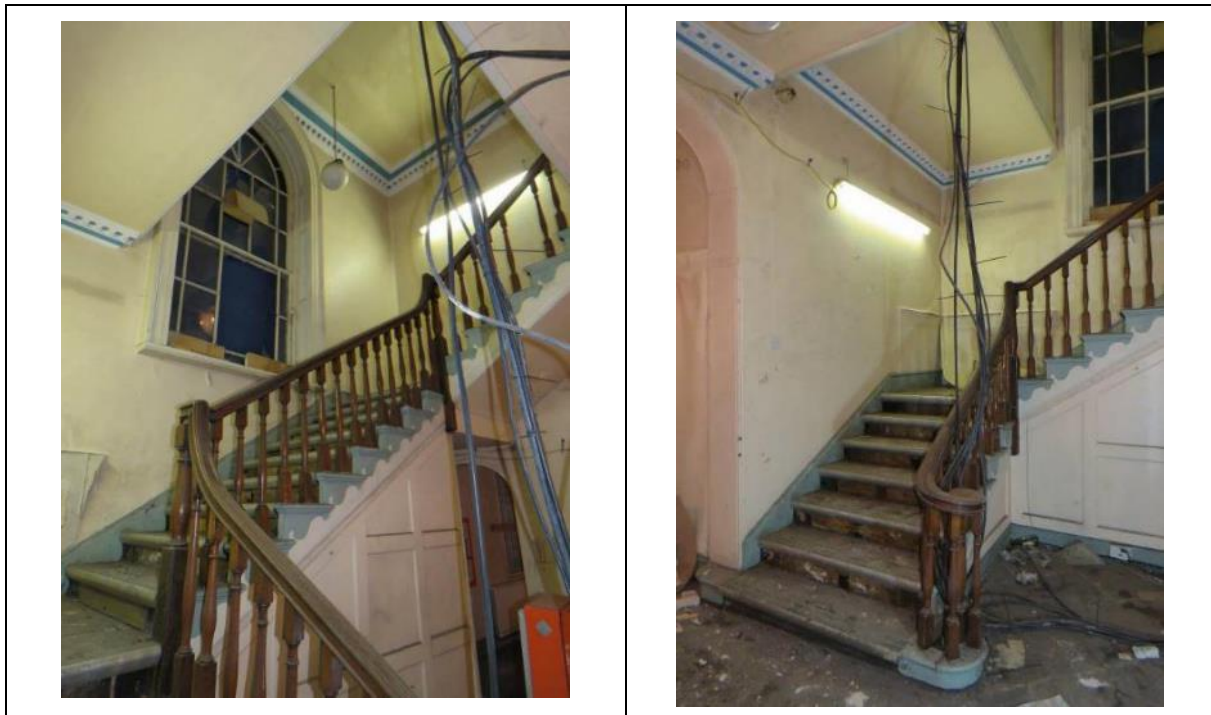
Figure 60 & 61: Room G02 (looking southwards) – The original staircase to the eastern dwelling, showing the believed to be c19 th century hardwood balustrades. (Source: SLHA 2017 - please note the condition of the building has significantly worsened since 2007)
