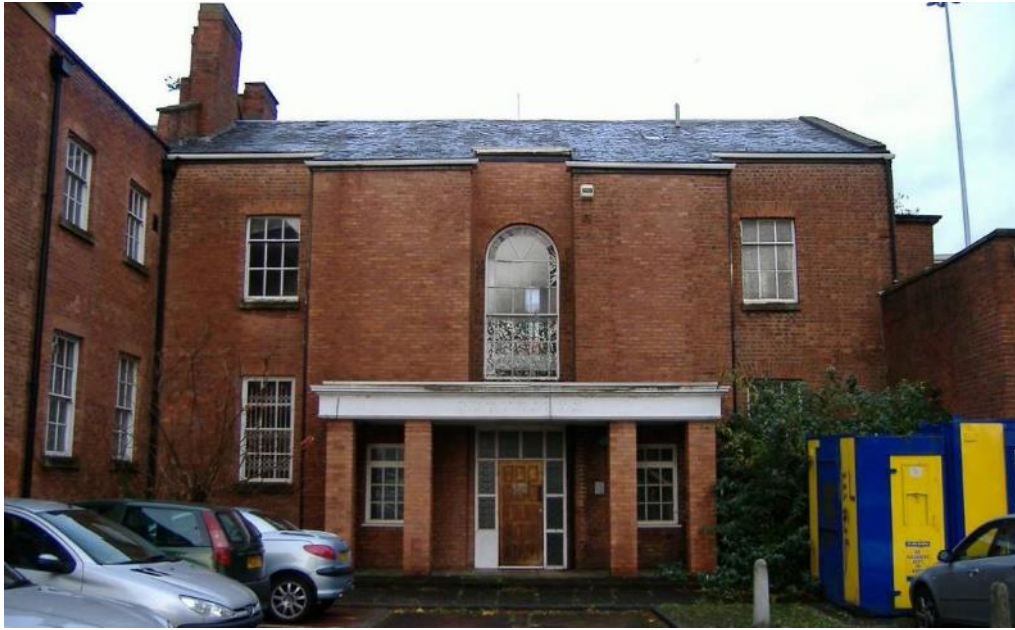
Figure 38: The south (rear) elevation of the eastern dwelling as seen in 2007, showing the alterations undertaken in 1977. (Source: SLHA 2007 – Note the current condition of the building has since worsened)
