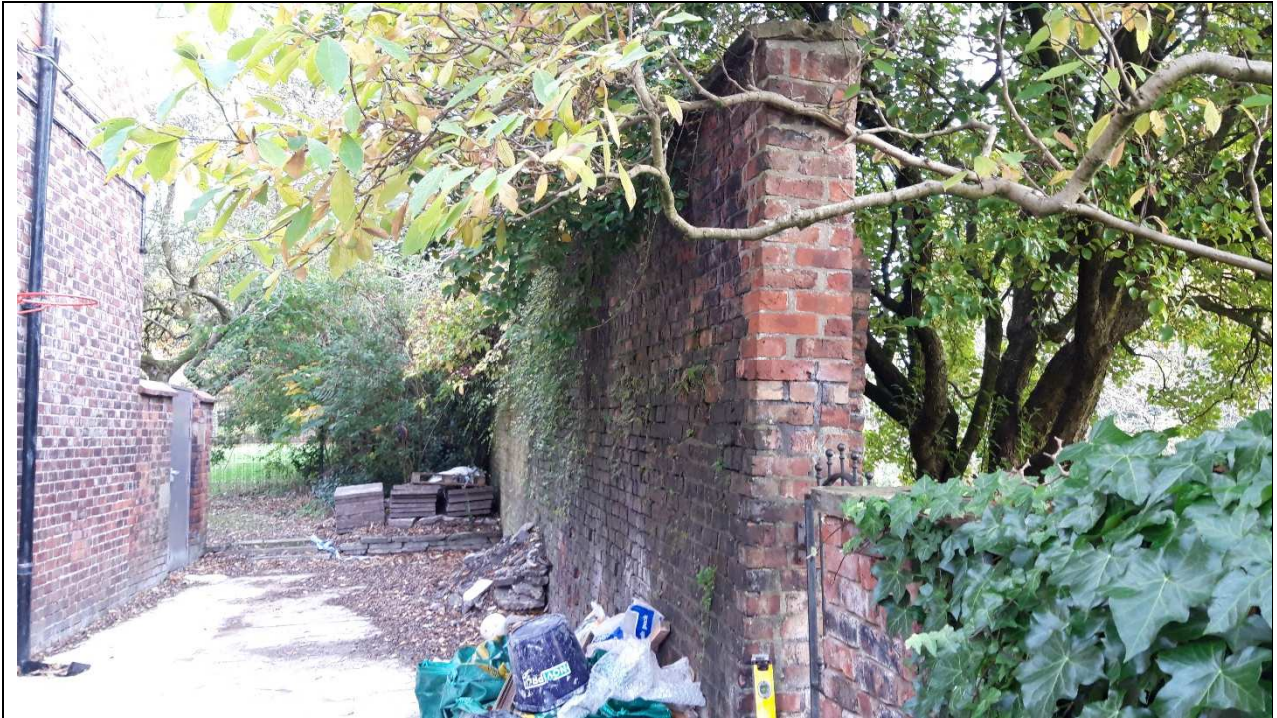
Leaning Garden Wall to Left of Property
