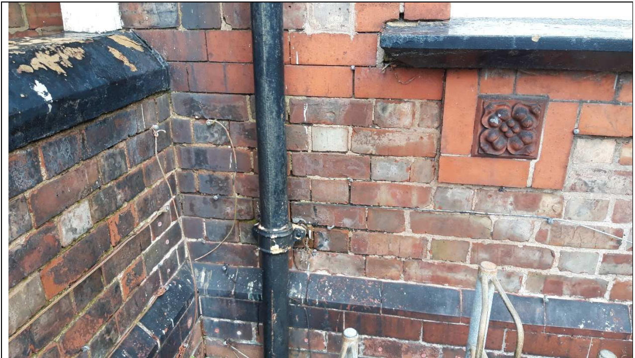
Staining & Perishing Joints to Front Wall Around Down-Pipe
