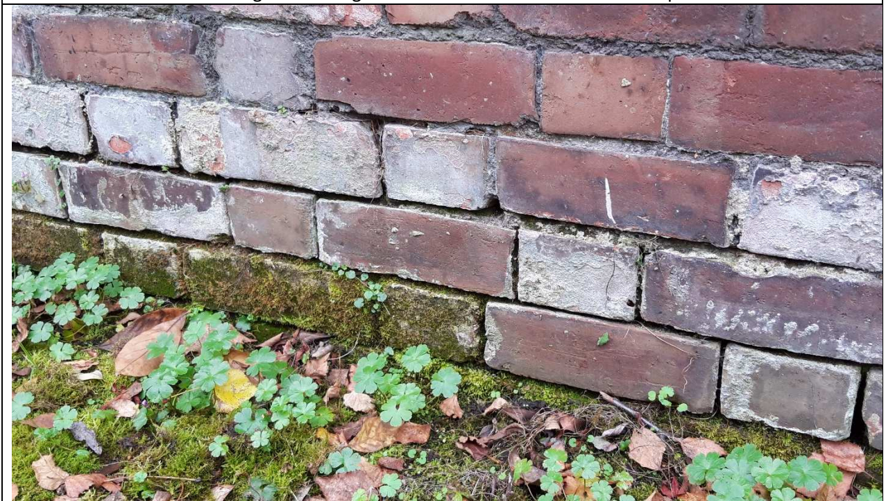
Eroded Mortar Joints to Left Gable Wall Base
