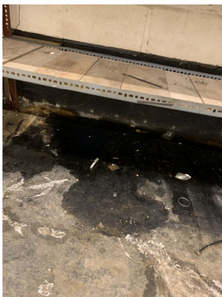
Photograph 3: Evidence of staining on the concrete floor in the north east section of the existing building.
