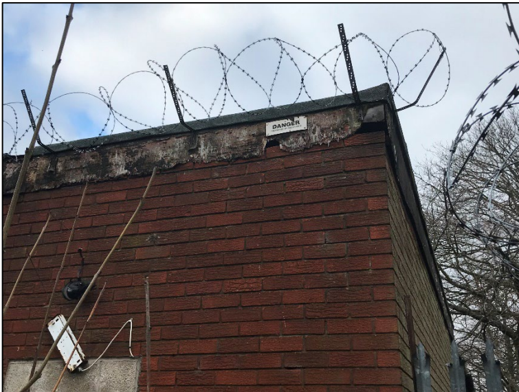
Photograph 4.5 Holes in wooden barge boards
