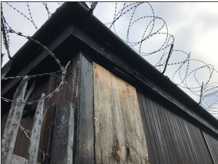
Photograph 4.6 Hole into wooden soffit box
