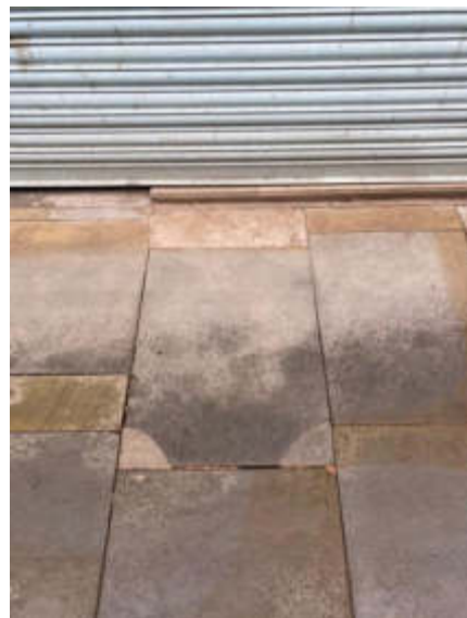
6. Cracked corners of paving stone
