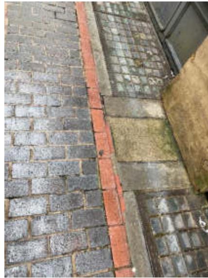
8. Loose bricks and damaged concrete infill
