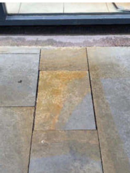
11. Loose paving stone
