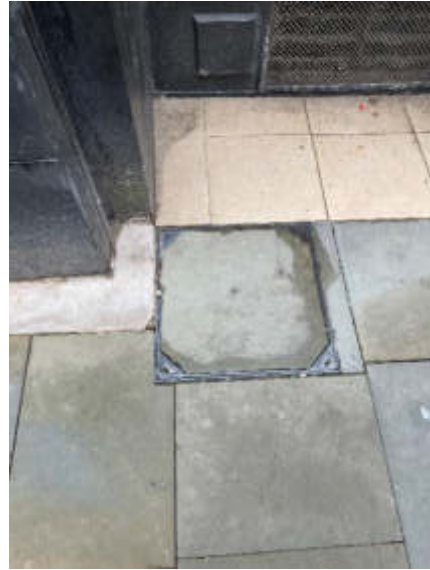
2. Service chamber to the side of the
