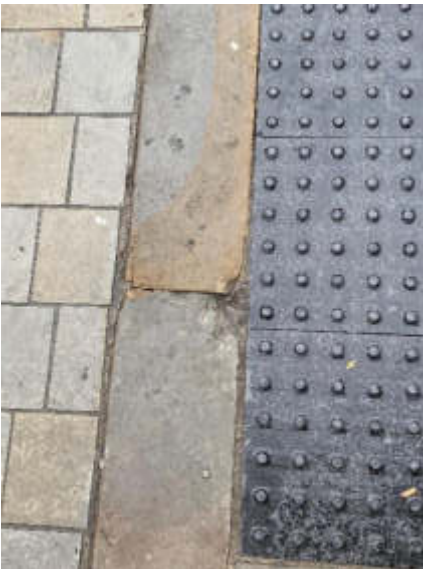
39. Corners of tiles chipped
