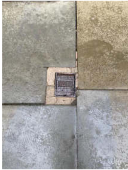
14. CATV service chamber
