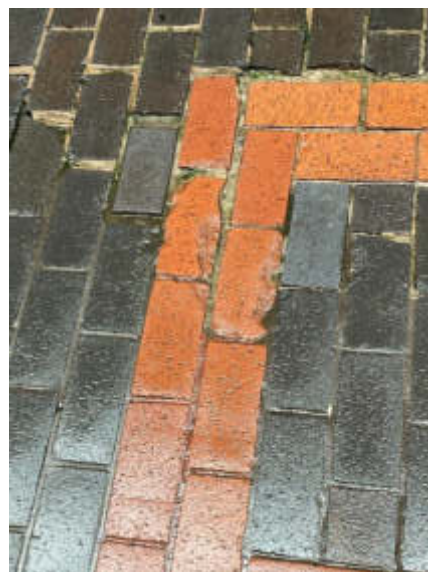
12. Significant damage to feature bricks
