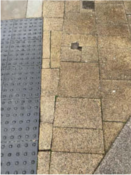
19. Cracked paving tiles
