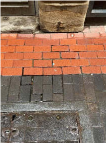
13. Missing mortar – loose bricks
