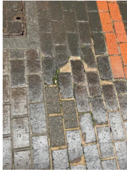
14. Damaged bricks infilled with concrete
