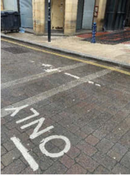
13. Arrow paint significantly faded
