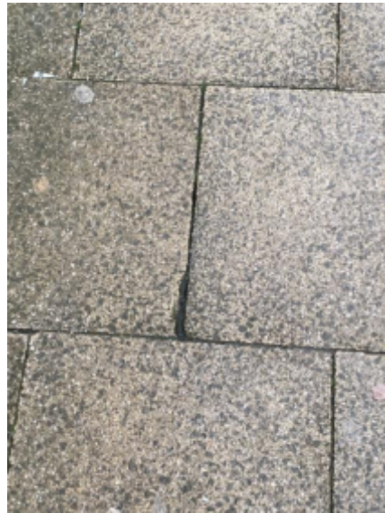
8. Small chip to paving tile
