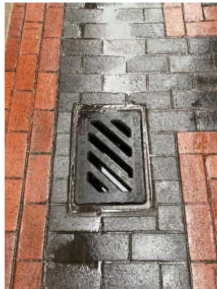
10. Blocked drainage inspection chamber
