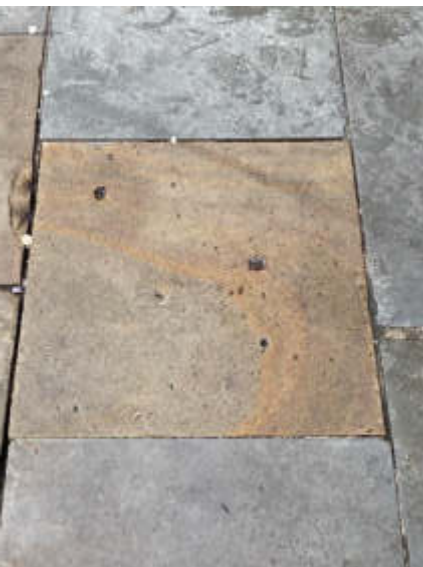
41. Two chips / damage to tile
