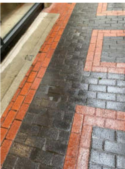
5. Pooling in sunken bricks
