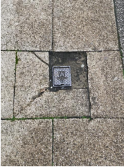
1. Water service chamber
