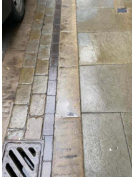
28. Scarring to edge paving.
