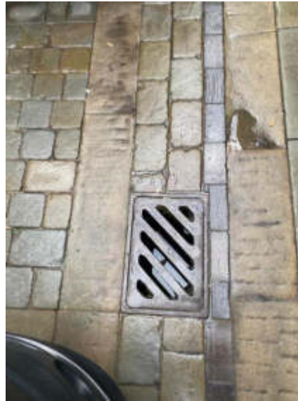
30. Blocked drainage inspection chamber
