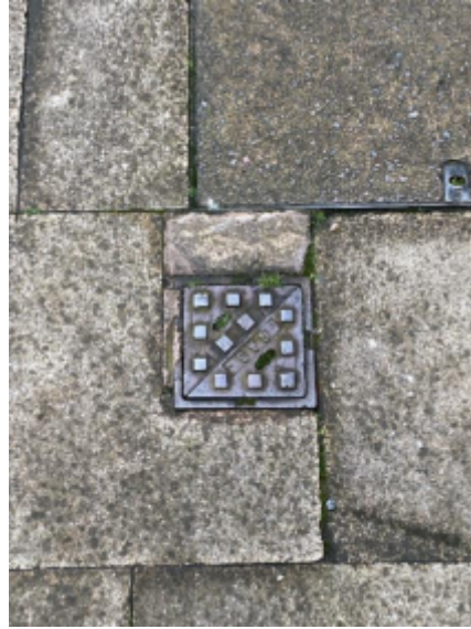
26. Gas service chamber
