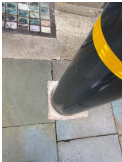
21. Condition of bollards
