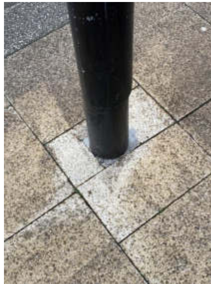
2. Cracking to tile surrounding post
