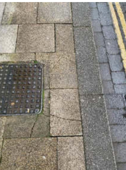
17. Multiple cracked tiles
