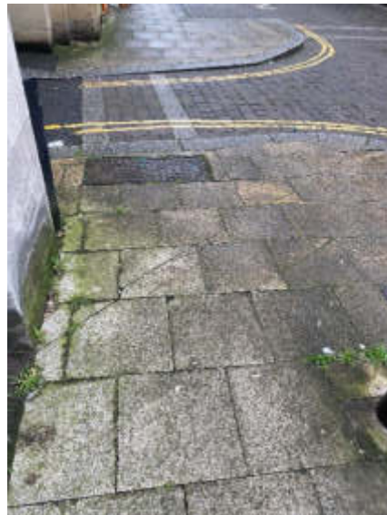
24. Some minor damage to certain tiles
