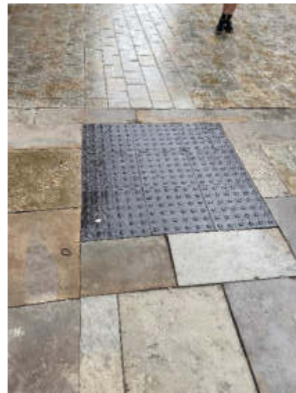
40. Condition of pedestrian crossing
