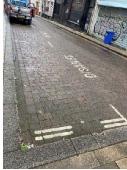
2. Disabled bay with some fading to paint
