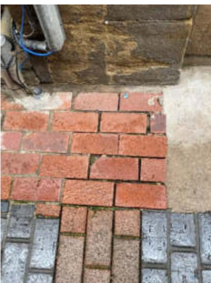
17. Chipped brick and loose mortar Exposed wires
