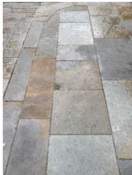
42. Corner damage to tile
