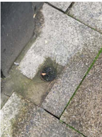
23. Evidence of removed post – scarring around
