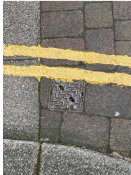
14. Water service chamber
