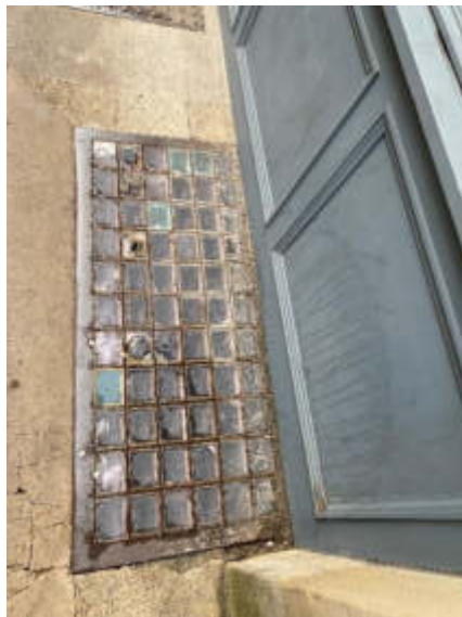
33. Glass tiles – some damage to certain tiles
