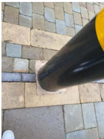
23. Condition of bollards
