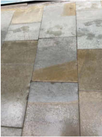
13. Damage to paving tiles
