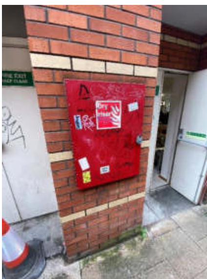
5. Graffiti damage to dry riser
