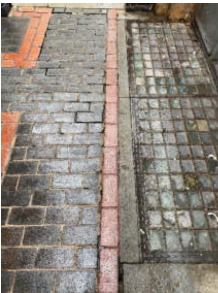
9. Missing mortar and condition of glass tiles
