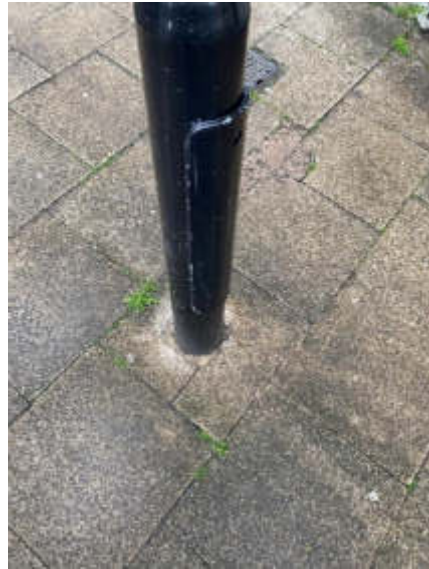
16. Cracking to tile surrounding post
