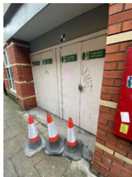
6. Graffiti damage to doors
