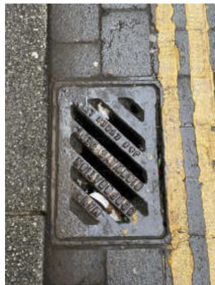
30. Blocked drainage inspection chamber
