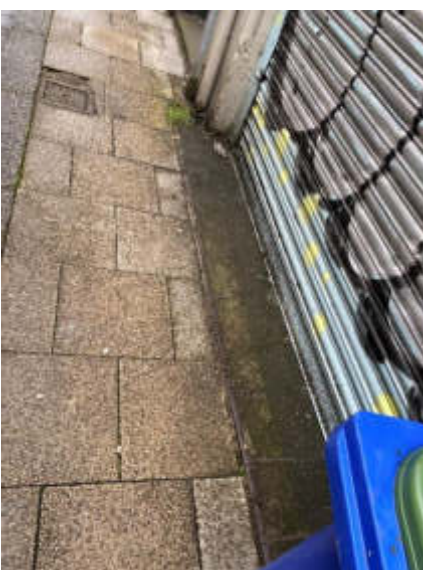
11. Condition of shutter & surrounding tiles
