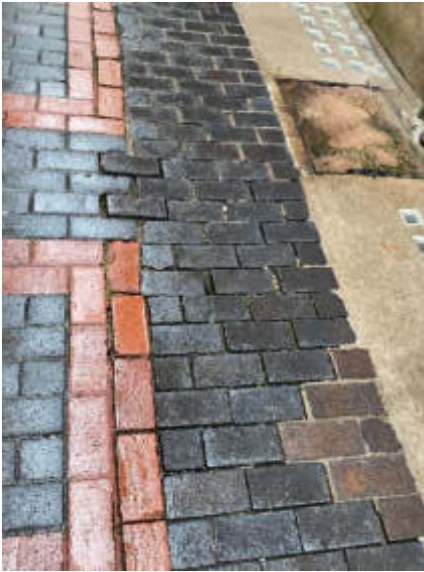
25. Loose bricks with some areas of damage
