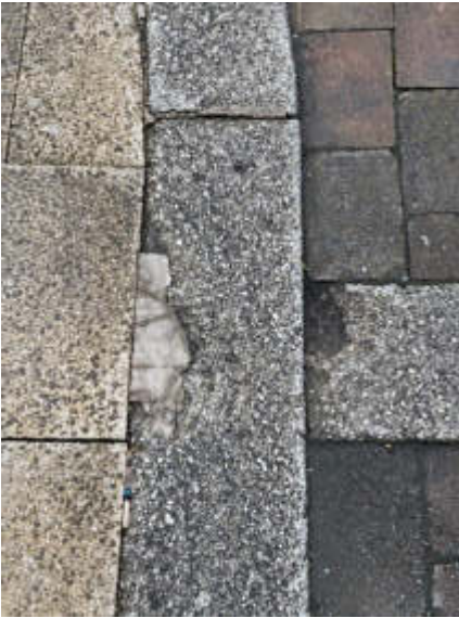
13. Damage to brick in road and concrete infill to damage edge
