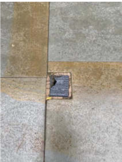
17. Cracked service chamber
