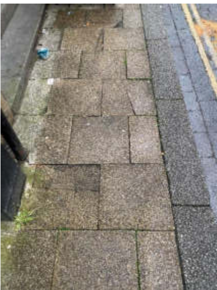
29. Multiple cracked tiles
