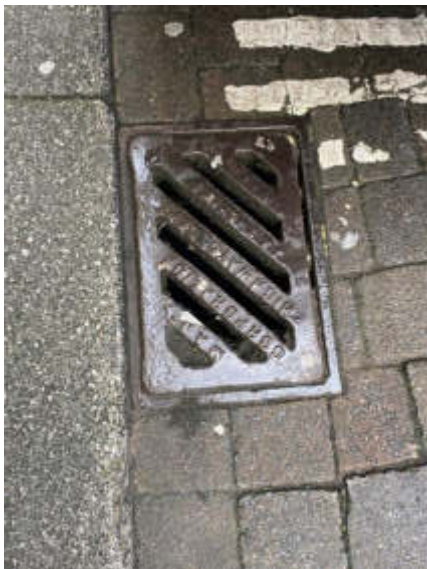
15. Partially blocked (corner) inspection chamber
