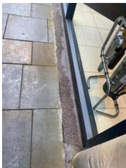
12. Wearing of tarmac infill between store front and paving
