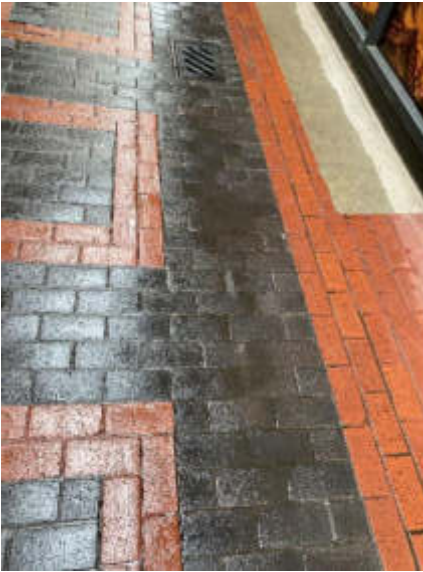
1. Significant pooling along sunken bricks
