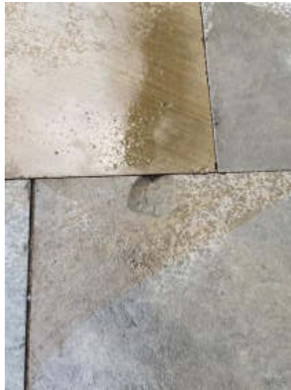
20. Significant chip in paving tile
