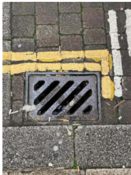
10. Blocked drainage inspection chamber
