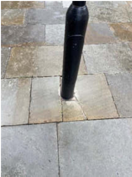
19. Cracking of tile surrounding post
