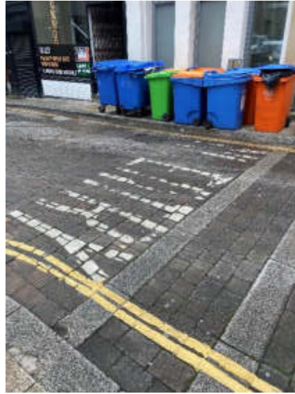
14. Faded no entry paint
