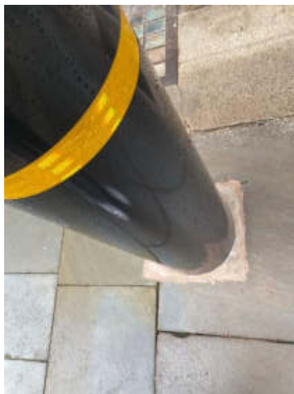
22. Condition of bollards
