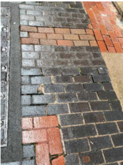
15. Some loose bricks and additional section of feature bricks
