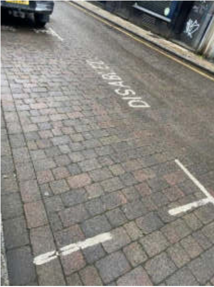
1. Disabled bay with some fading to paint
