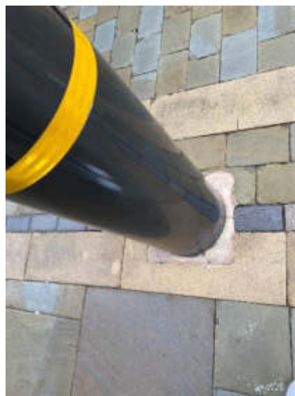
24. Condition of bollards
