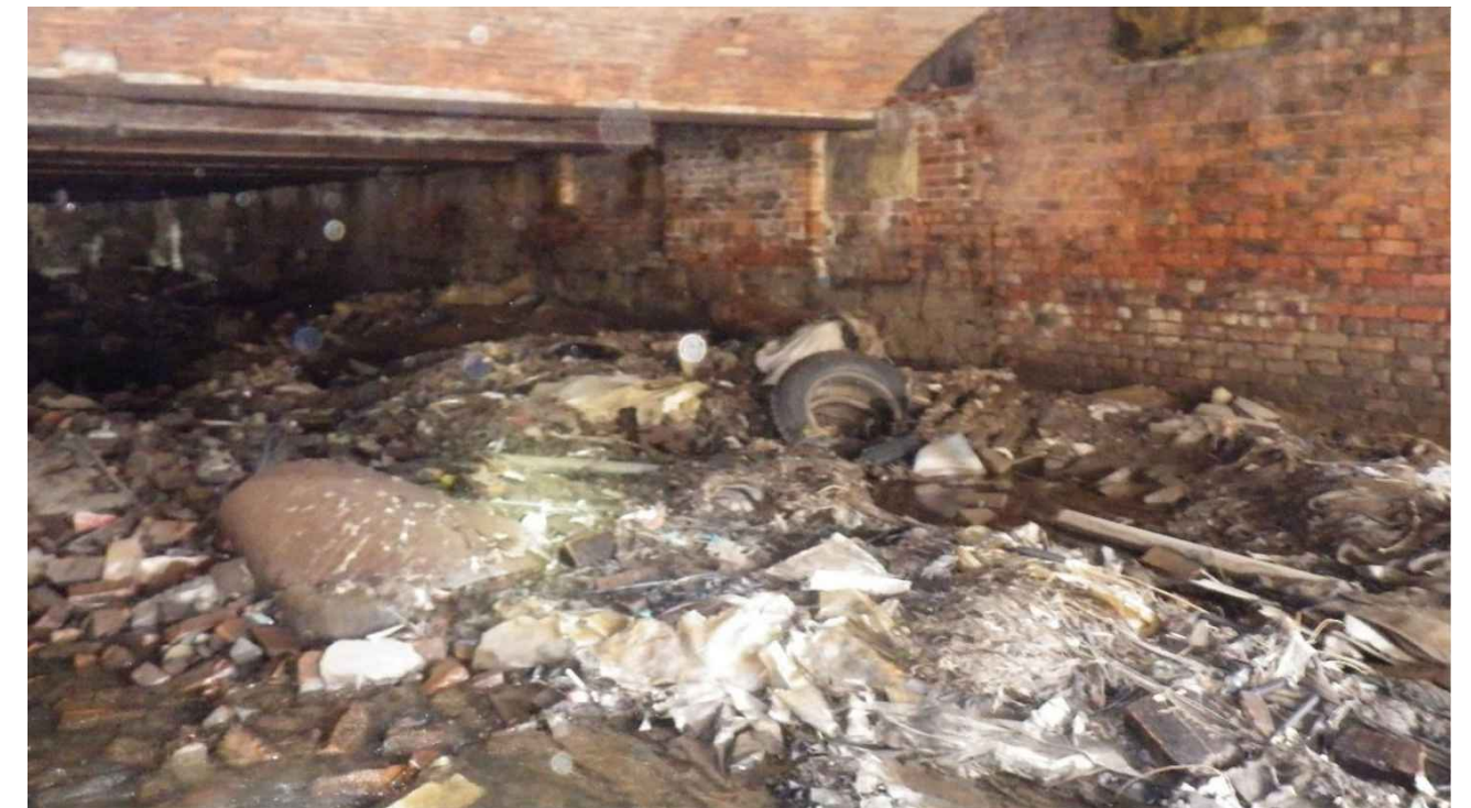
Figure 5-3 Debris build up within culvert
