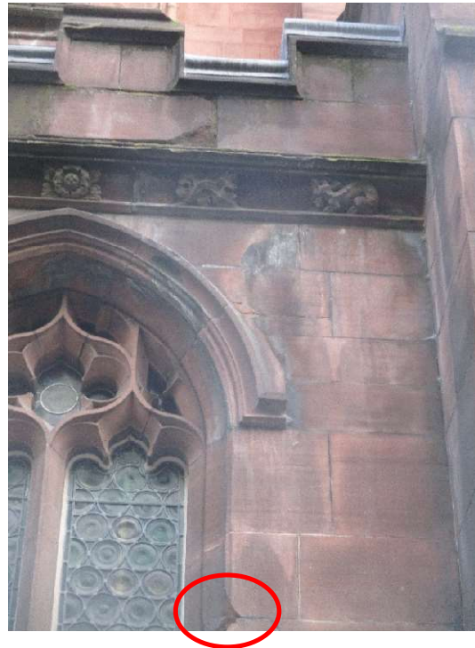
Stonework damage to window GW52(S) on Spinningfields (south) elevation
