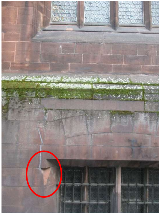
Stonework damage to window BW49(S) on Spinningfields (south) elevation
