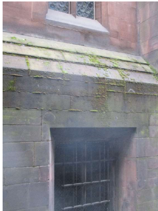
Example of moss and algae growth and open joints on Wood Street (north) elevation
