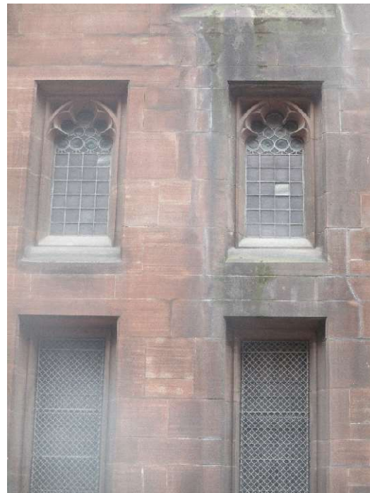
Example of moss and algae growth on Wood Street (north) elevation
