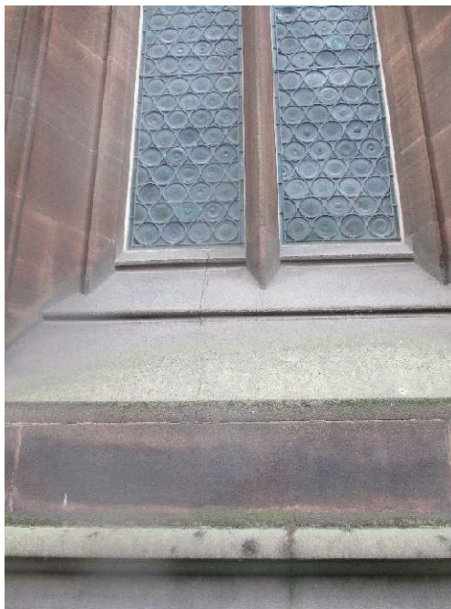
Example of moss and algae growth to window sill and string course on Deansgate (east) elevation
