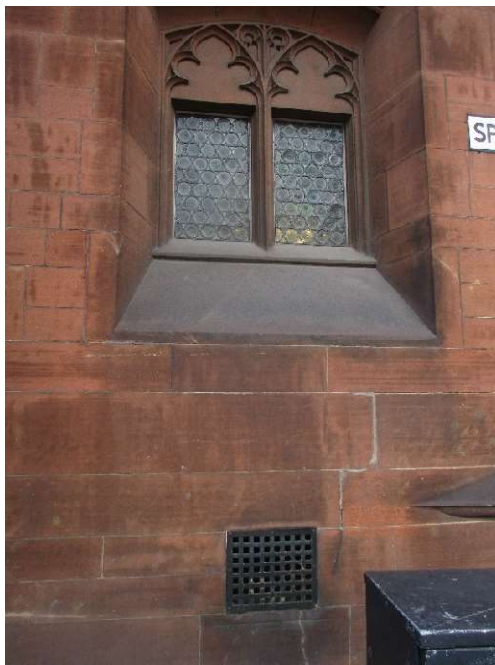
Example of unsympathetic previous mortar repair to cracking on Spinningfields (south) elevation
