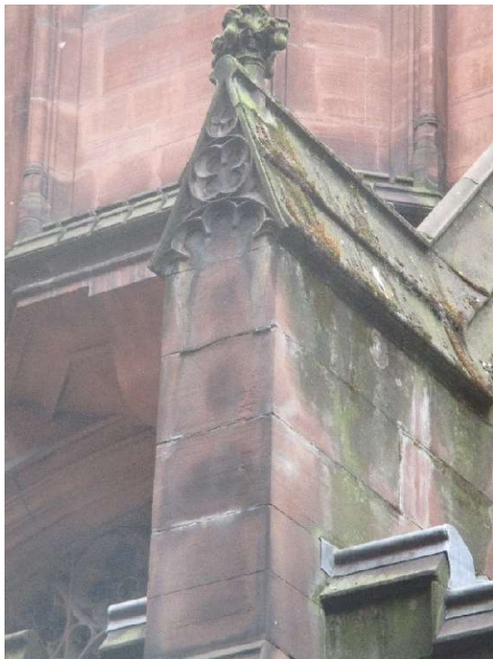
Example of moss and algae to buttress on Wood Street (north) elevation
