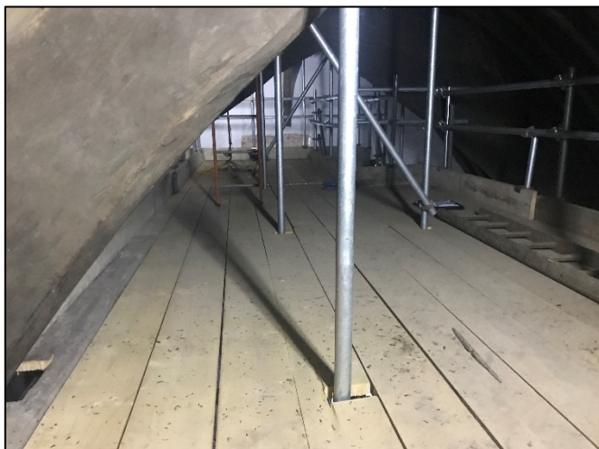
Figure 4: Bat droppings on scaffold boards.
