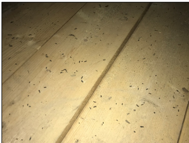
Figure 5: Close up of bat droppings on scaffold boards.
