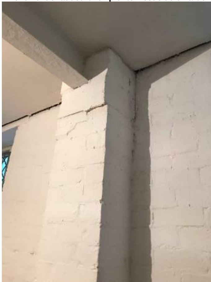
Photograph 59A: Lateral displacement between wall and pier, as well as enlargement of gap between ceiling finish and wall
