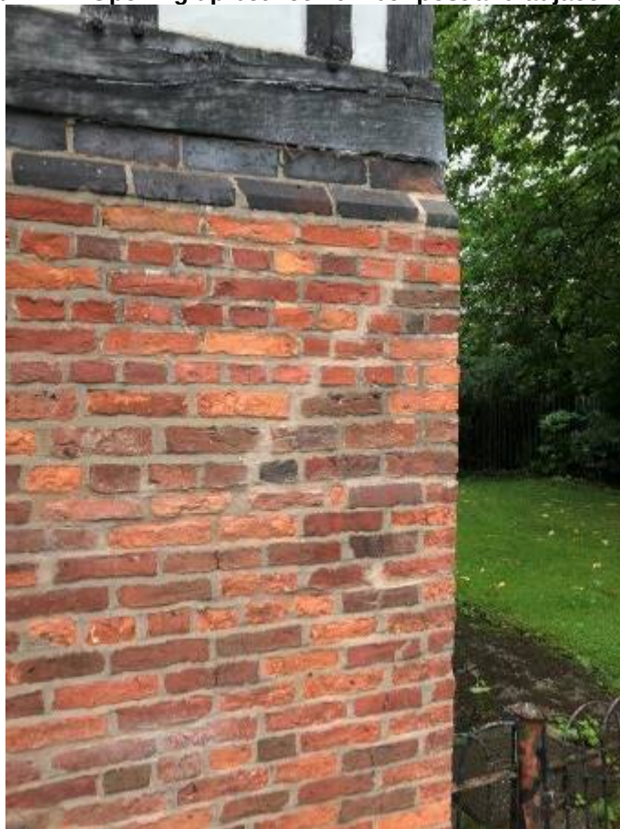
Photograph 41B: Repointed stepped cracking to south west corner with cement. A number of horizontal repointed lengths around corner (perhaps HeliBar). Satisfactory condition.
