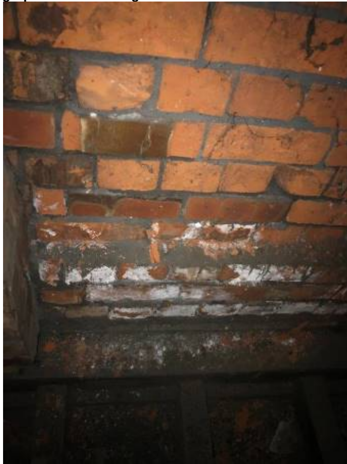
Photograph 9B: Salt staining and debris collection
