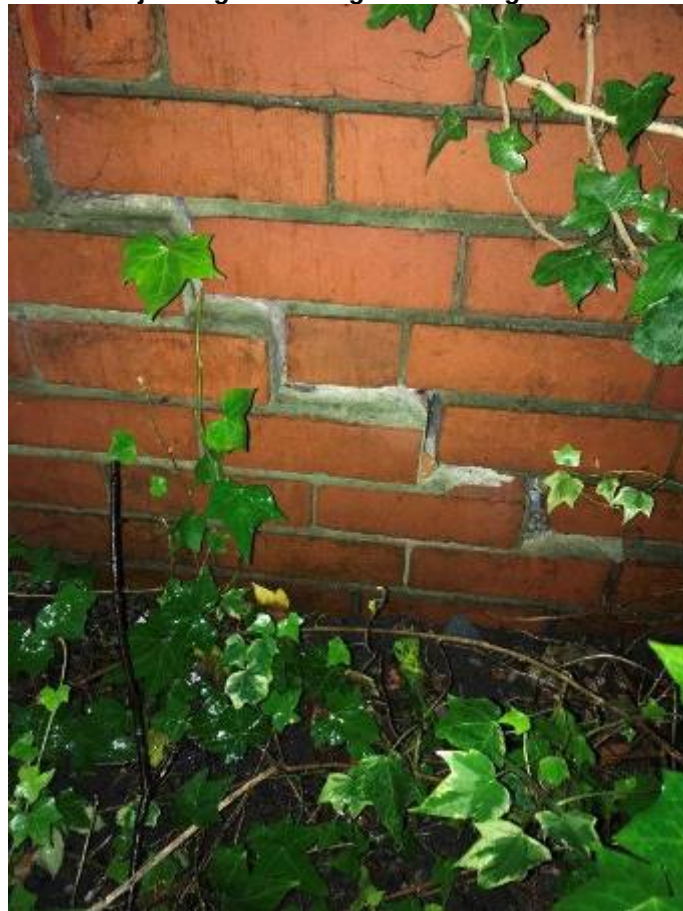
Photograph 69B: Stepped cracking to north west corner of building to flat roofed element
