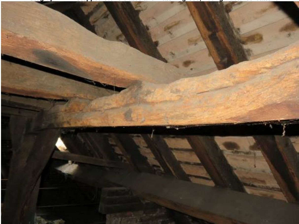
Photograph 12: Collar purlin with sapwood decay
