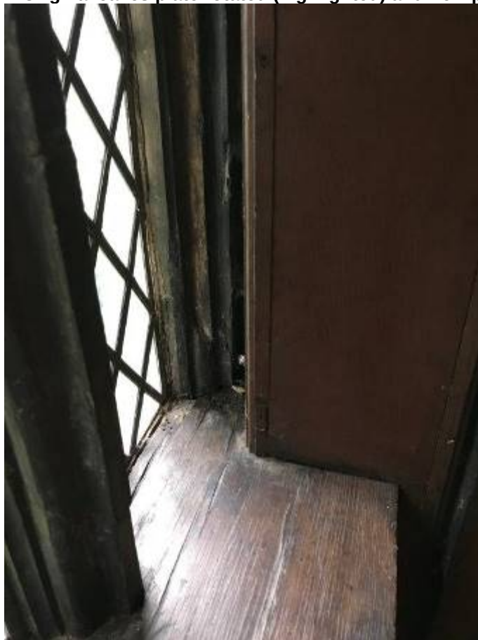
Photograph 22A: Water ingress and damage to south side of mullion window
