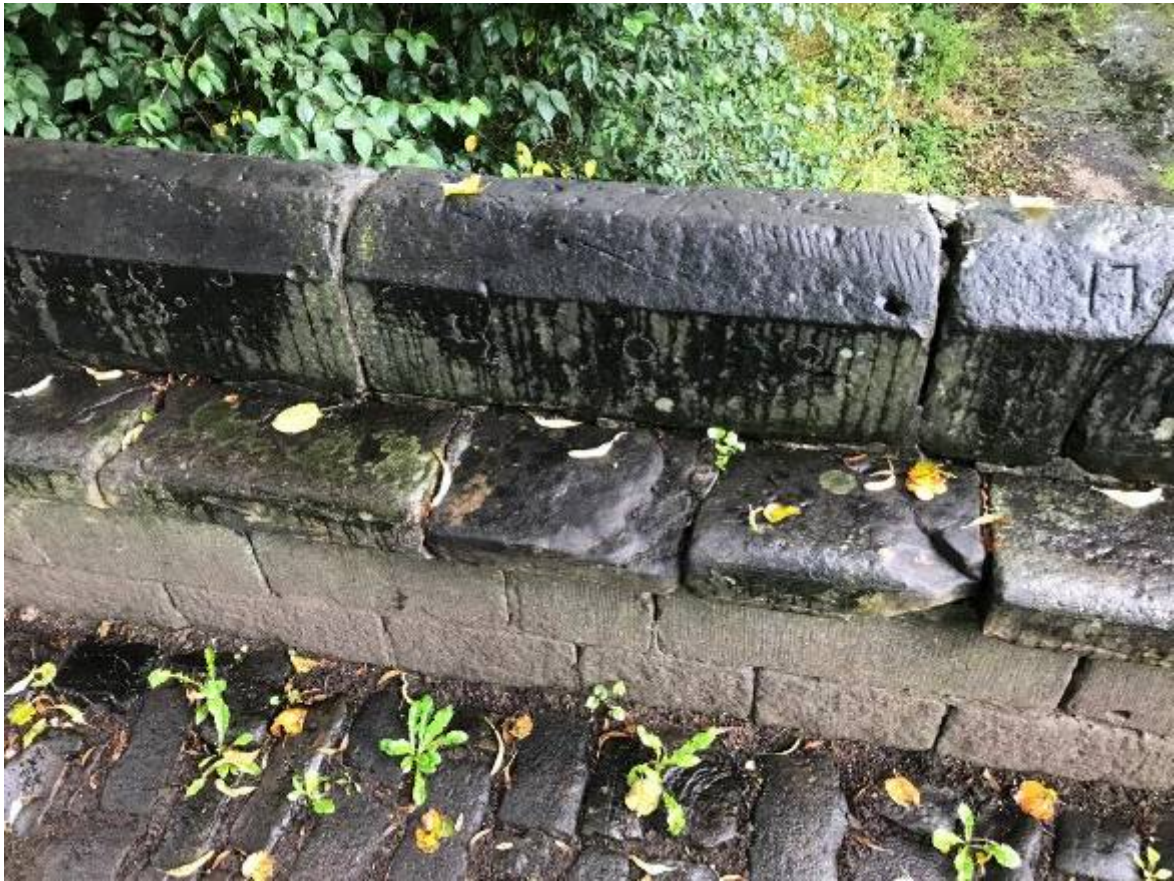
Photograph 70B: Open jointed nature of coping stone joints to east continuing through into parapet
