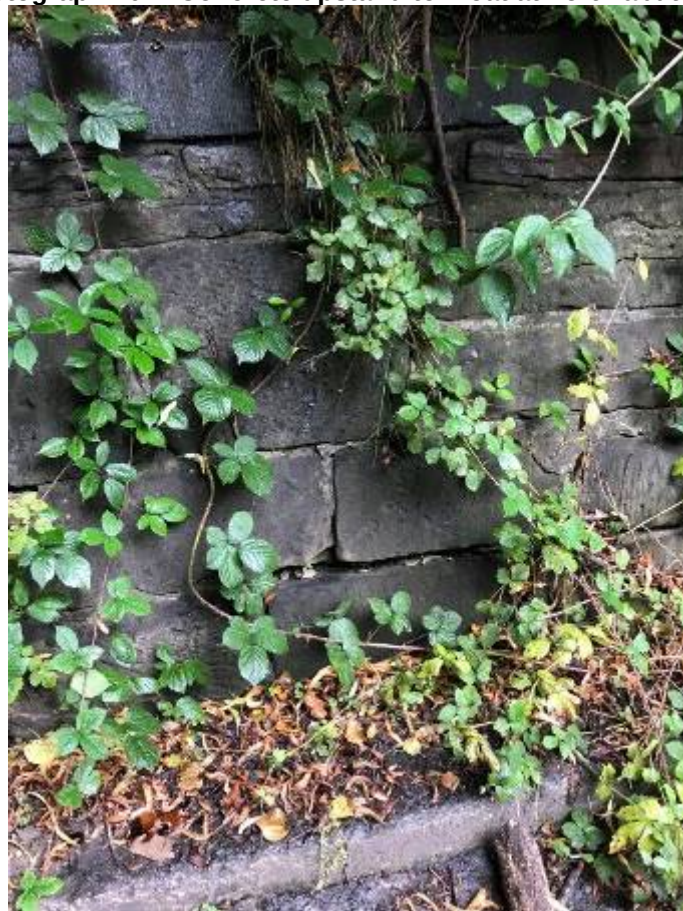
Photograph 70I: Retaining wall to north abutment exhibiting deterioration through mortar joints
