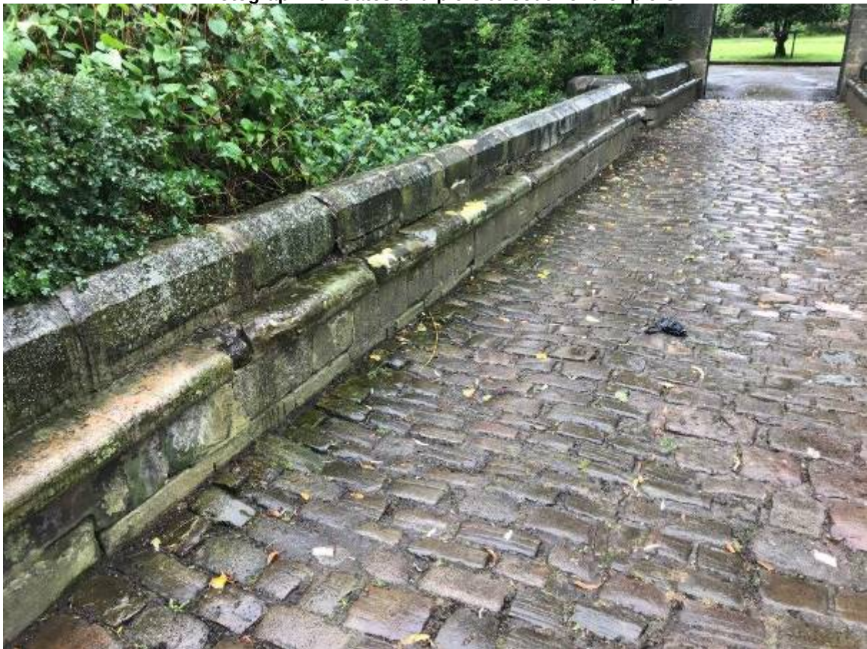
Photograph 70A: Distorted nature of western copings and deterioration at base joint
