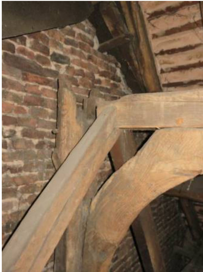
Photograph 13: Collar purlin no longer engaged with crown post but with added struts
