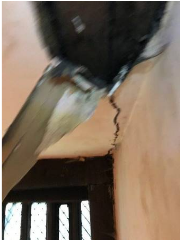
Photograph 25A: Looking east continuation of cracking through ceiling finishes at south gable
