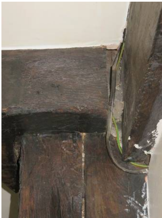
Photograph 30: Minor opening up between cross beam and first floor plate to northern bay
