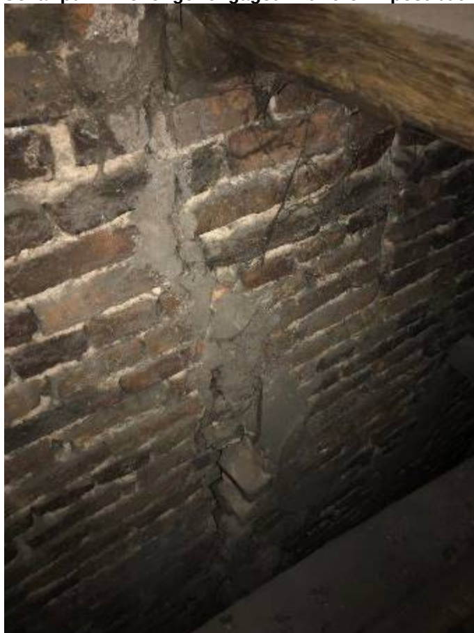
Photograph 13A: Historic crack to end wall of south range
