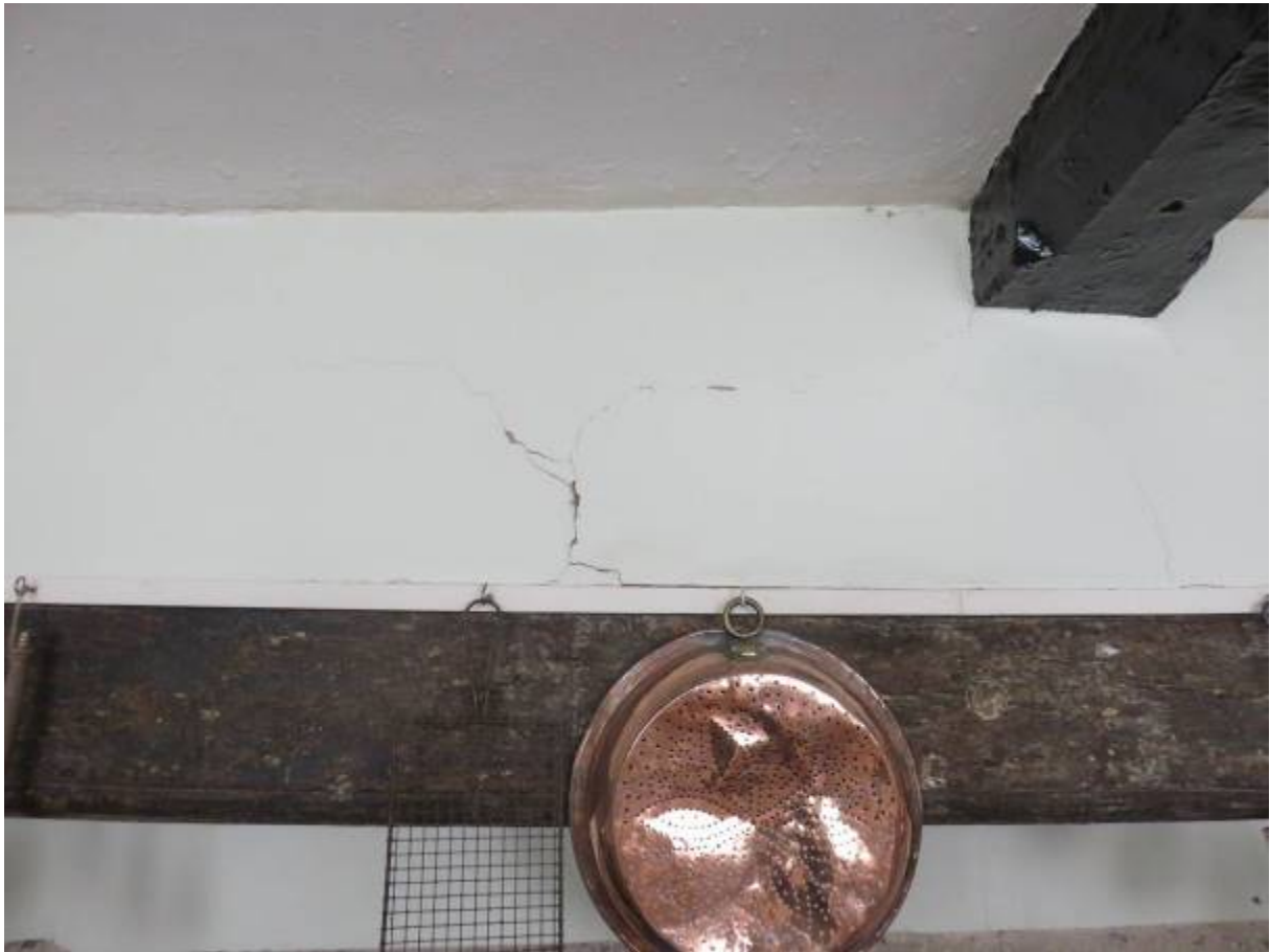
Photograph 62: Minor cracking above timber bressumer to kitchen
