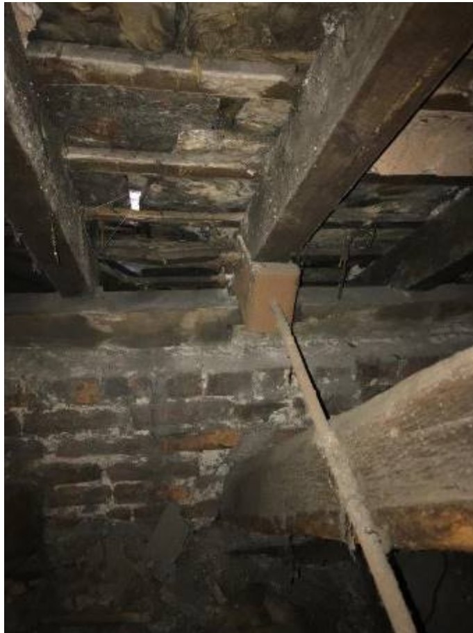
Photograph 11A: Stepped stone slates and water ingress, noting fractured battens
