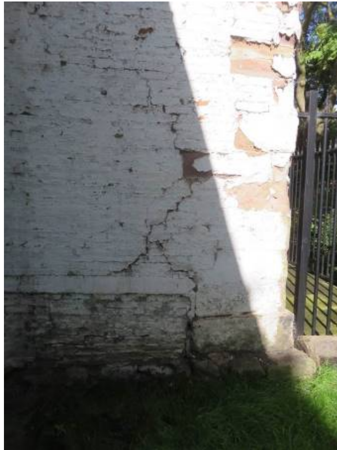
Photograph 48: Close up of movement to south gable
