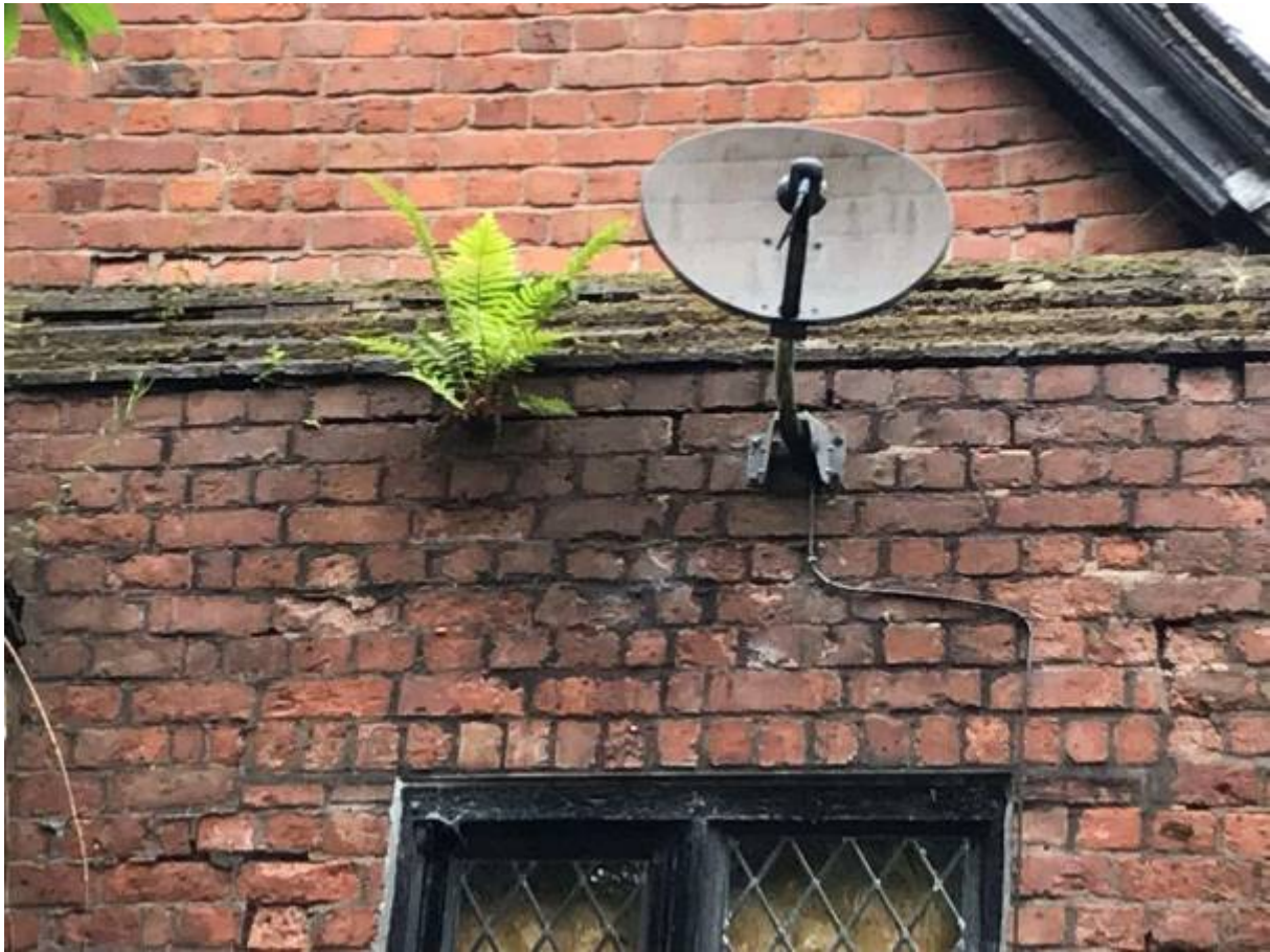
Photograph 42E: Poor condition of upper 9" masonry panel and weatherings to south gable
