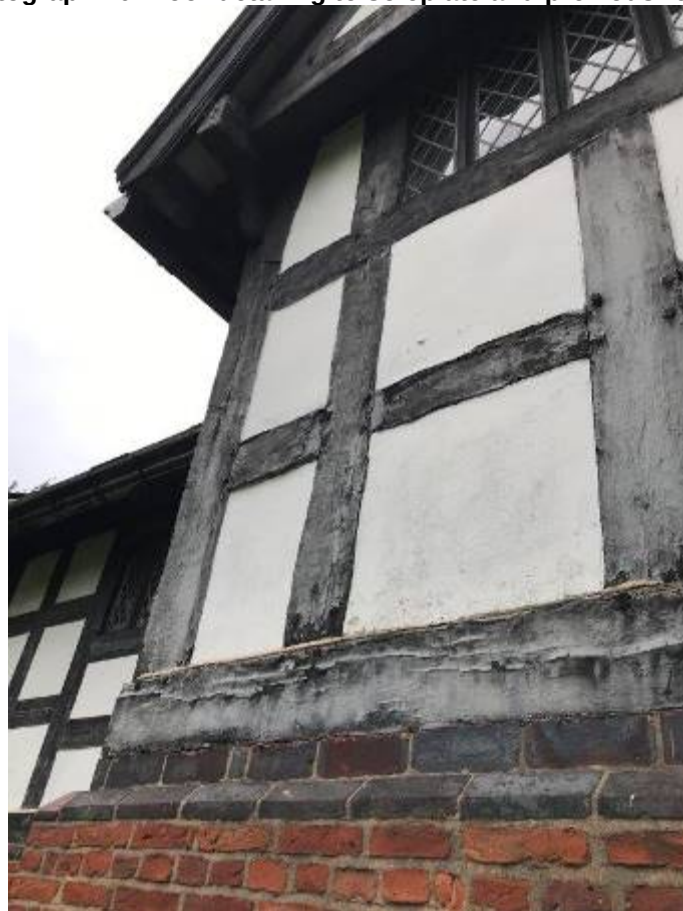
Photograph 40A: East elevation of stair tower. Noticing loss of filler material and increased decay
