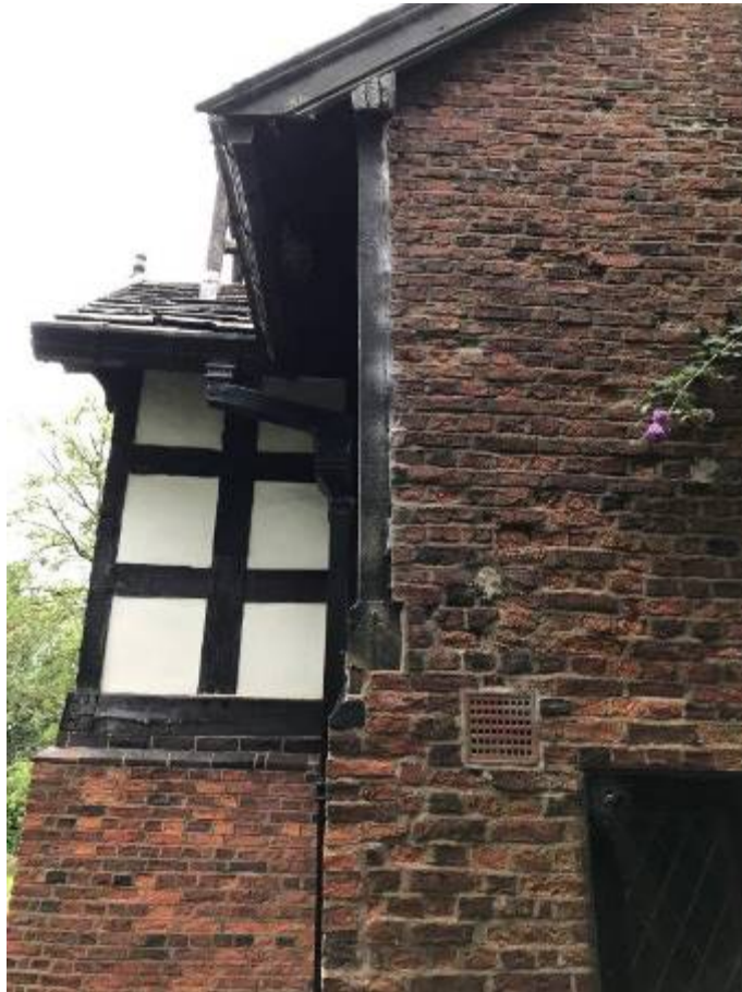
Photograph 41A: Opening up between timber post and adjacent brickwork
