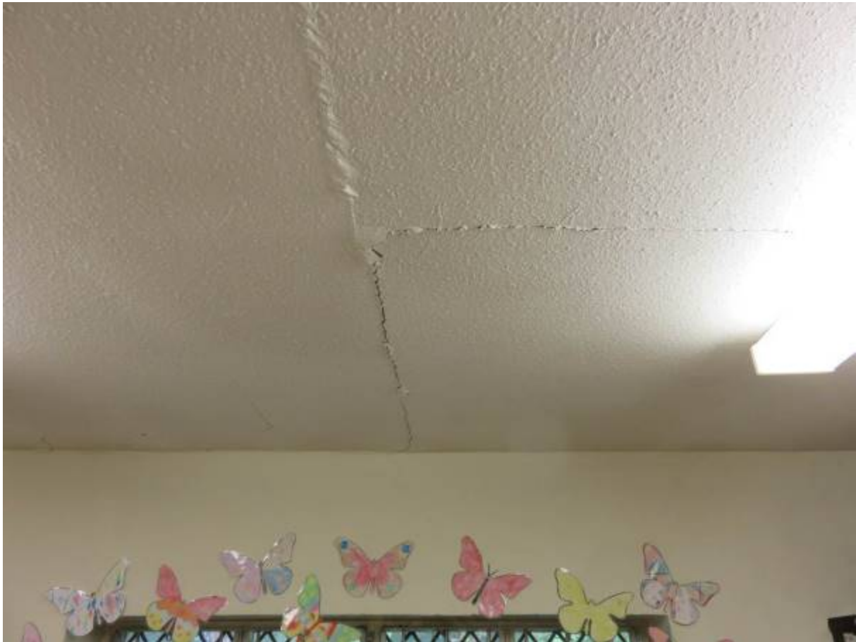
Photograph 52: Cracks in ceiling suggesting probably plaster-boarding or similar
