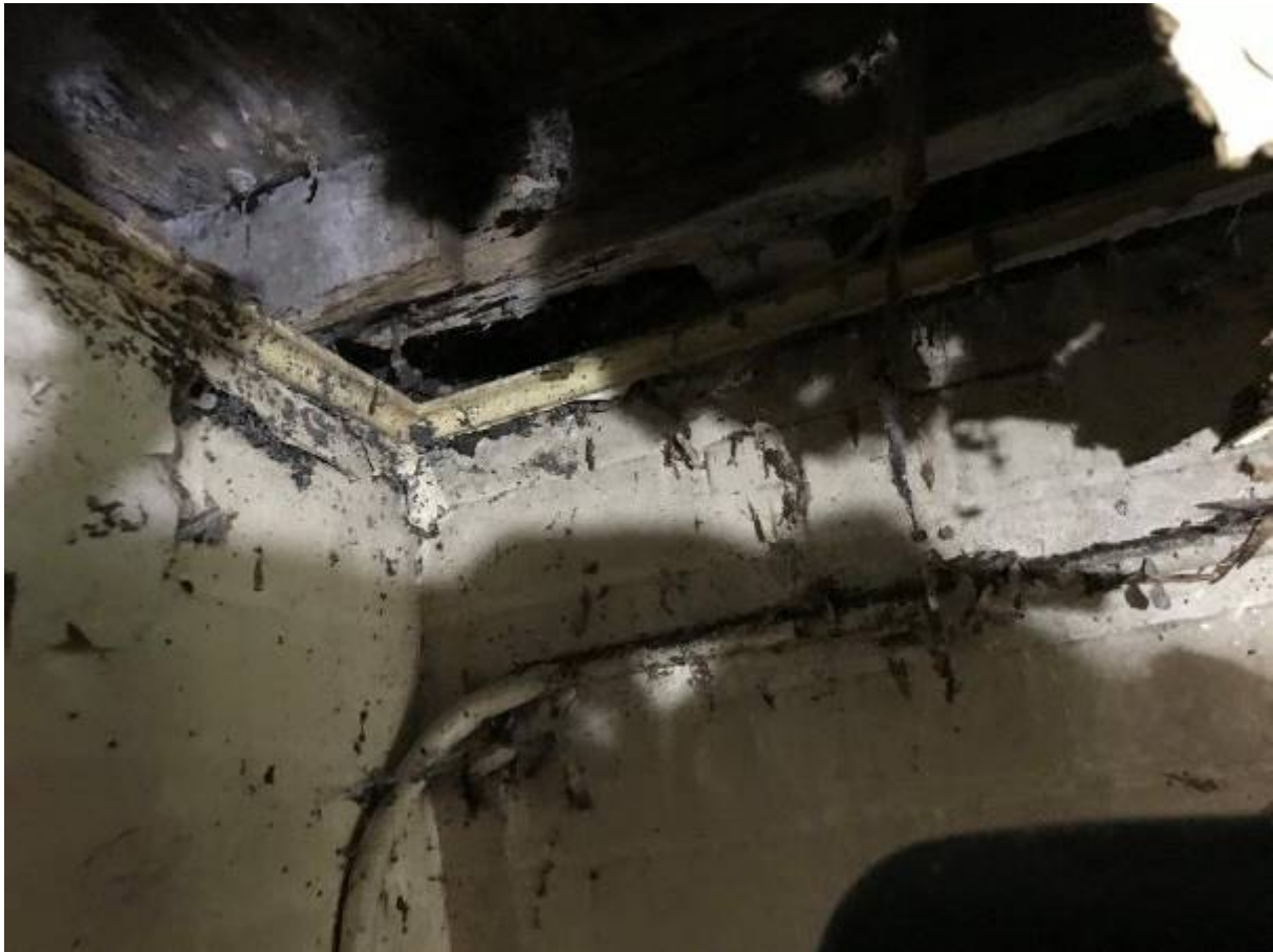
Photograph 66A: Poor condition of flat roof joists
