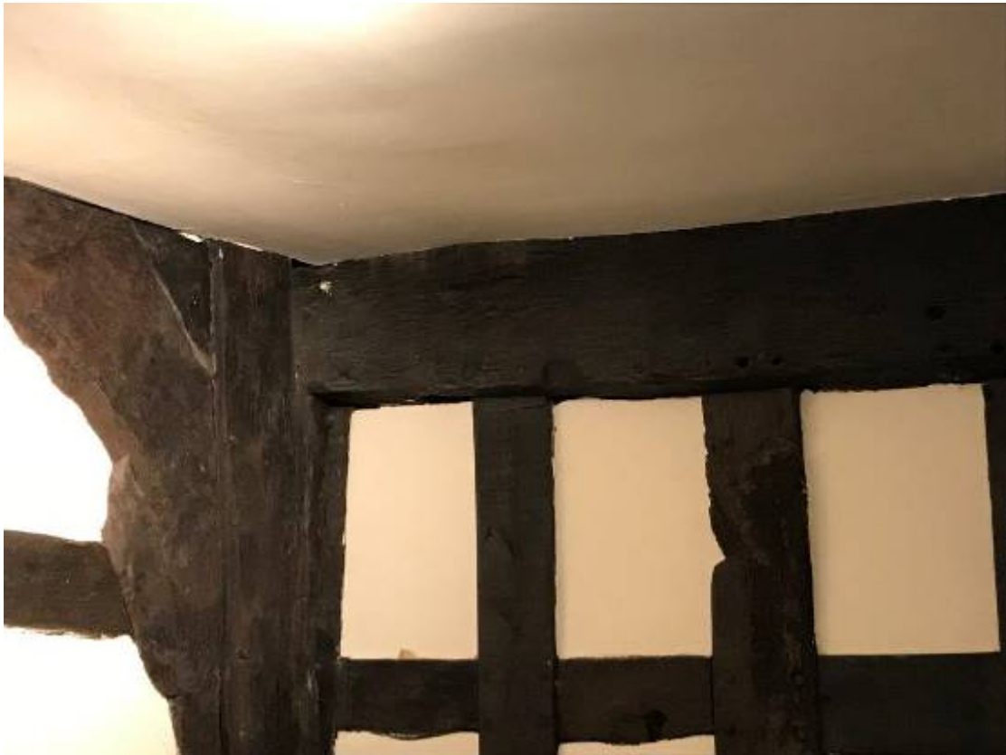
Photograph 15A: Studwork to north panel of east wall to northern bay. Minor opening up noted between frame and finishes
