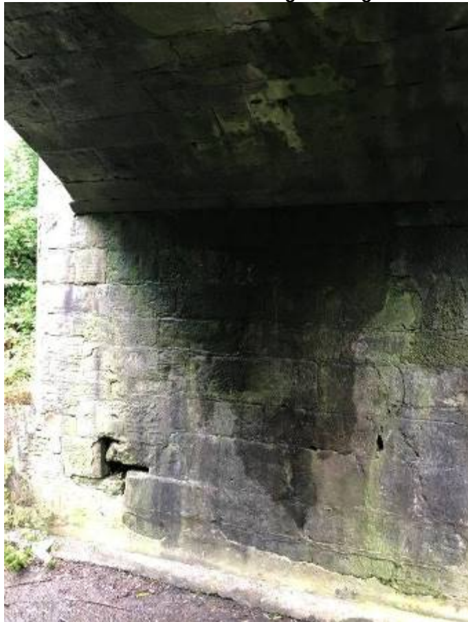
Photograph 71B: Water staining to intrados of central pier, from southern side. Low level void
