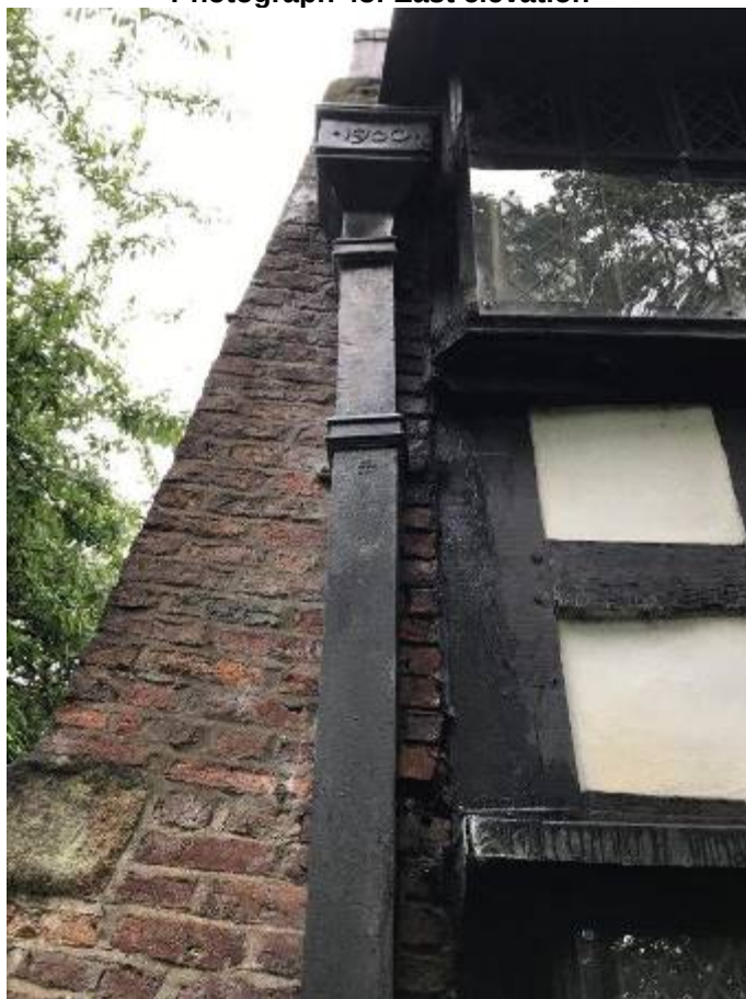
Photograph 43A: Leakage on downpipe and hopper onto material join
