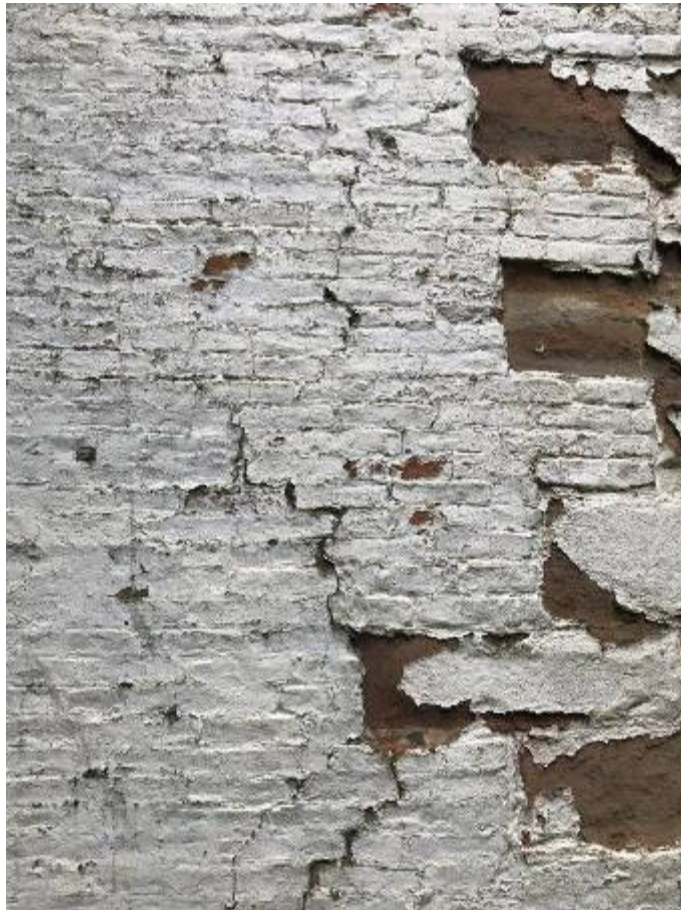
Photograph 48B: Continuation of cracking at higher level to south wall
