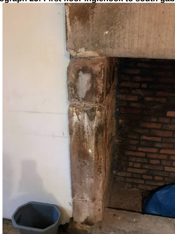
Photograph 23A: Increase of efflorescence and damp upon fireplace surround
