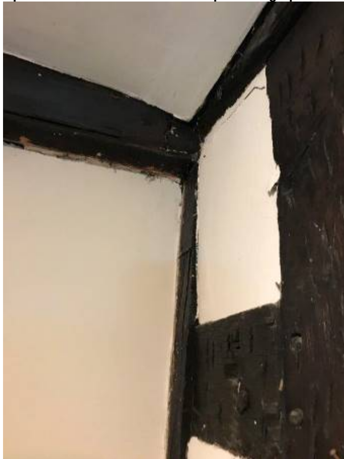
Photograph 34C: South mid-rail to west frame connection indicating fracture to mid-rail and movement in adjacent finishes
