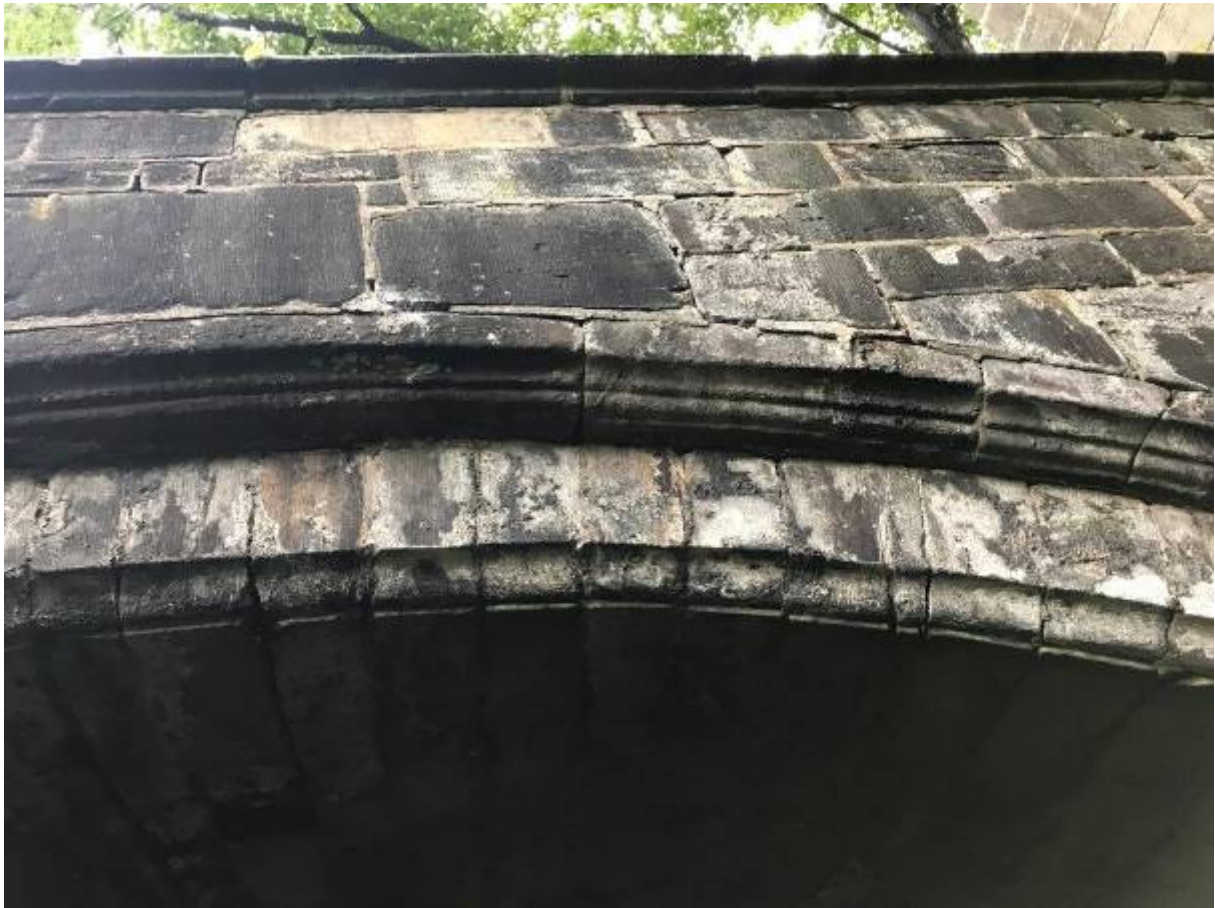
Photograph 70J: Poor condition of masonry joints to the north can arch at its east elevation
