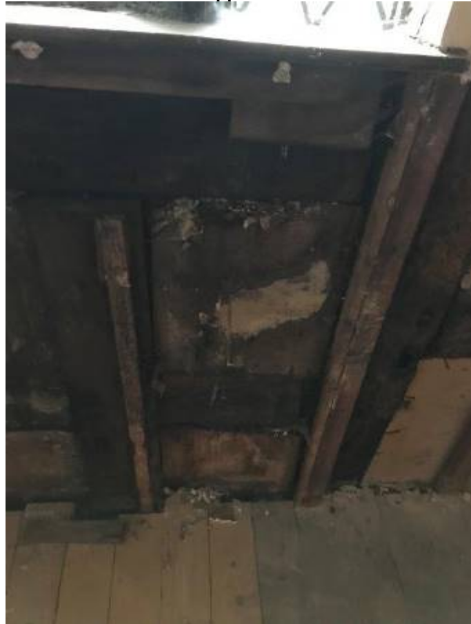
Photograph 28D: Water ingress of stripped back panelling with stair tower
