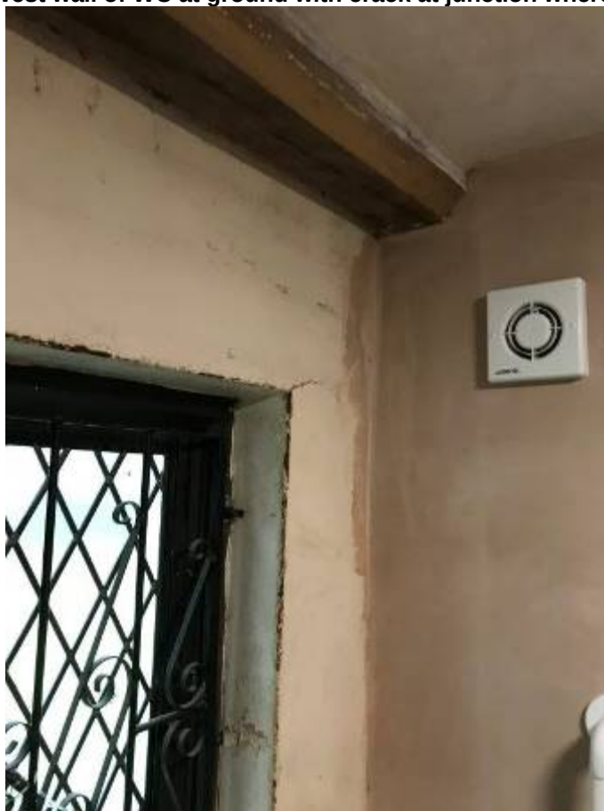
Photograph 37A: Cracking to west bearing of south window 1mm width
