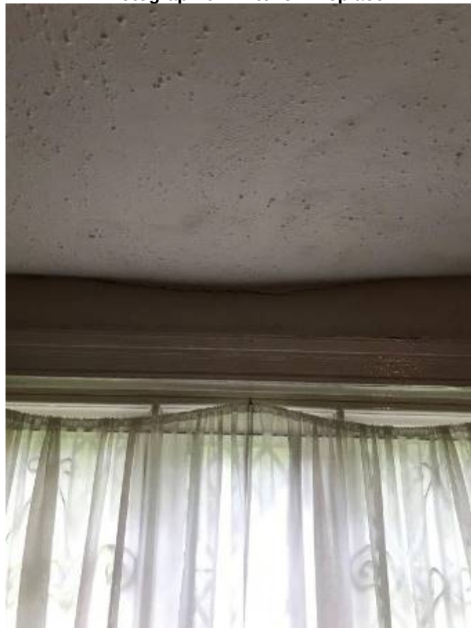
Photograph 61A: Minor differential movement between west wall and ceiling within pressed kitchen
