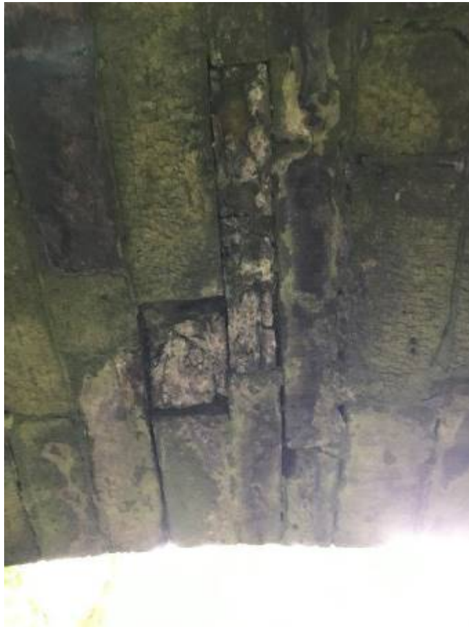
Photograph 70F: More deteriorated profile to finer stone to crest of intrados
