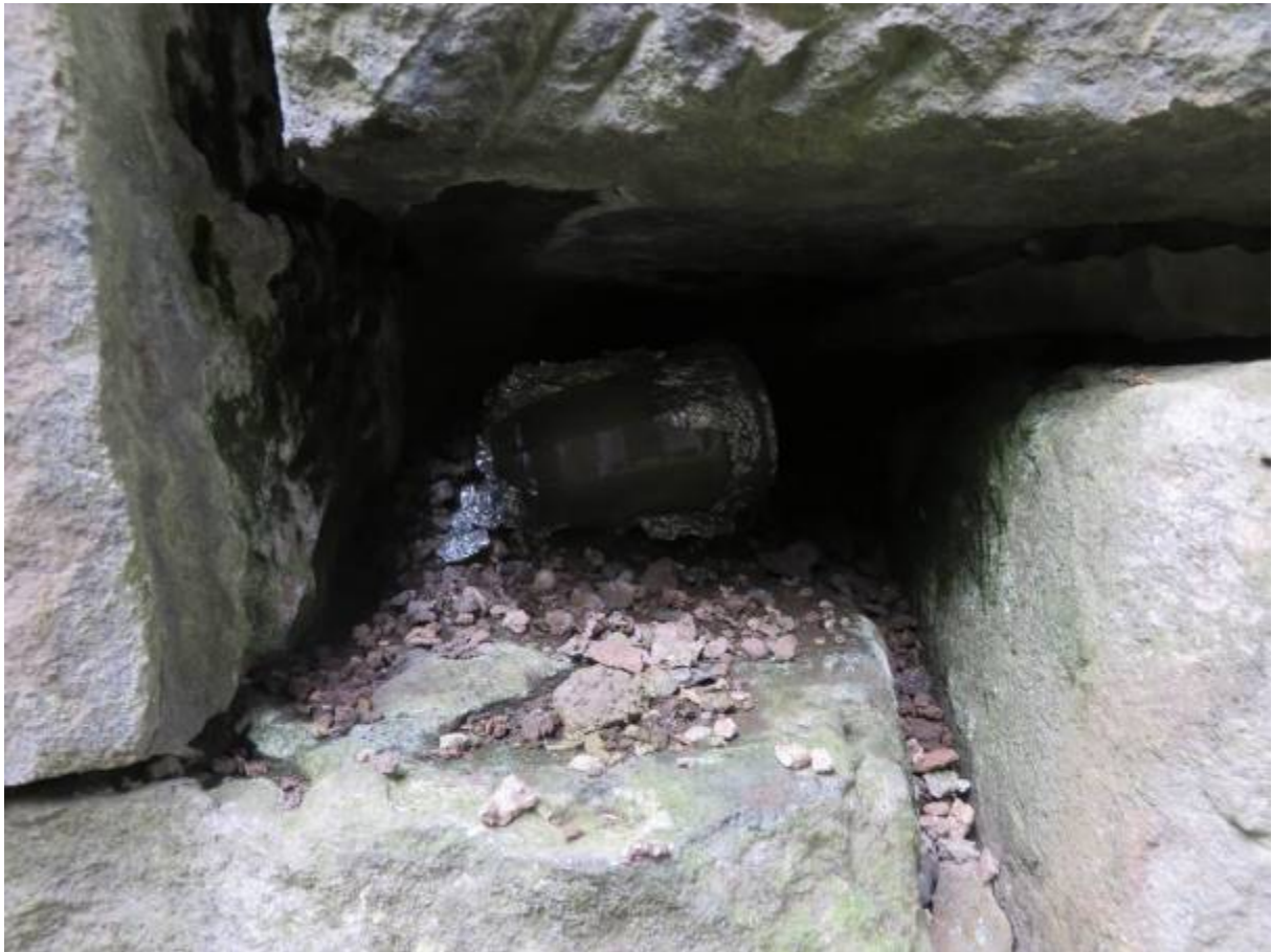
Photograph 72: Void to pier
