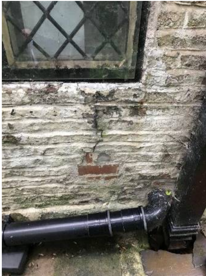
Photograph 46A: Cracking through brickwork to east elevation around drains
