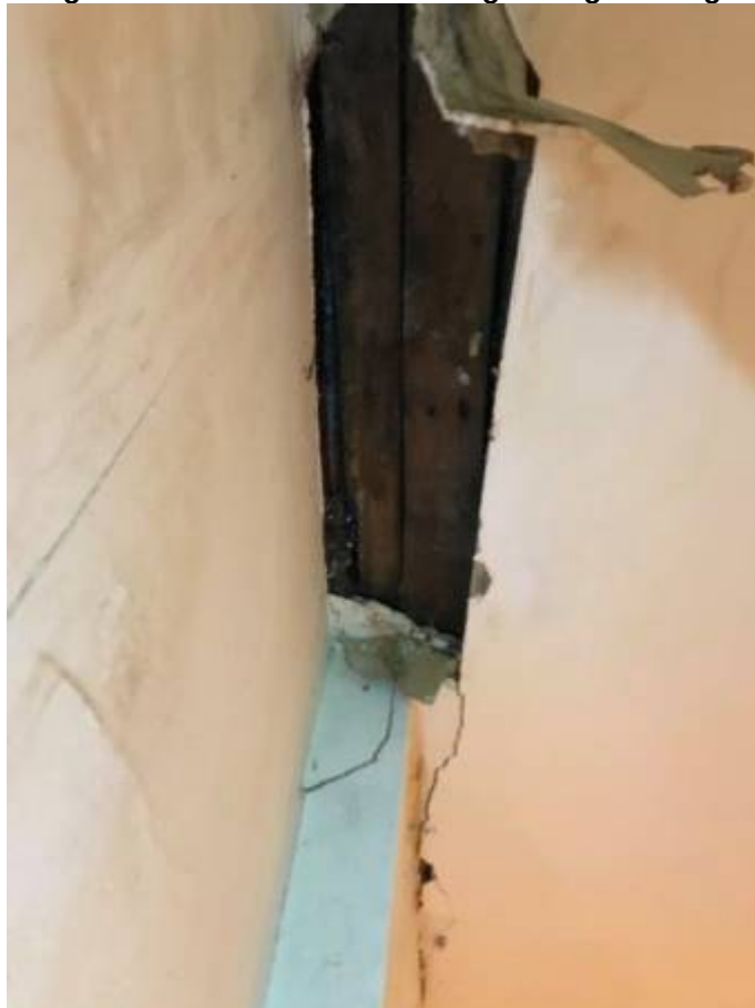
Photograph 25B: Cracking and loss of plaster at stack
