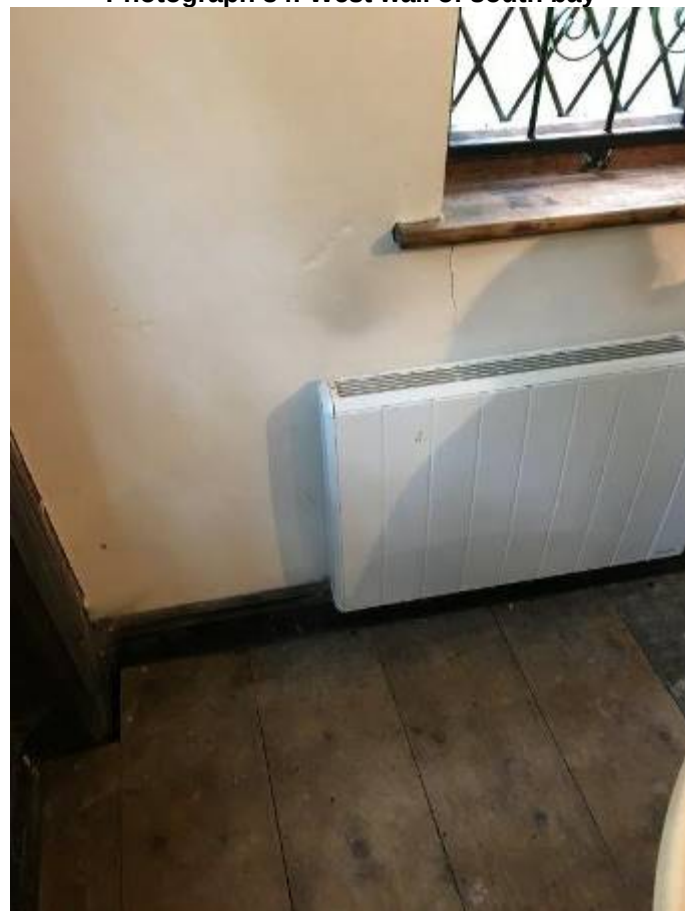
Photograph 34A: Cracking from sill downward within southern range indicating recent movement
