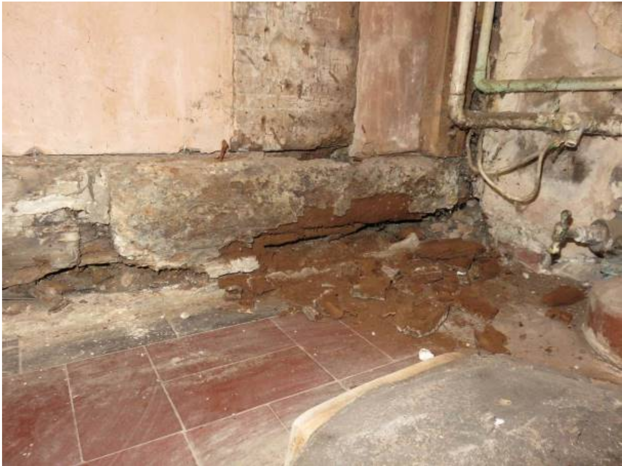
Photograph 36: Historic decay to soleplate to south end of southern bay
