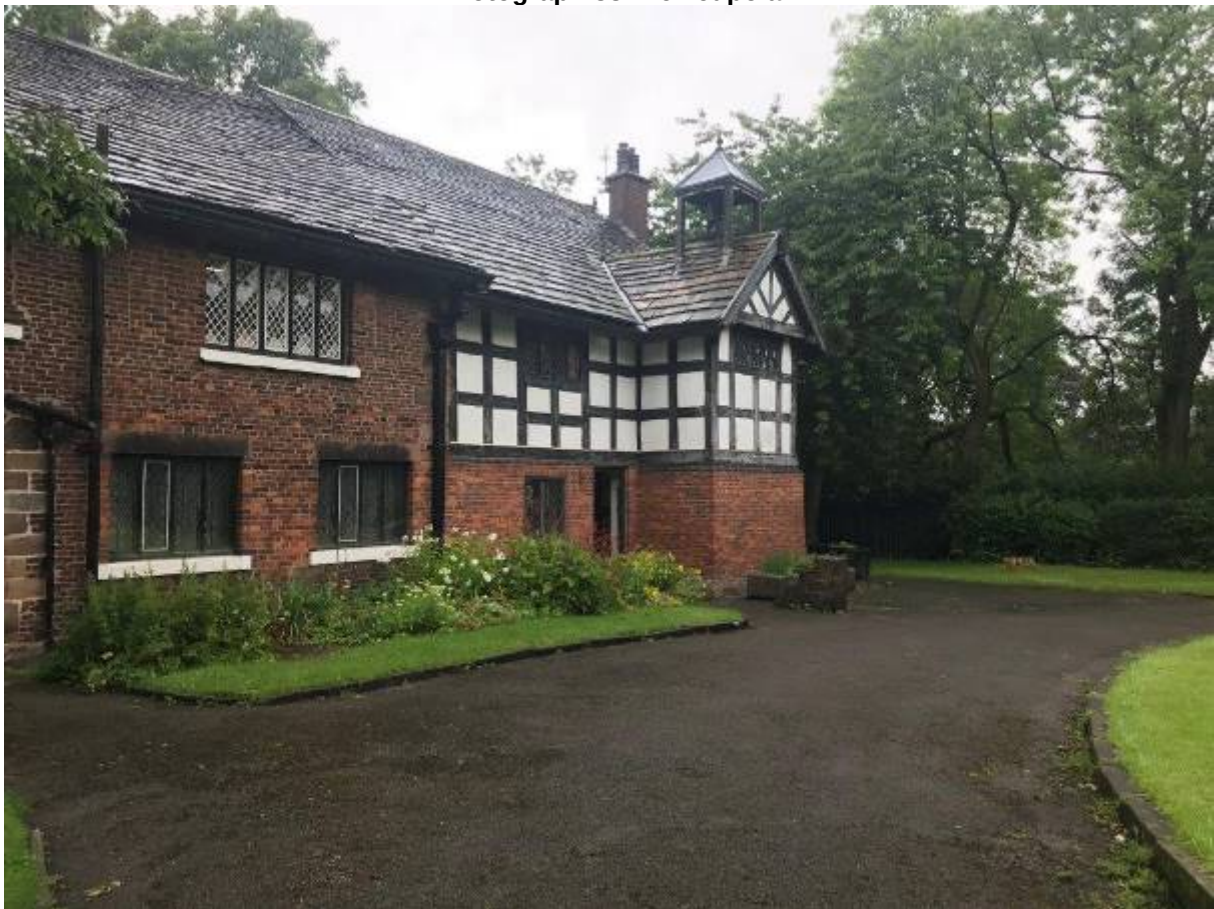
Photograph 38A: General photo showing condition of west slope of roof
