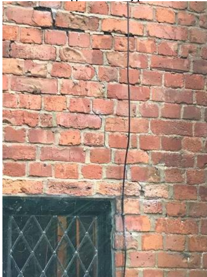
Photograph 42F: Stepped cracking above ground floor lintel indicating failure
