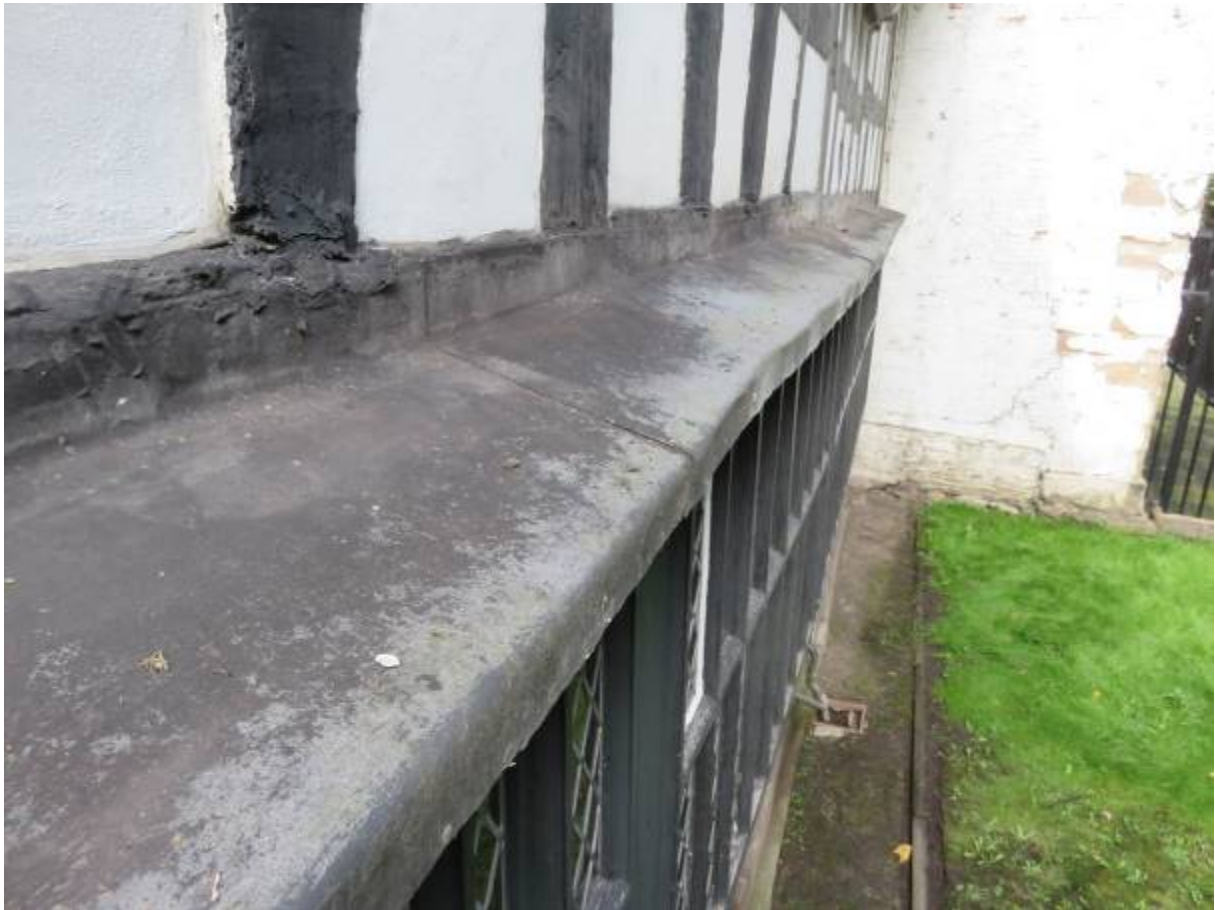
Photograph 45: Weathering to head of window, appearing to be holding at present
