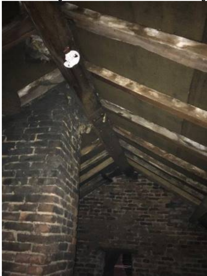
Photograph 51B: Loss of membrane either side of stack. Note previous steel angle plate repair to ridge beam
