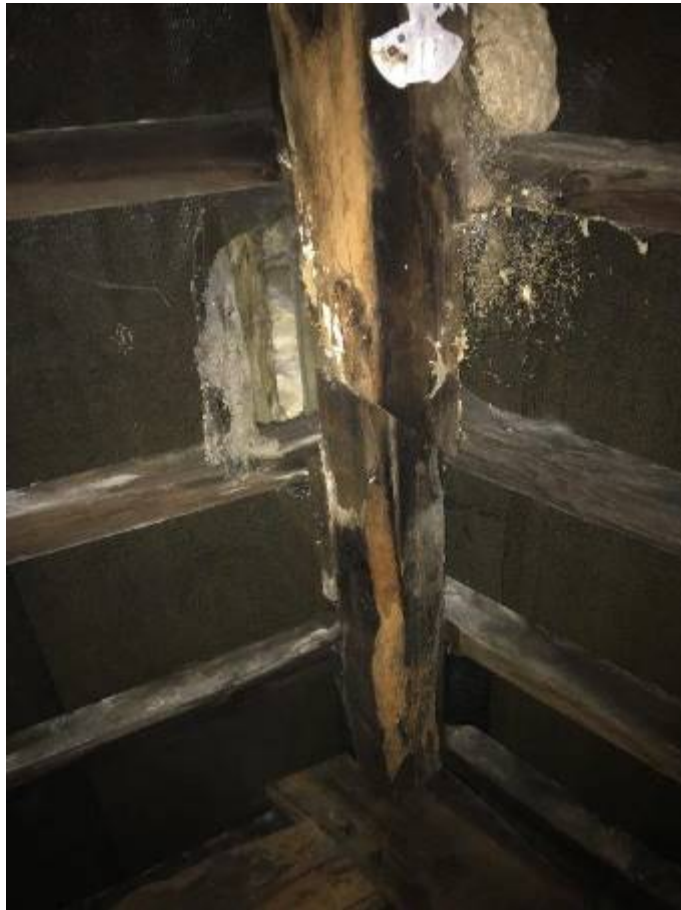
Photograph 51C: Loss of membrane and water ingress into adjacent ridge beam which shows decayed condition
