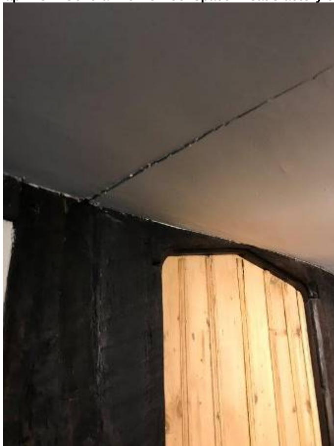
Photograph 28B: Cracking between boarded panels to ceiling within corridor
