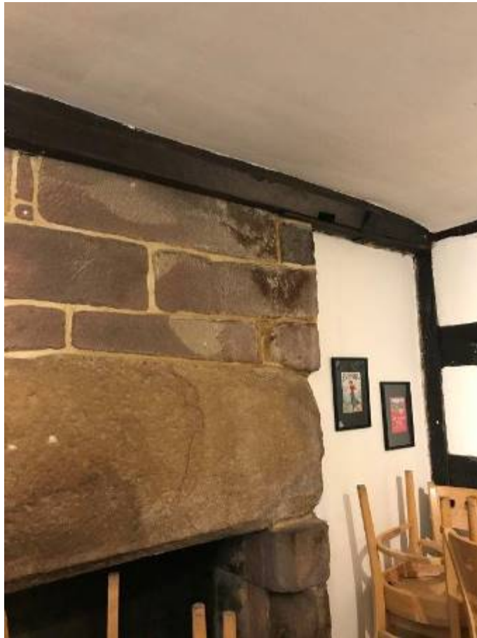
Photograph 34B: Efflorescence and damp staining upon the fireplace
