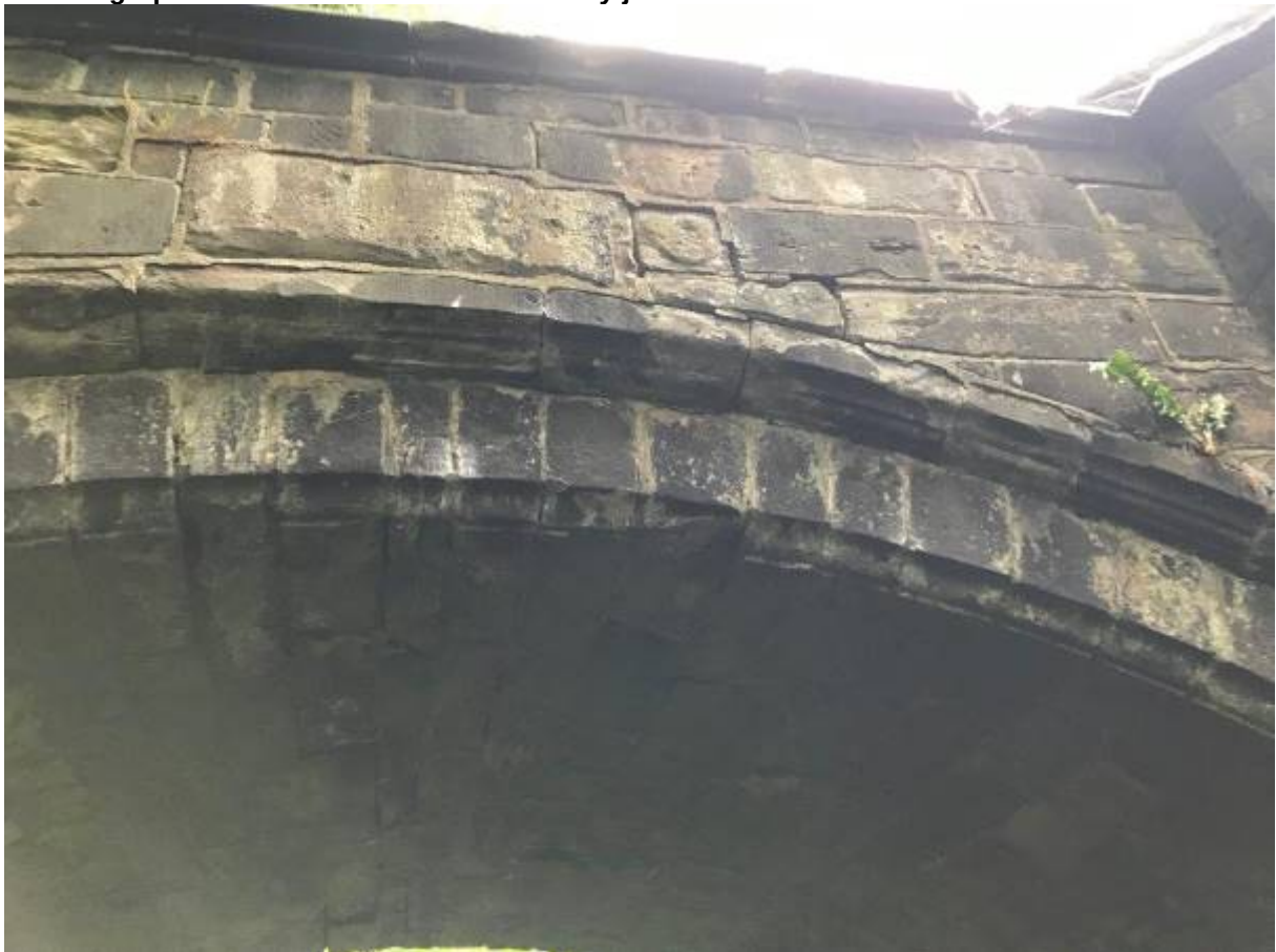
Photograph 70K: Poor condition of masonry joints to the northern arch at its west elevation
