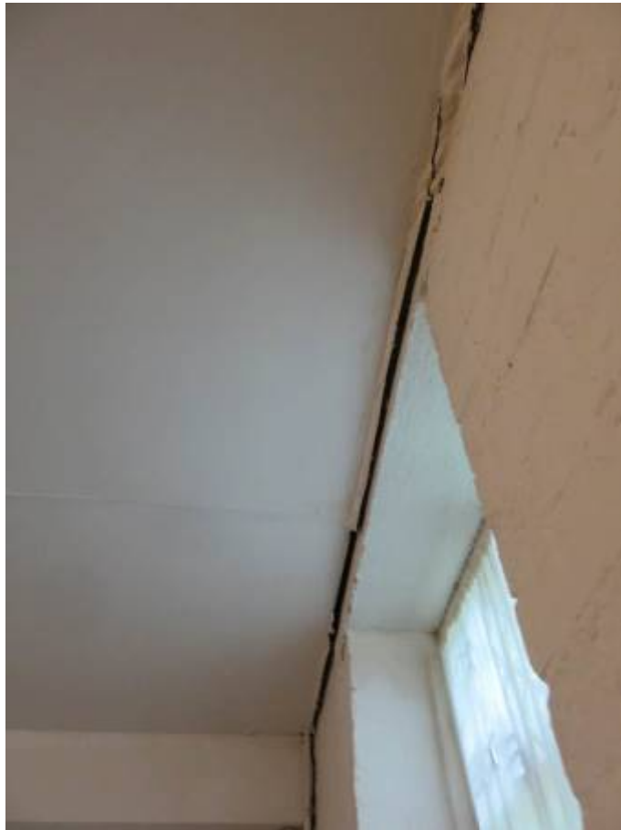
Photograph 60: Movement of floor/ceiling to east side of larder
