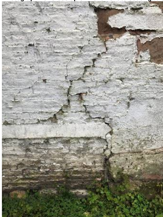
Photograph 48A: Cracking and deterioration to south wall of north range
