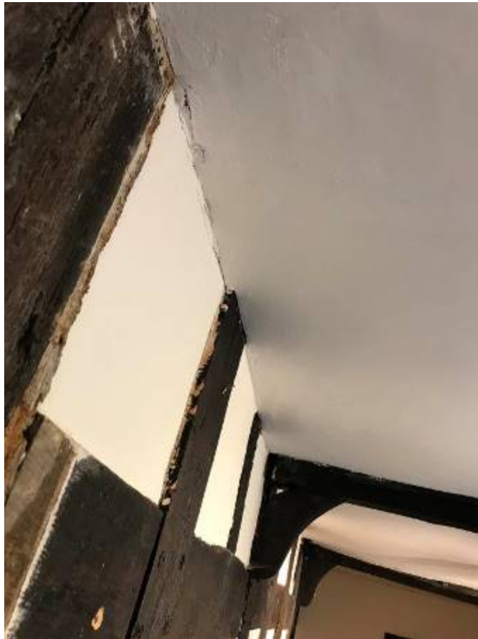
Photograph 34D: Opening up between west wall and ceiling in corridor
