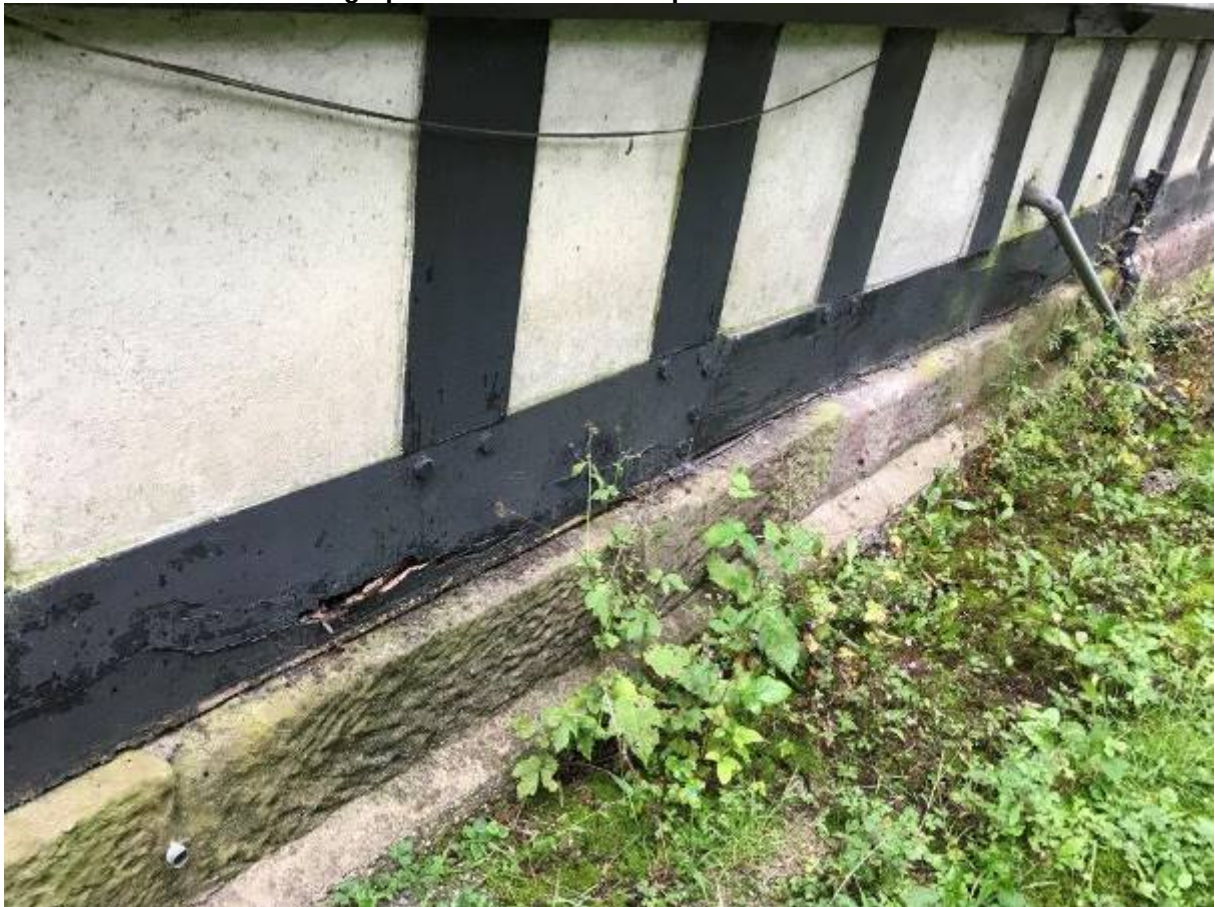
Photograph 44A: Decay to base of soleplate which sits upon DPC.
