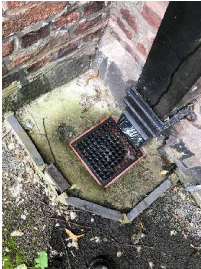
Photograph 41C: Downpipe gully with cracking where this meets sides of adjacent building
