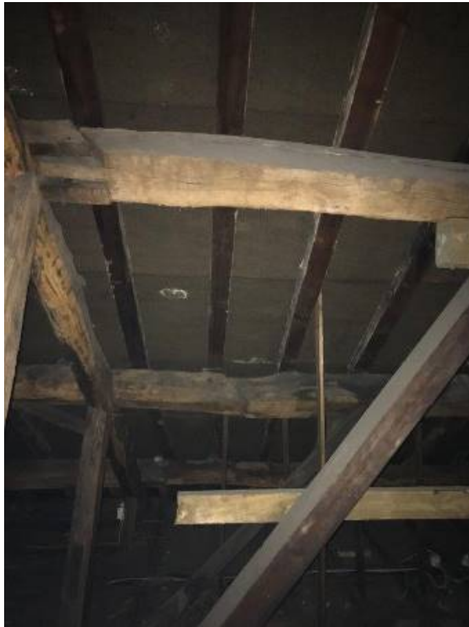
Photograph 49A: Spliced joints to purlins with hinging taking place at these points. Note packing between purlin and rafter level
