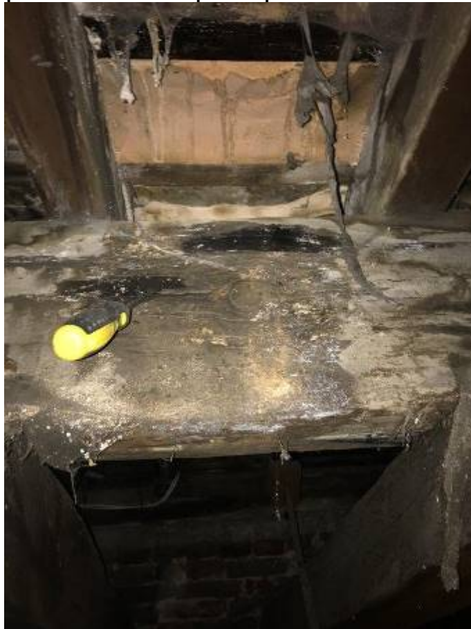
Photograph 12B: West flank at blind window with water ingress onto purlin
