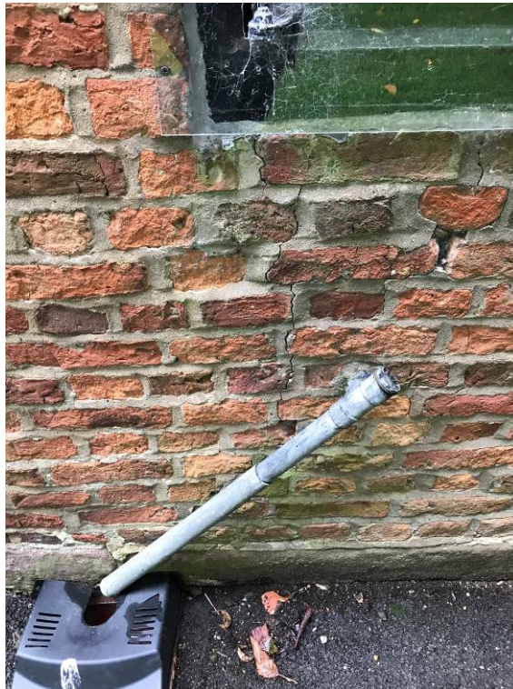
Photograph 42A: Active 1 – 2mm width cracking from sill level downwards
