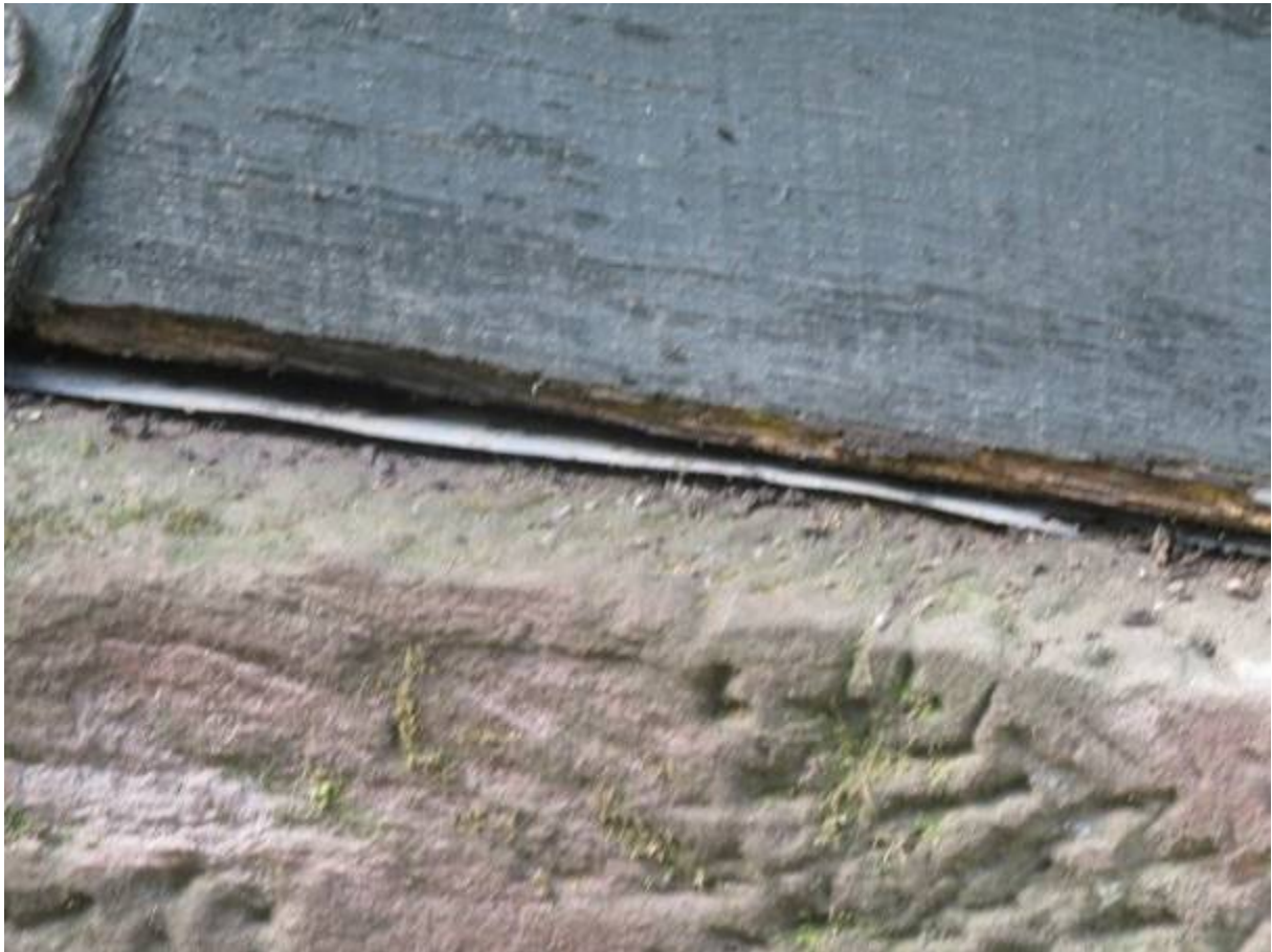
Photograph 44: DPC below soleplate to east elevation
