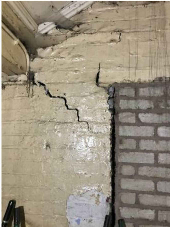
Photograph 68B: Diagonal cracking from timber beam bearing toward adjacent opening, with north west corner of building clearly dropping
