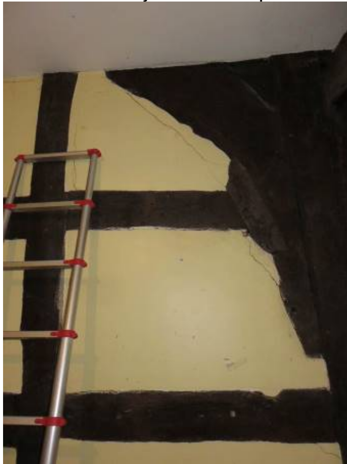
Photograph 18: Minor cracking to assumed infill plaster main frame
