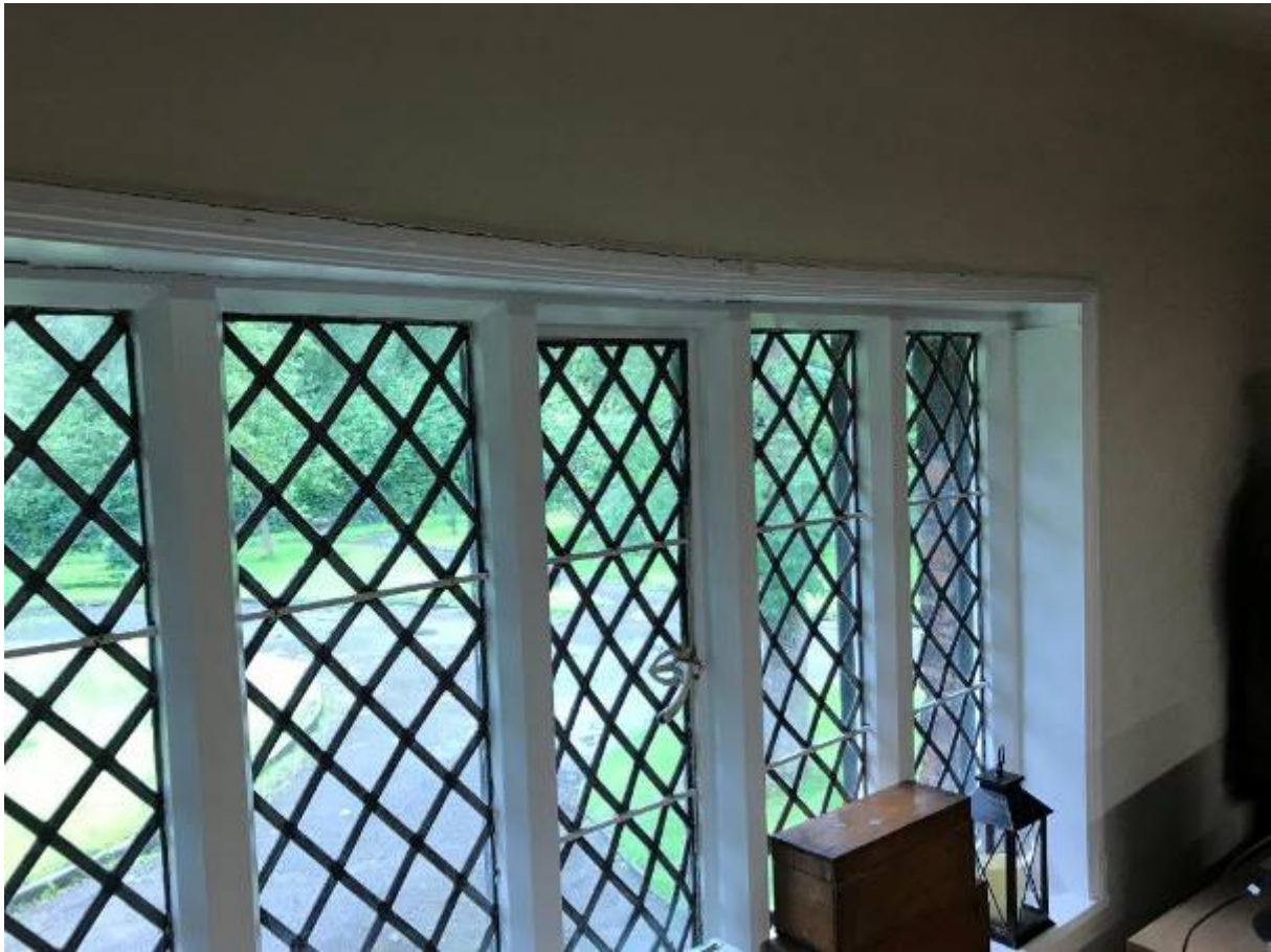
Photograph 28C: Opening up between window frame of plaster, noting slight dropping mullion frame o upper architrave
