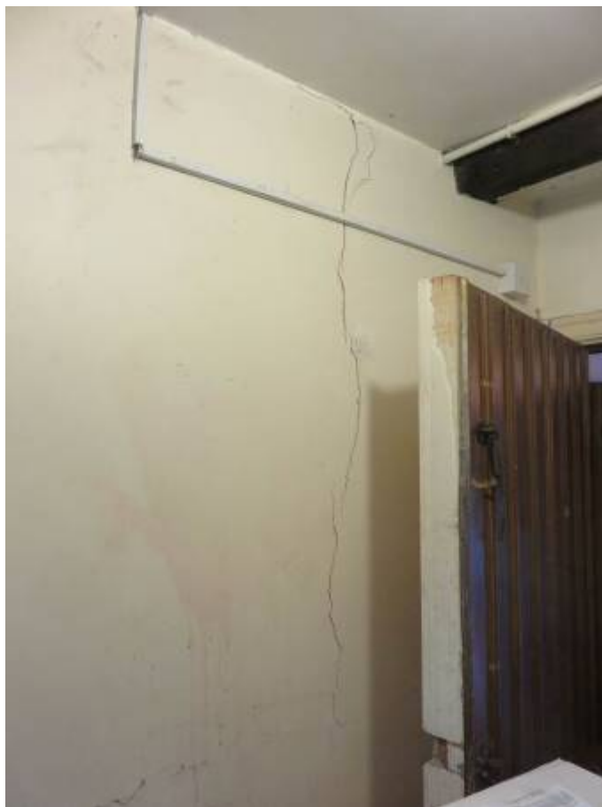
Photograph 37: West wall of WC at ground with crack at junction where stair tower abuts
