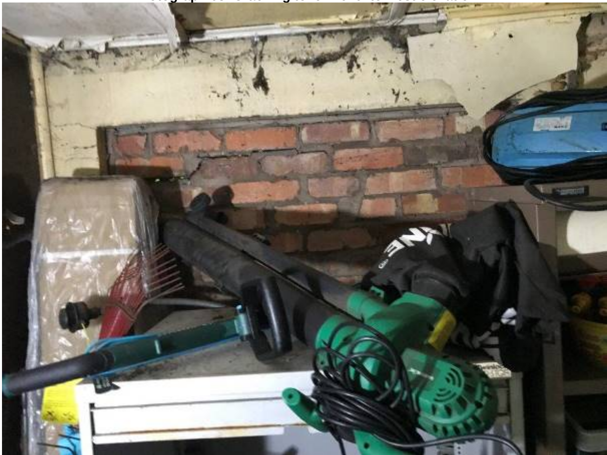
Photograph 68A: Horizontal cracking through the bricked in opening to west elevation
