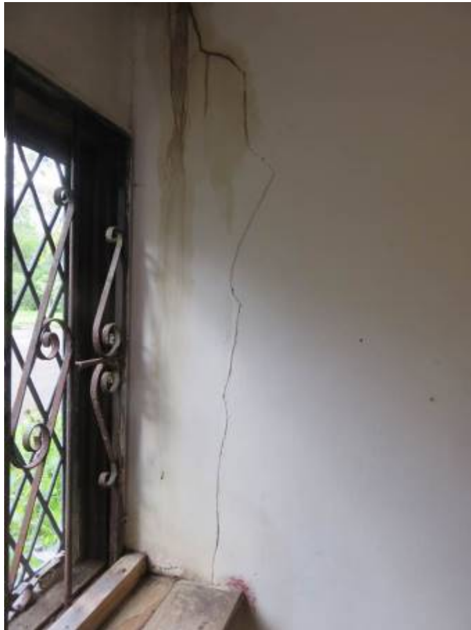
Photograph 35: Cracking to corridor of west wall at position of later infill
