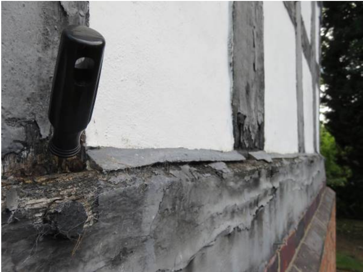
Photograph 40: Poor detailing to soleplate and previous repairs
