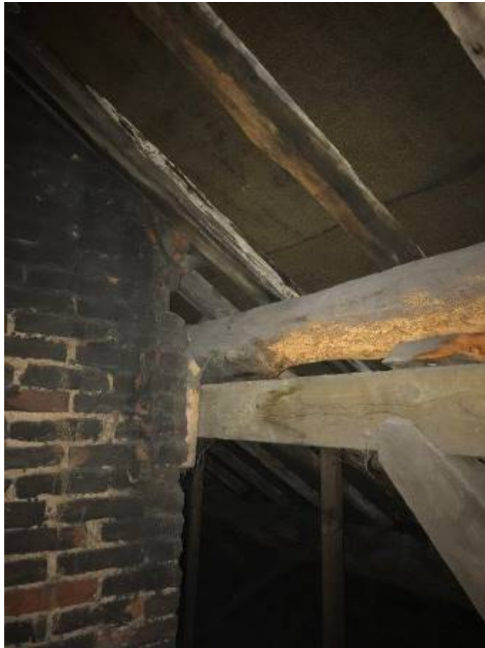
Photograph 51A: Water ingress to common rafters and doubling up to purlin
