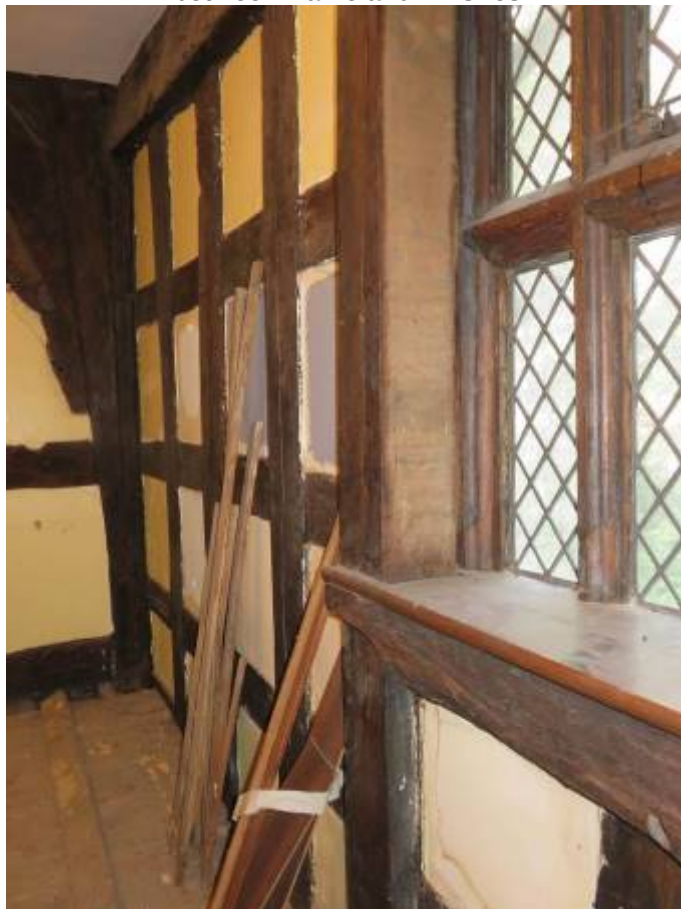
Photograph 16: Post sitting proud of wall face and supporting cill
