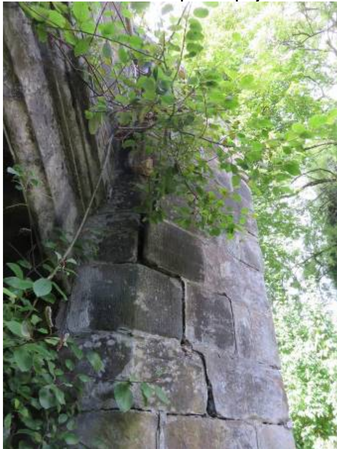
Photograph 71: Shrub growth to eastern side of bridge
