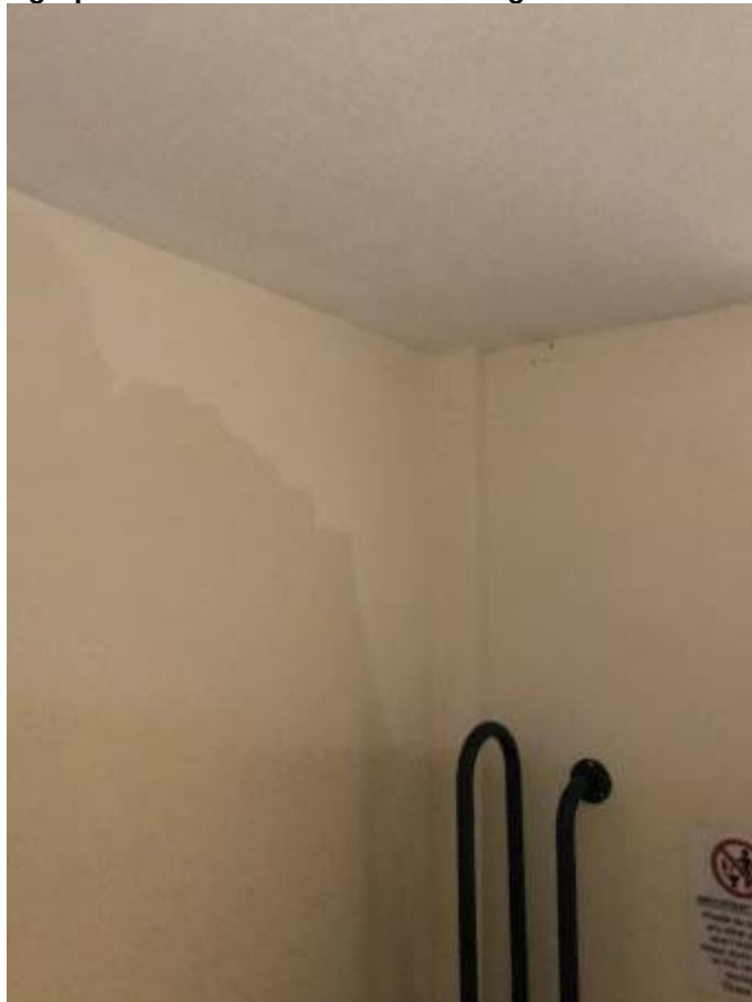
Photograph 60A: Damp staining to north wall of WC
