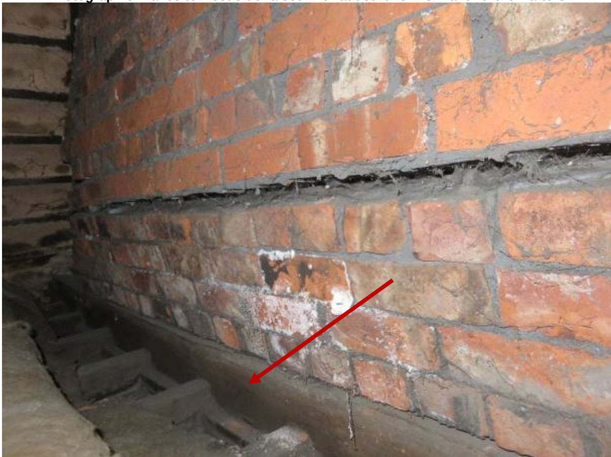
Photograph 9: Timber plate built into south gable (highlighted) with fracture above
