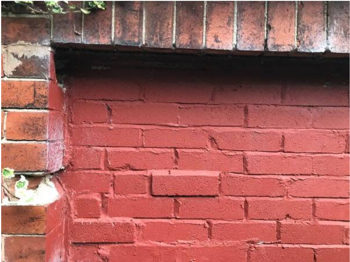
Photograph 69A: Rust jacking at bearing of steel angle lintels to west elevation
