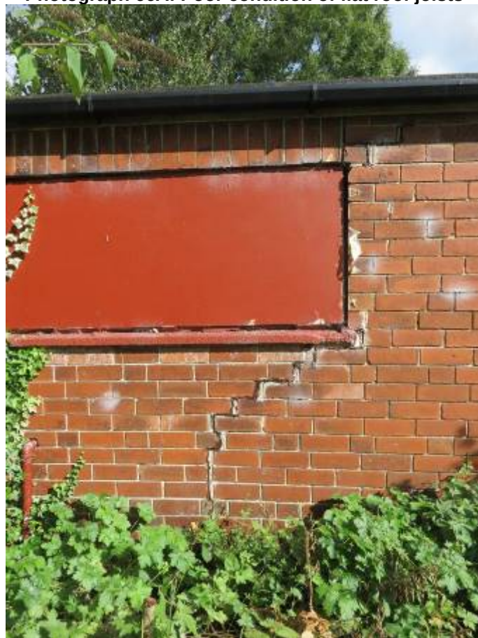
Photograph 67: Cracking to west elevation
