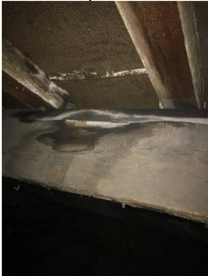
Photograph 51D: Water ingress and leak at puncture to membrane upon purlin to east flank
