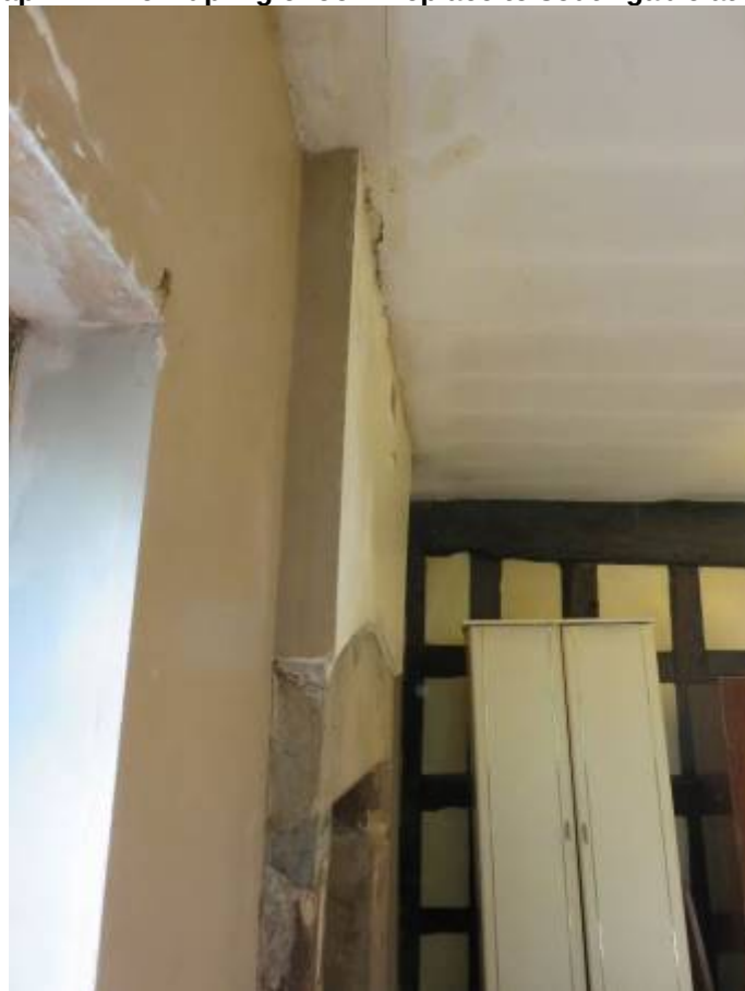
Photograph 25: Apparent minor movement to wall above fireplace
