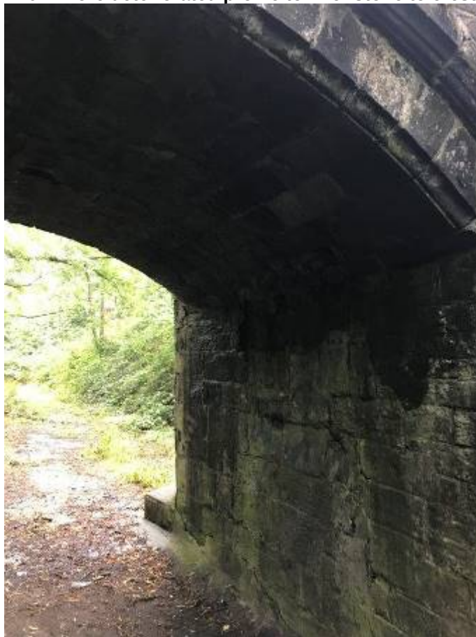
Photograph 70G: Damp staining to barrel toward central pier indicating moisture ingress through deck build up
