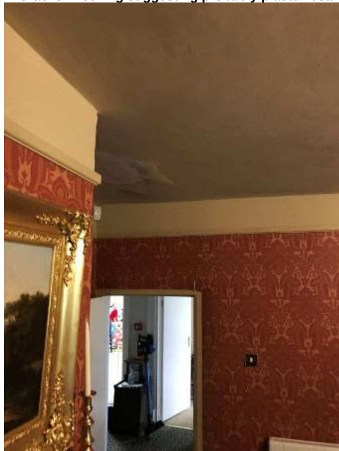
Photograph 52A: Water damage to drawing room ceiling
