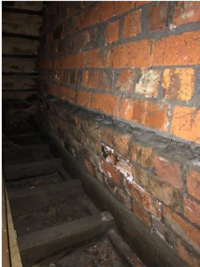
Photograph 9A: Worsening of rotational movement to south gable
