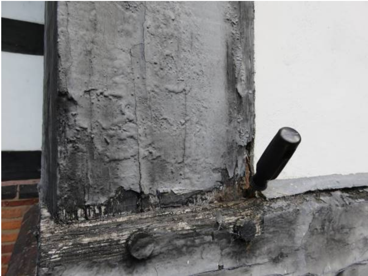
Photograph 39: Decay pocket to the north end of the west elevation of the stair turret
