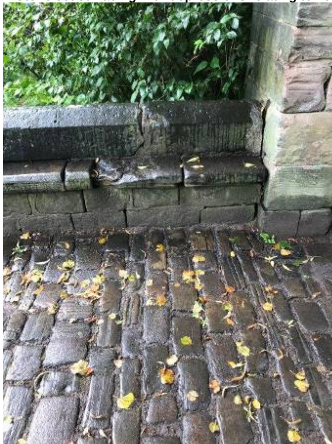
Photograph 70E: Opening up between western parapet stone and adjacent pier
