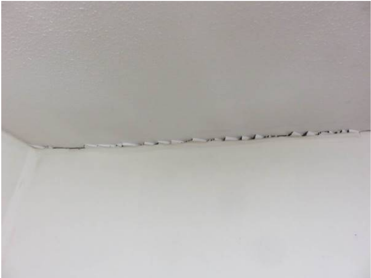
Photograph 53: Movement to first floor kitchen ceiling wall junction
