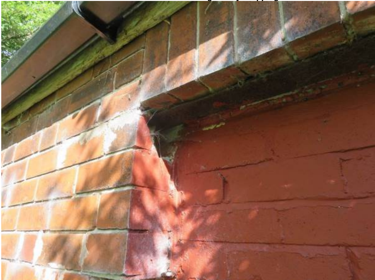
Photograph 69: Window head with steel flat bar lintels and associated corrosion jacking
