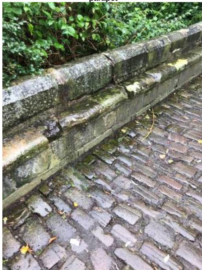
Photograph 70C: Disjointed coping blocks to west side where vehicle impact may have influenced
