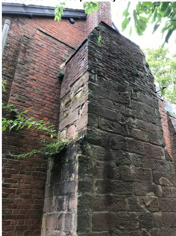
Photograph 42D: Vegetation growth to stack as well as poor condition of weatherings
