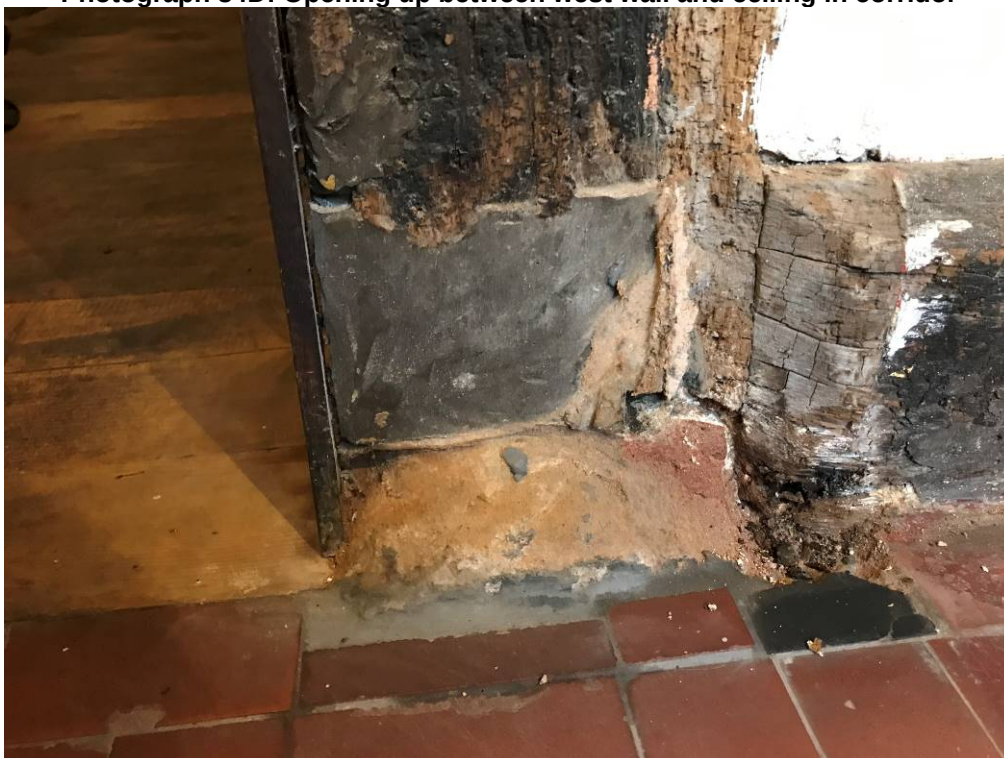
Photograph 34E: Decay to soleplate adjacent to entrance onto north bay
