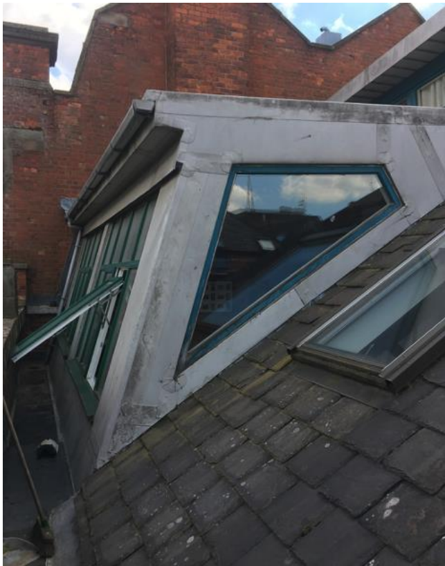
(Figure 9 Existing patched trocal dormer dating back to 1997)
