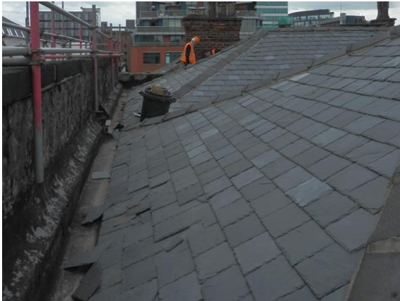
Fig. 9: View over the roof of 56 Dale Street, showing state of repair before / during conversion works
