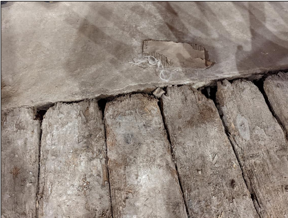
Decayed timber boards butted by concrete
