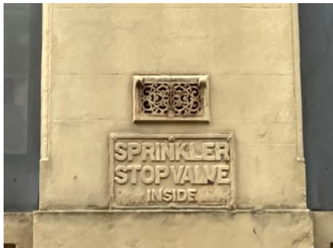
Photo 3C Sprinkler Marker Plate (directly below alarm gongs)
