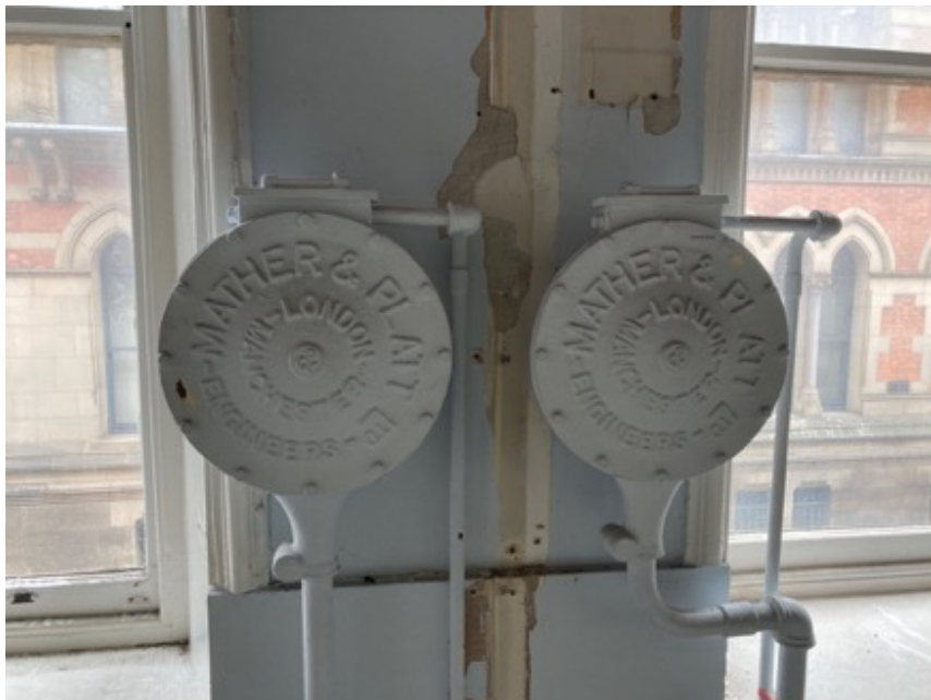
Photo 3A Interior of building showing rear of rotary alarm gongs
