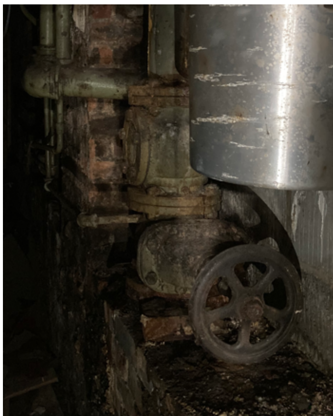
Photo 6: Extensively corroded alarm valve
