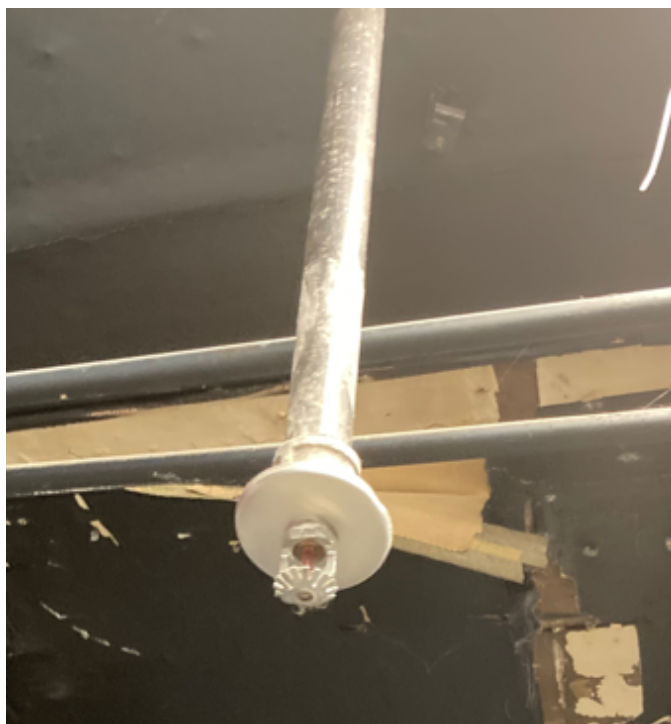
Photo 5: Modern sprinkler head and pipework
