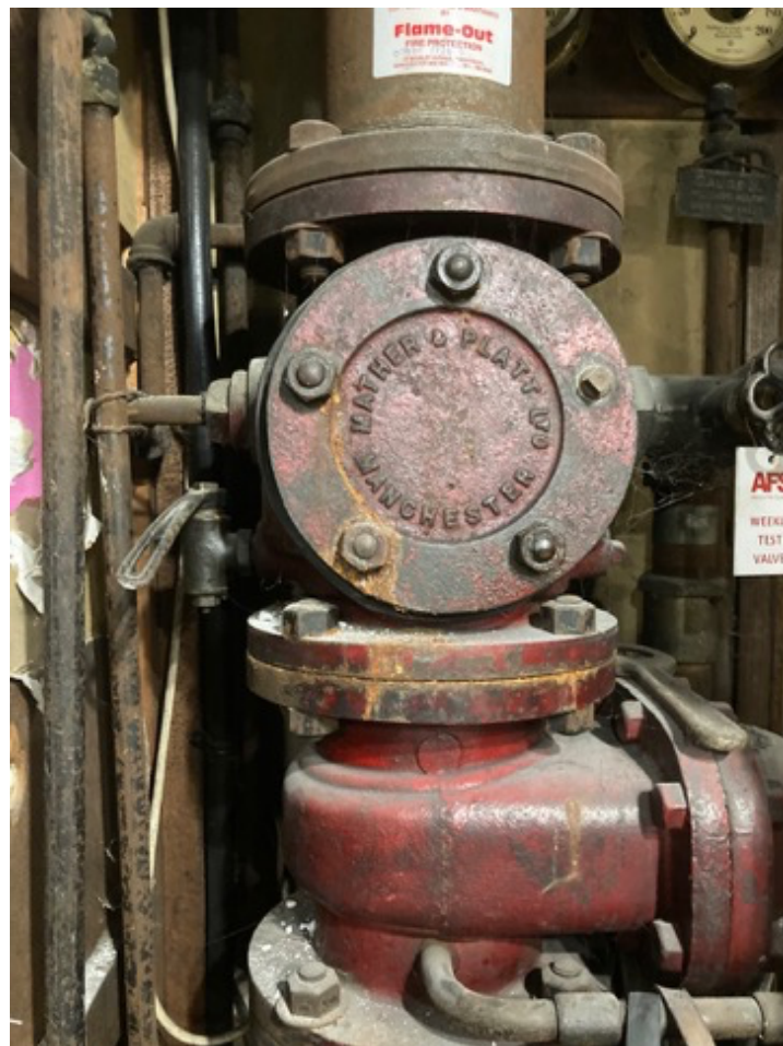
Photo 1: Detail of Sprinkler Alarm Valve
