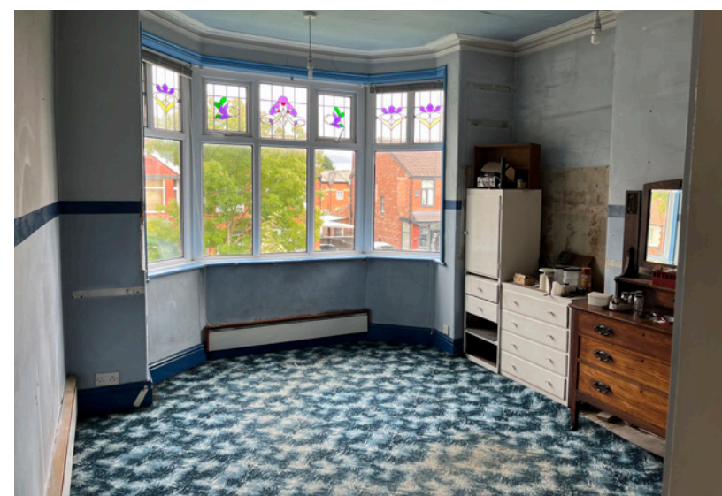
Poor condition of existing internal spaces
