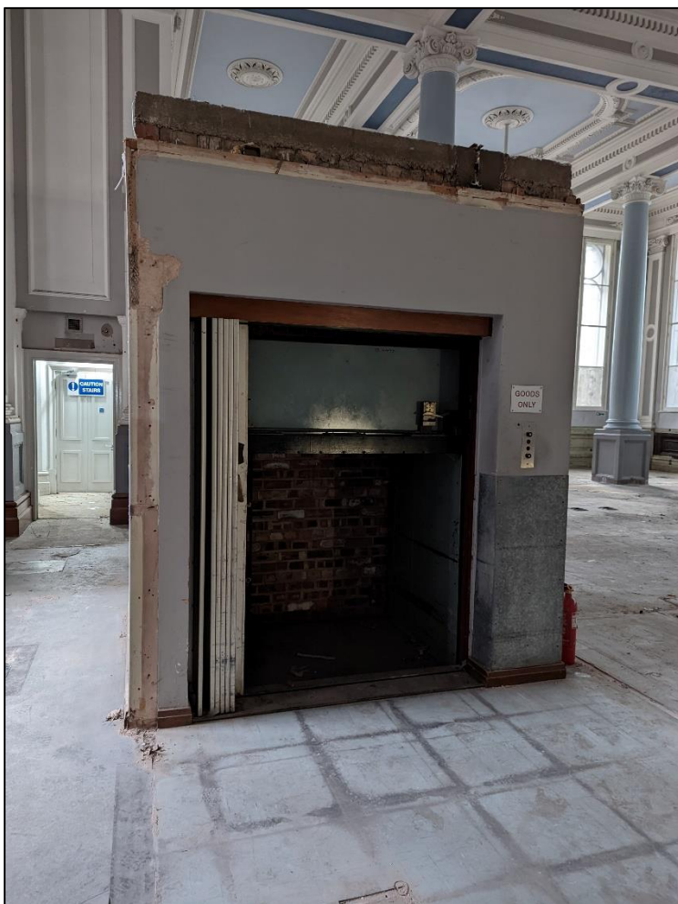
Plate 38: Goods lift to basement
