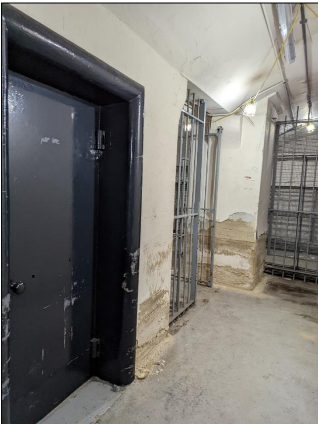
Plate 107 as above showing arched ceiling
