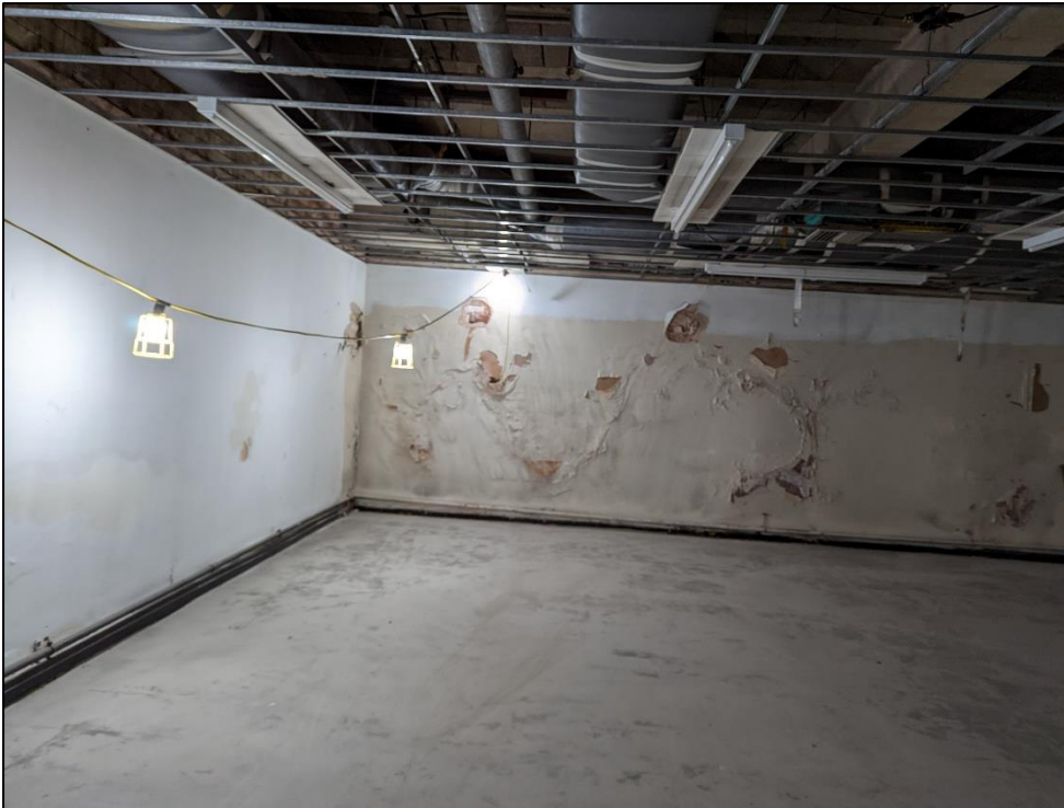
Plate 112: As above showing decaying plasterwork
