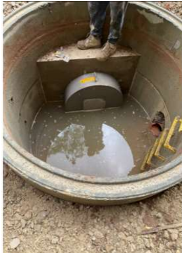
Image of installed Hydrobrake
