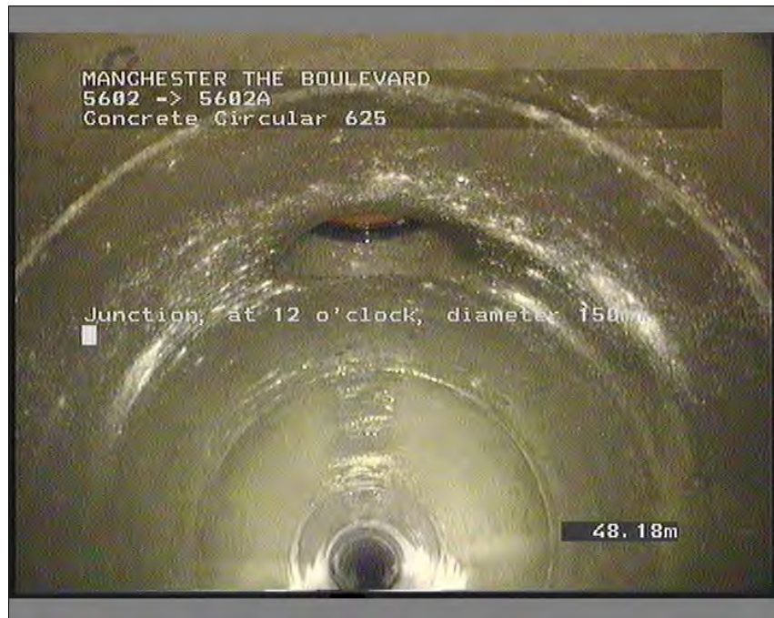
Photo: 3_3_9_A.JPG 48.18m, Junction, at 12 o'clock, diameter 150mm
