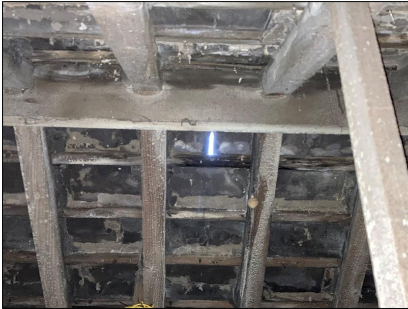
Photograph 23 showing the daylight seen where mortar has crumbled
