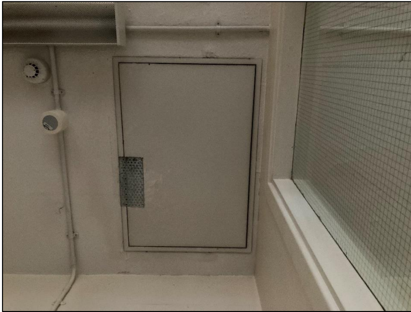
Photograph 19 showing the inaccessible loft hatch in the eastern section of the building
