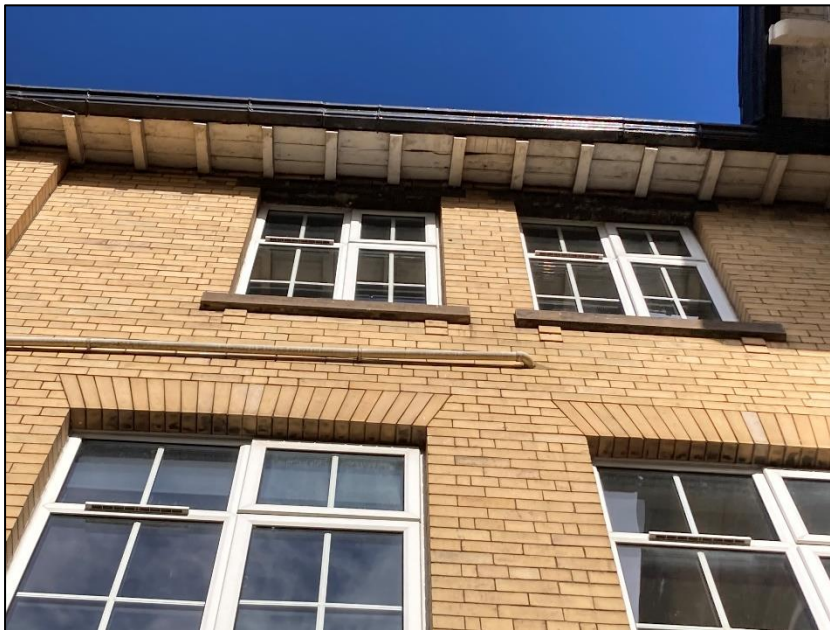
Photograph 18 showing the gaps at the eaves of the roof and damaged soffits
