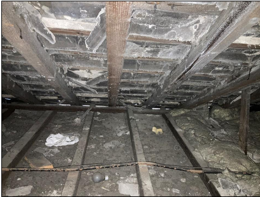
Photograph 25 showing daylight at the roof edges
