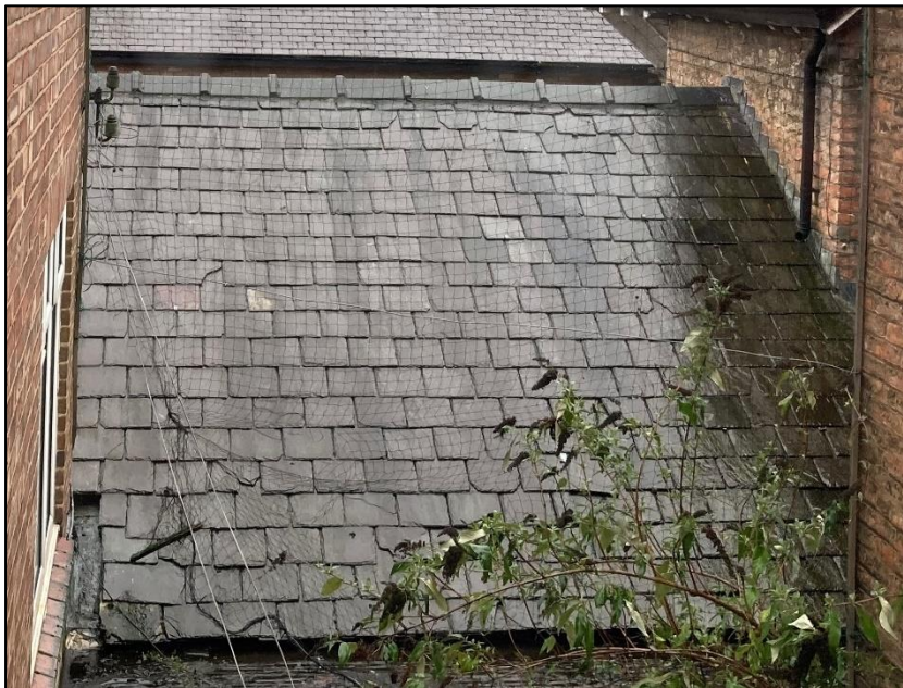
Photograph 16 showing some of the slipped and damaged roof slates
