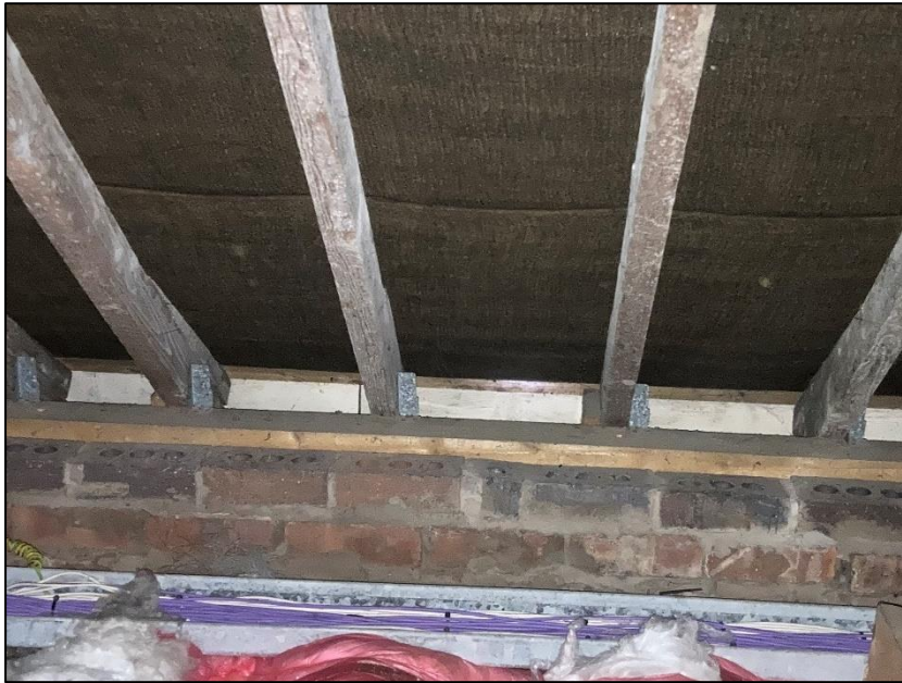
Photograph 41 showing daylight at the roof edges
