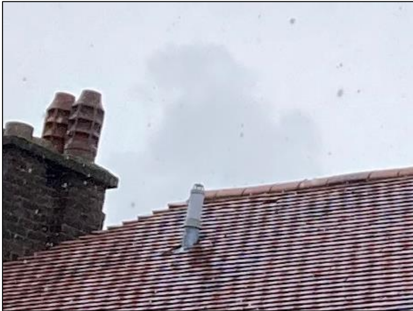
Photograph 35 showing the missing tile
