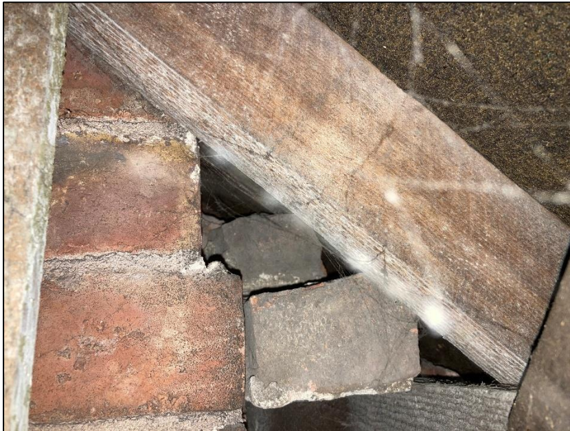
Photograph 40 showing a cavity at the roof apex
