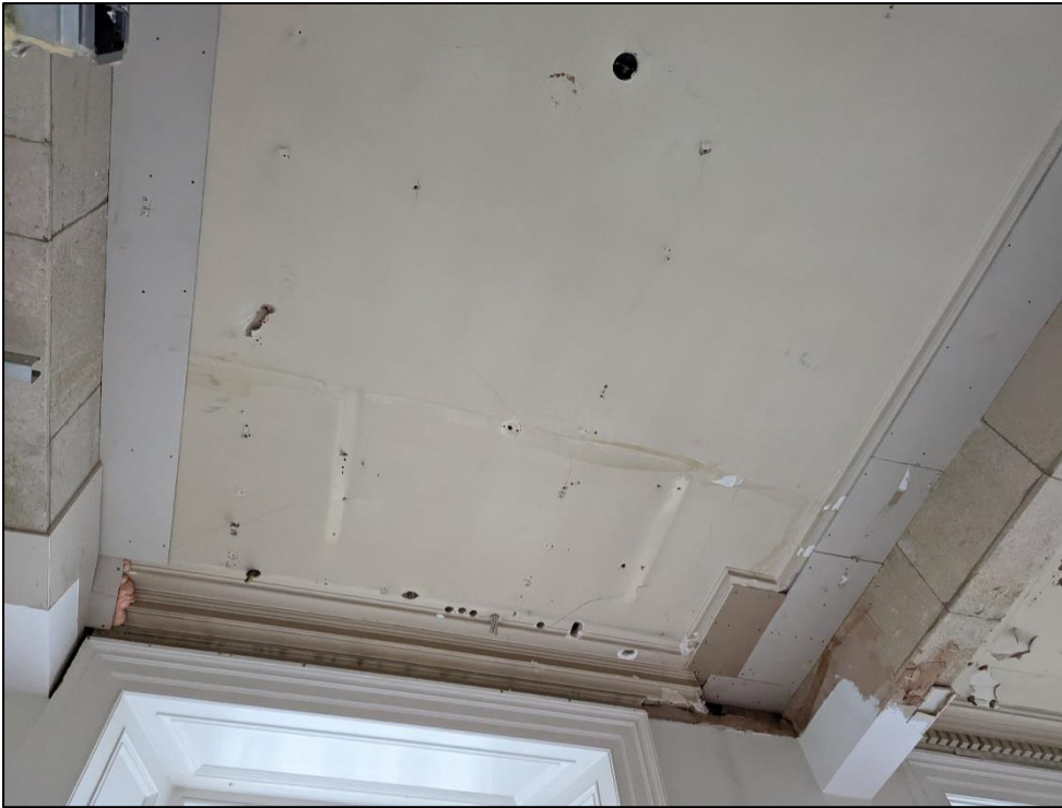
Plate 66: Detail of damaged cornice
