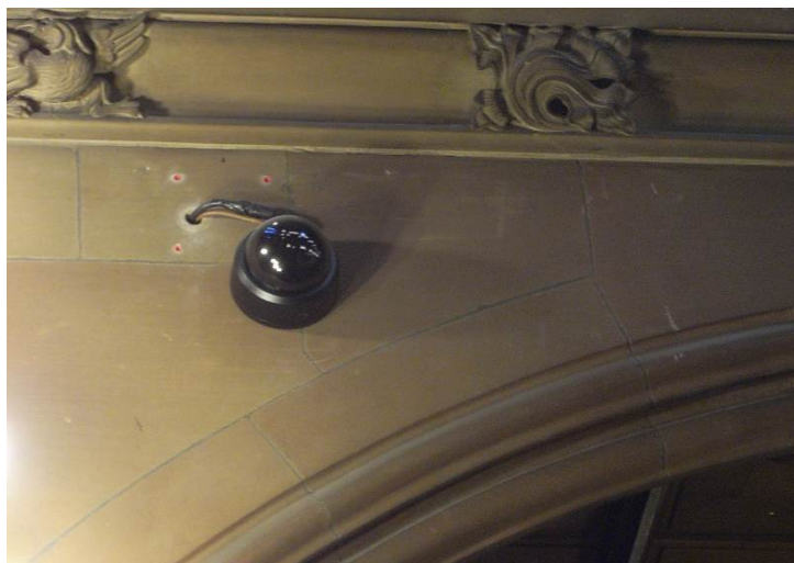
Fig 30. Inappropriate installation of CCTV camera
