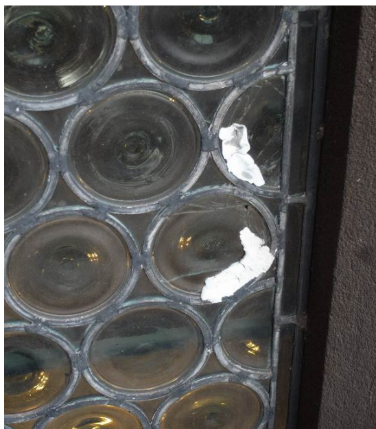
Fig 27. Example of inappropriate building repair
