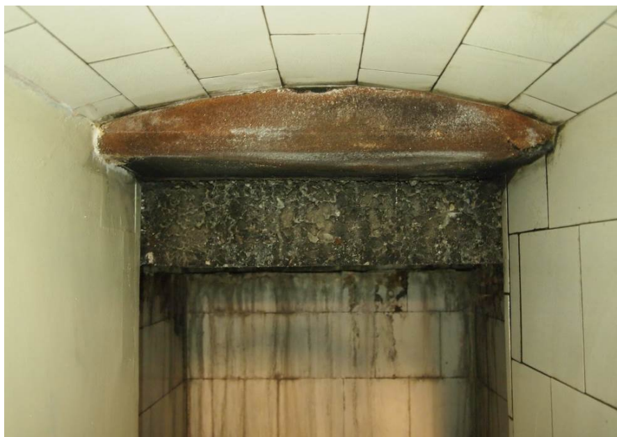
Fig 26. Water ingress to pavement light infills
