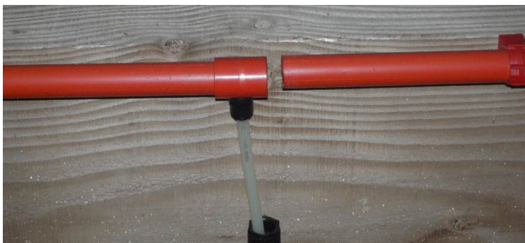
Fig 27. VESDA system within main roof void
