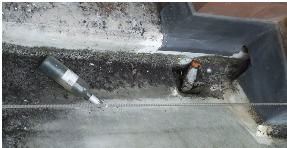
Fig 26. Example of inappropriate building maintenance
