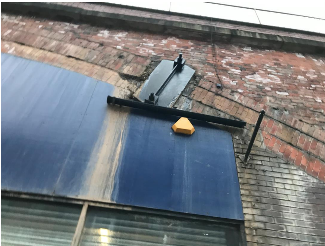
2) Failed guttering detail with the water bypassing the gutter and rinsing down the fascia.
