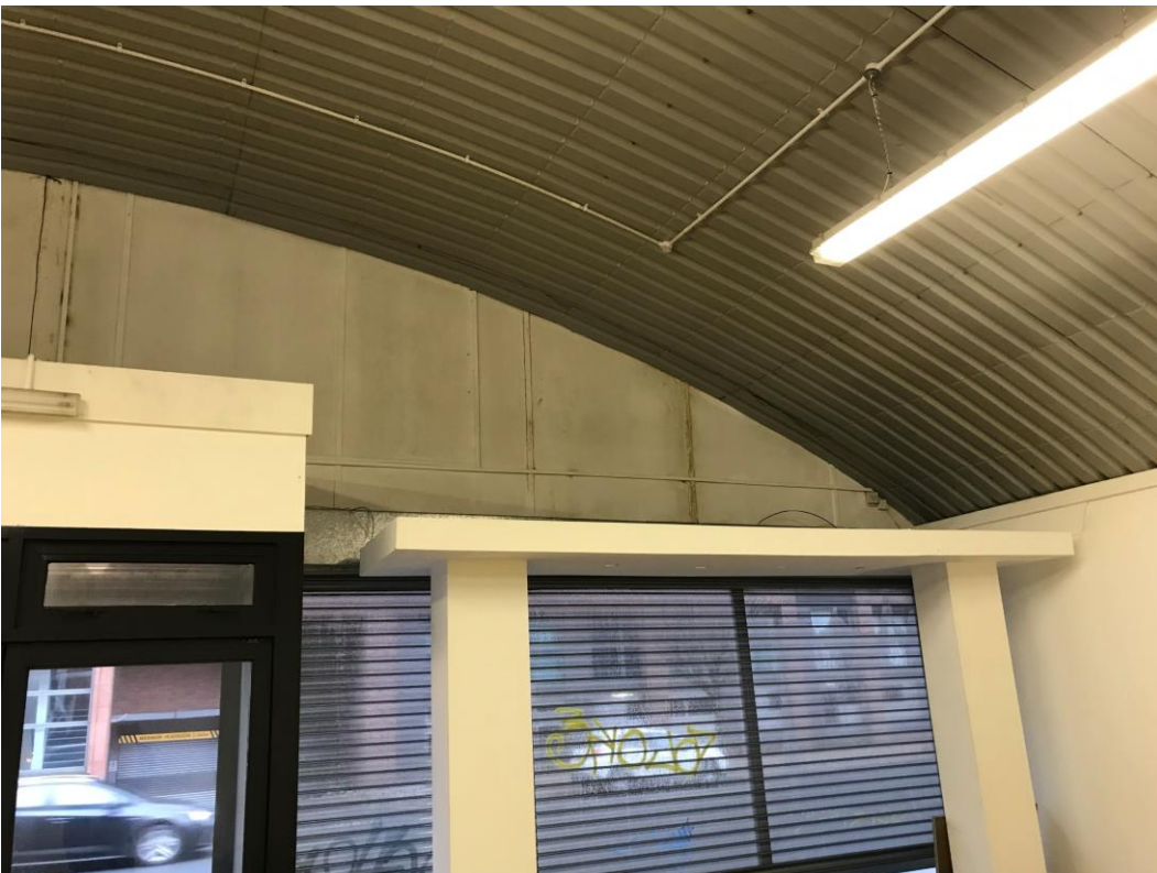
12) Stained wall lining.
