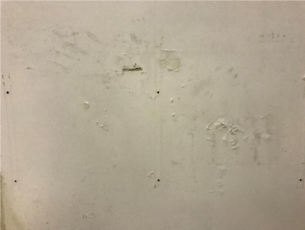
17) Damp affected paint finish.
