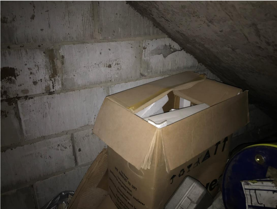
28) Debris to basement level.
