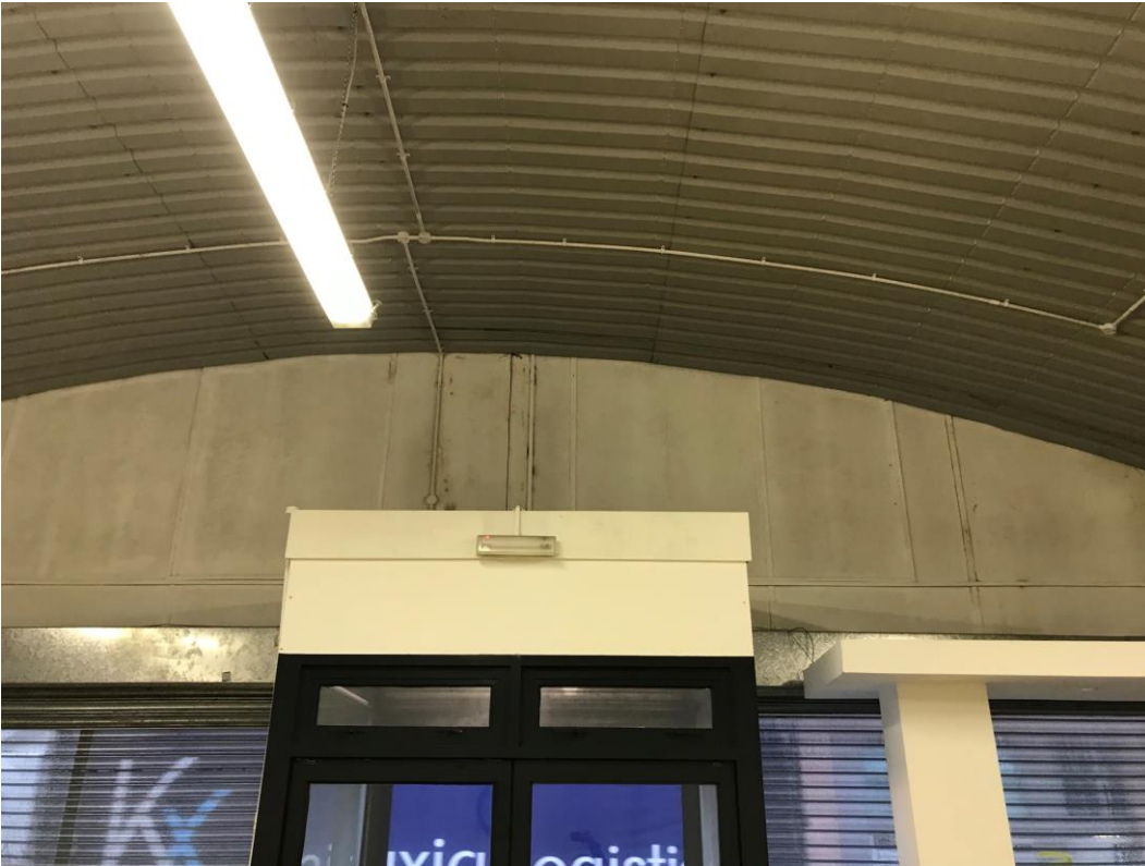
11) Stained wall lining.
