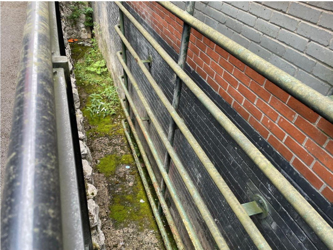
35) The rear emergency exit to 77 Whitworth Street West with the neighbouring retaining structure being built in close proximity, meaning that it is unsafe and impractical to use this exit.
