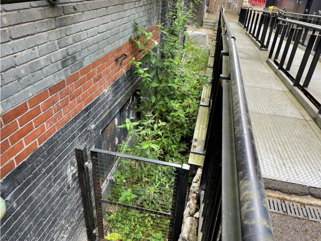
34) The rear emergency exit to 77 Whitworth Street West with the neighbouring retaining structure being built in close proximity, meaning that it is unsafe and impractical to use this exit.
