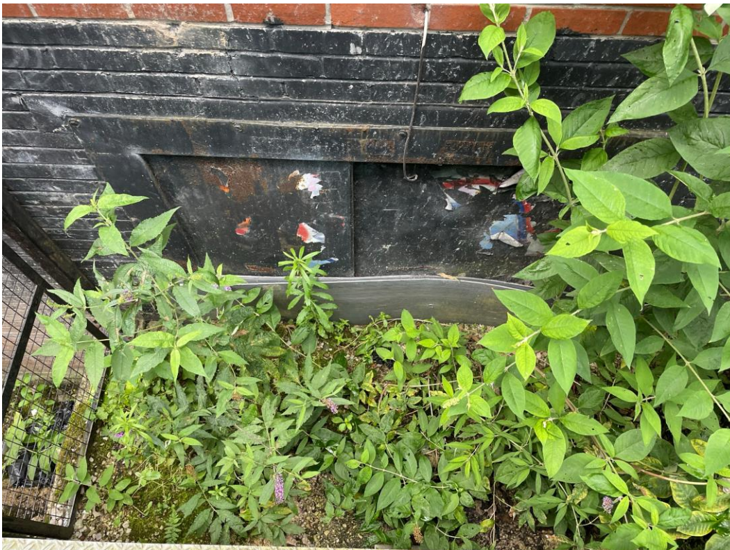
31) The rear emergency exit to 77 Whitworth Street West with the neighbouring retaining structure being built in close proximity, meaning that it is unsafe and impractical to use this exit.
