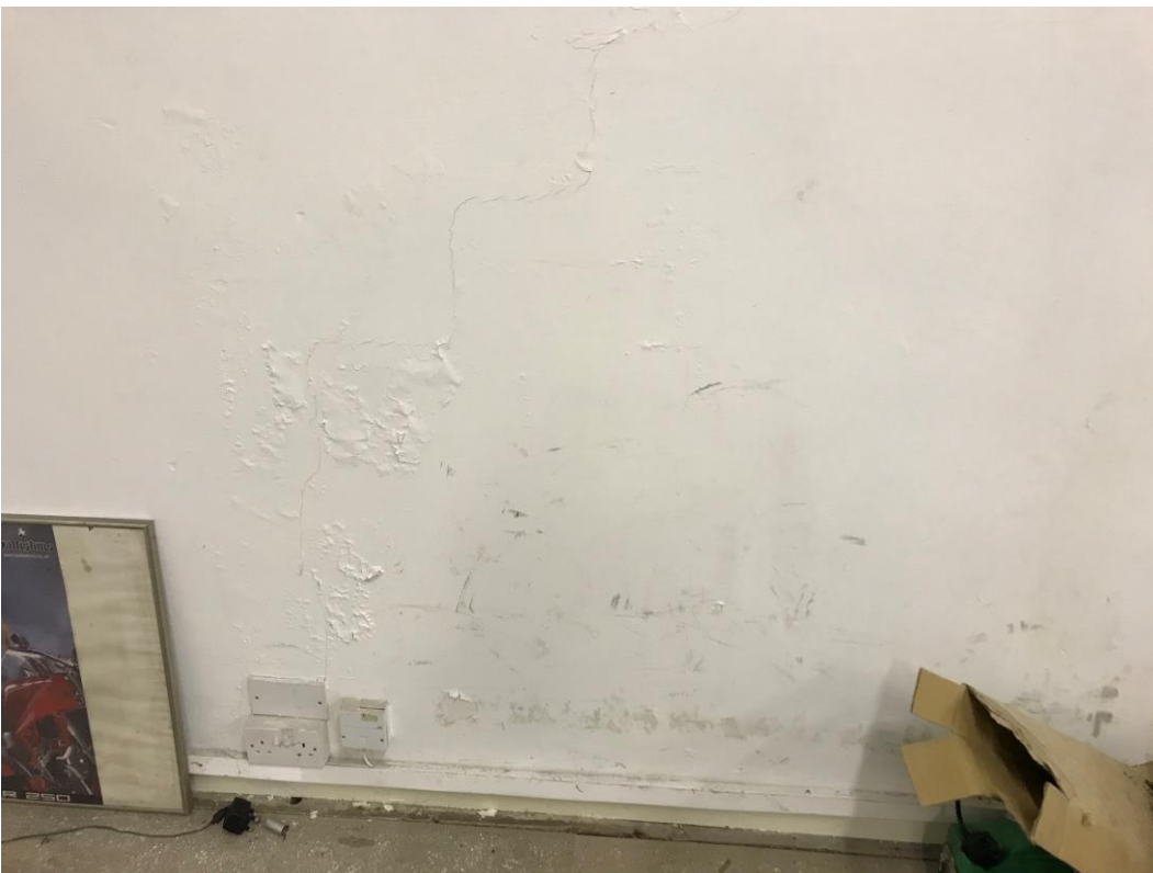
20) Damp affected paint finish.
