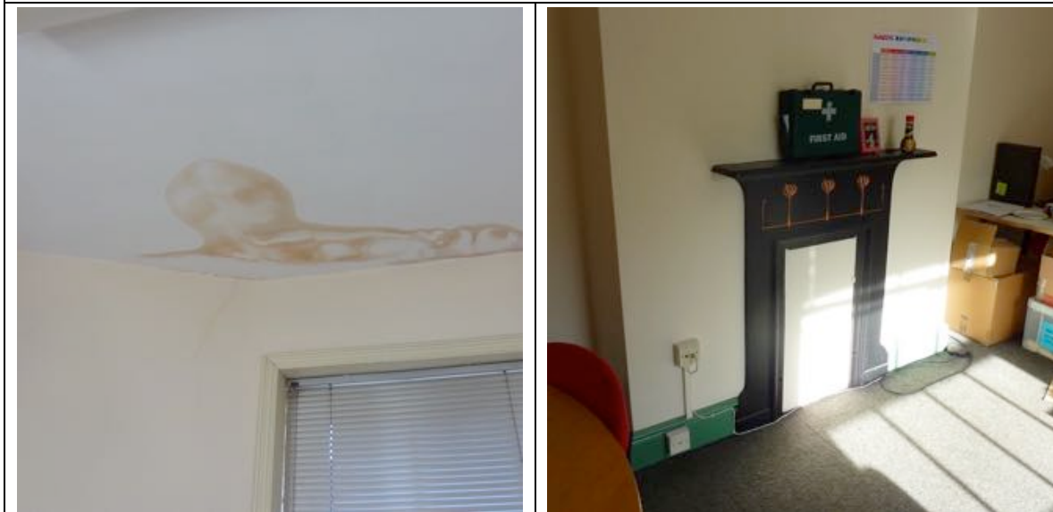
Damp staining to the edge of the ceiling at the west end but the wall otherwise free of the damp and salting on the floors above.
