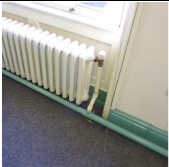
Rusting pipe connection to radiator. Very 'ordinary,' skirtings.
