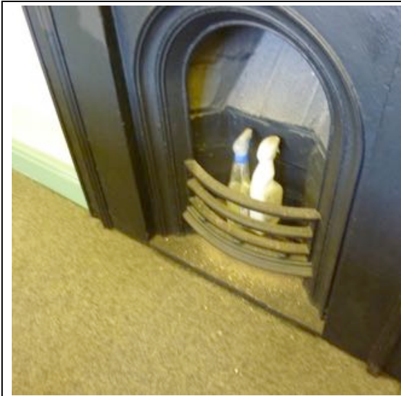
Dust in the fireplace shows this is an open flue.
