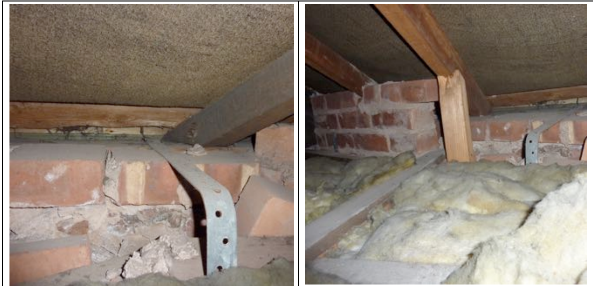
Shots into the eaves of the 'faceted roof' area. The brickwork is all a modern rebuild and looks bone dry.
