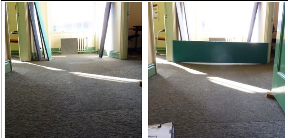
The floor of the lobby is distorted by 25mm over a short distance.
