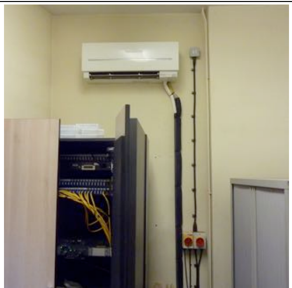
The room still has a large cabinet of data communications that is kept cool by the air-con unit.
