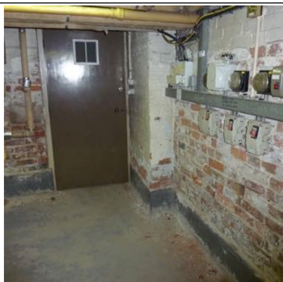
General view looking south east. The gas feed comes in across the ceiling from the adjacent room.
