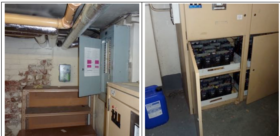
Main electrical panel for the building and a large battery back up unit.
