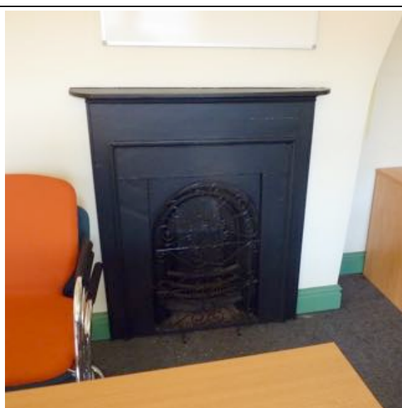
Fireplace has dust in the grate so must still be an open flue.
