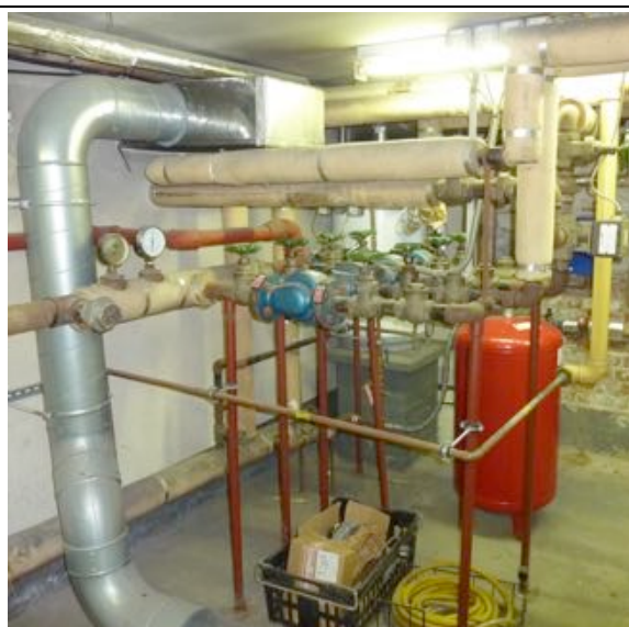
Boiler and manifold equipment. Some of this is live, some is cut off.
