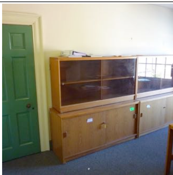
These cabinets would have imposed quite a load on the floor when full. No signs of any issues though.
