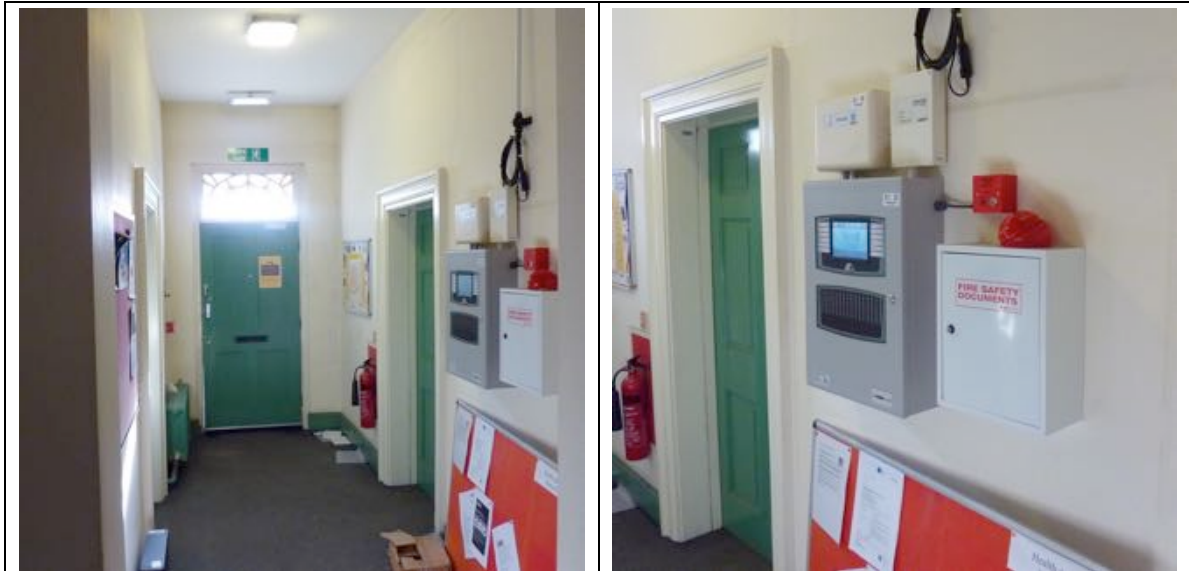
General view looking south to the front door. Main fire panel on the west wall.
