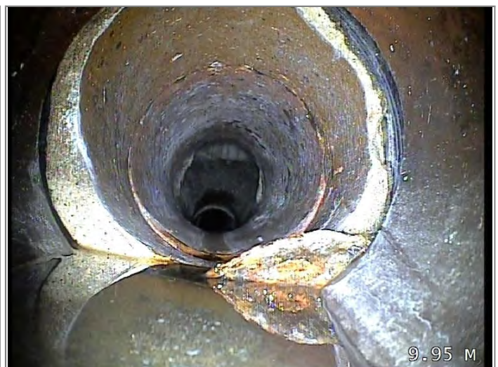
Joint displaced large - Remark: SEAL VISABLE - HOLDING WATER
