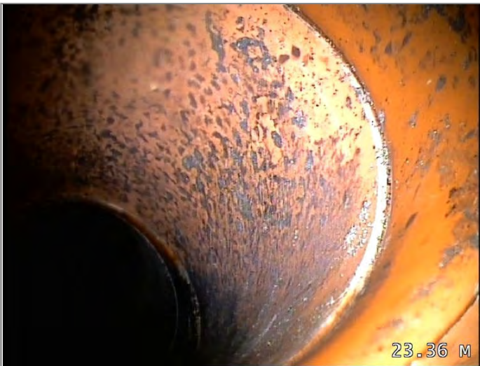
Line of drain/sewer deviates down
