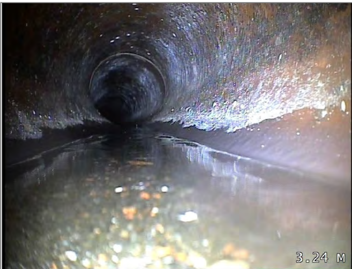
Settled deposits coarse 5% cross-sectional area loss
