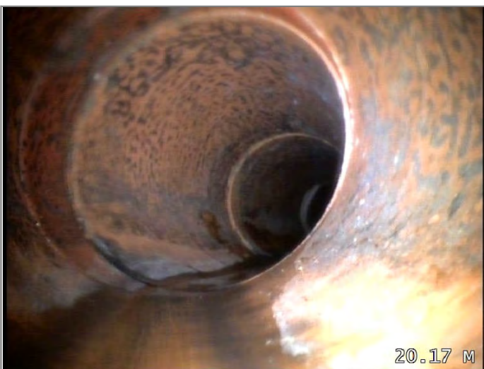
Line of drain/sewer deviates right
