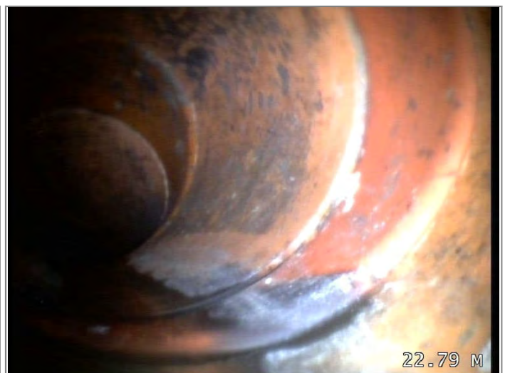
Line of drain/sewer deviates left
