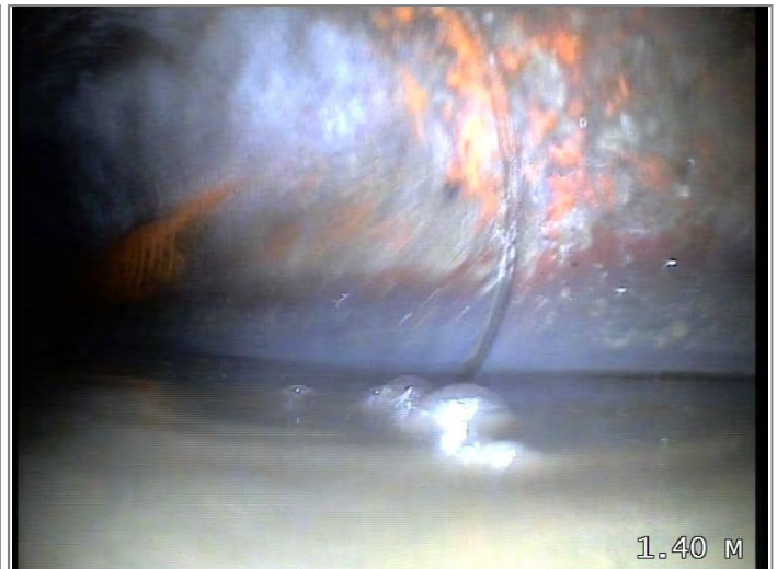
Line of drain/sewer deviates left
