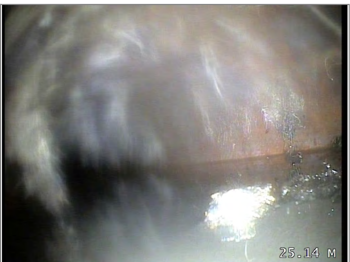
Settled deposits fine 20% cross-sectional area loss
