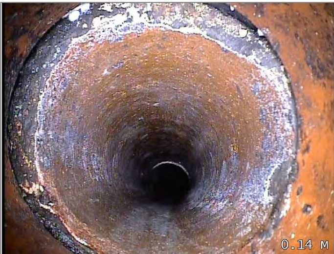
Joint displaced medium
