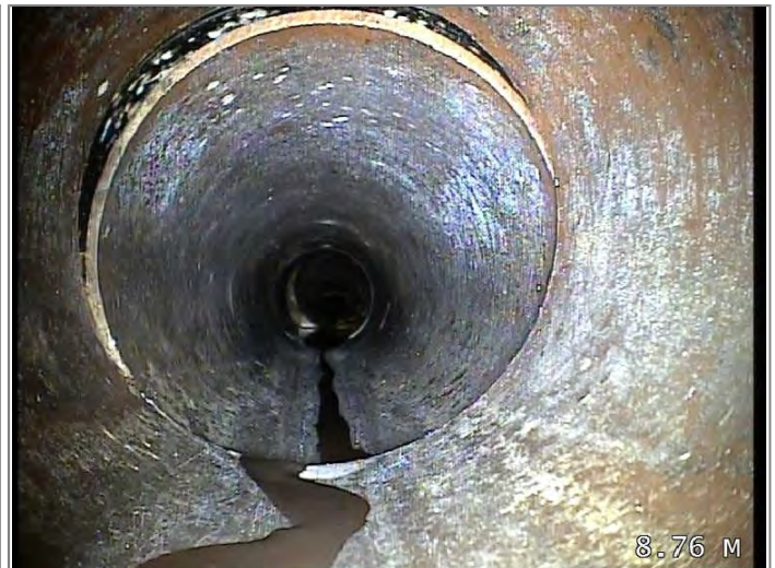
Joint displaced medium - Remark: SEAL VISABLE
