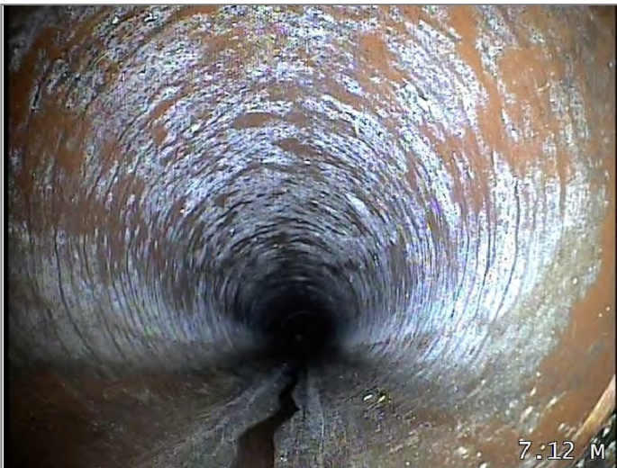
Line of drain/sewer deviates down
