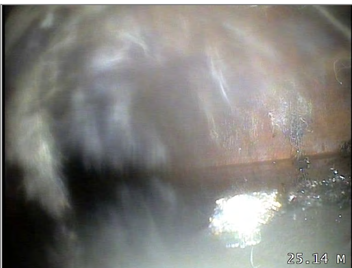
Line of drain/sewer deviates left
