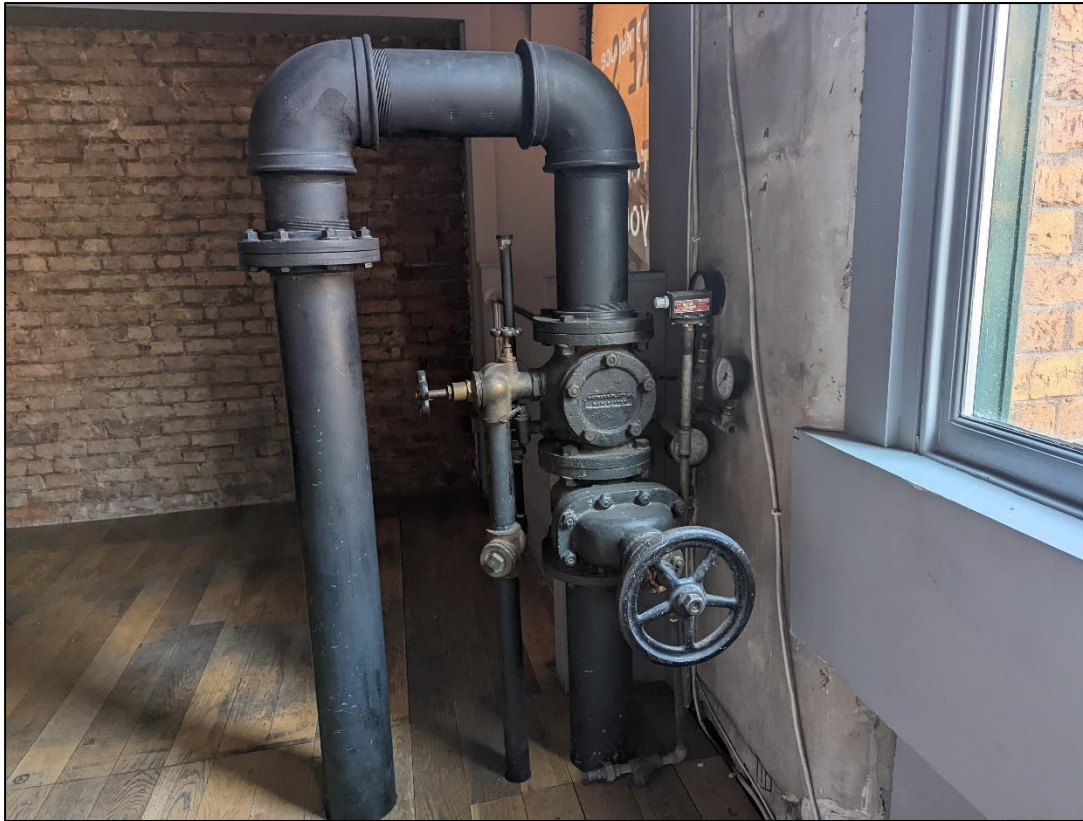
Plate 23: Cast iron sprinkler system
