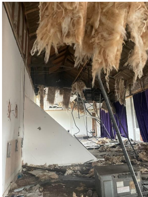
Figure 38: First floor space. Heavily altered and generally poor state. Evidence of original pitched roof and some brick detail.
