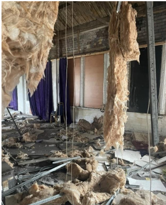
Figure 37: First floor space. Heavily altered and generally poor state. Evidence of original pitched roof and some brick detail.
