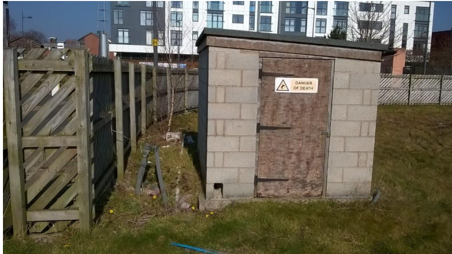
1) Electricity sub station north west corner of the site.
