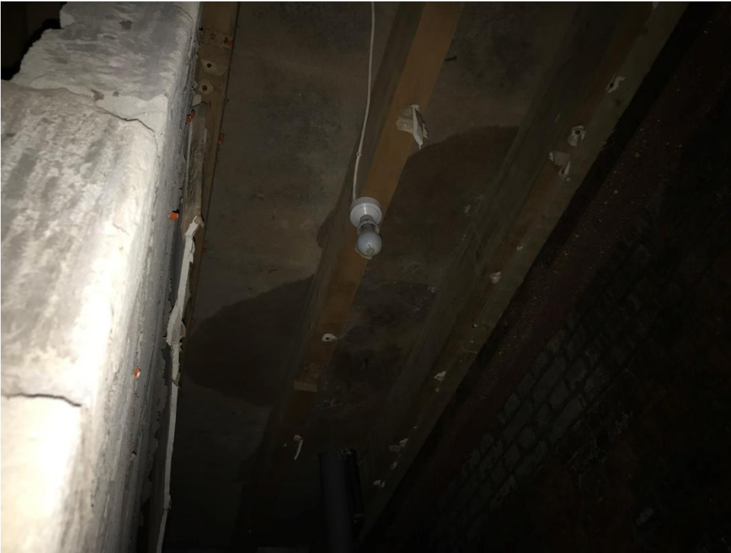
23) Underside of the mezzanine structure, which is damp affected and not fit for purpose.
