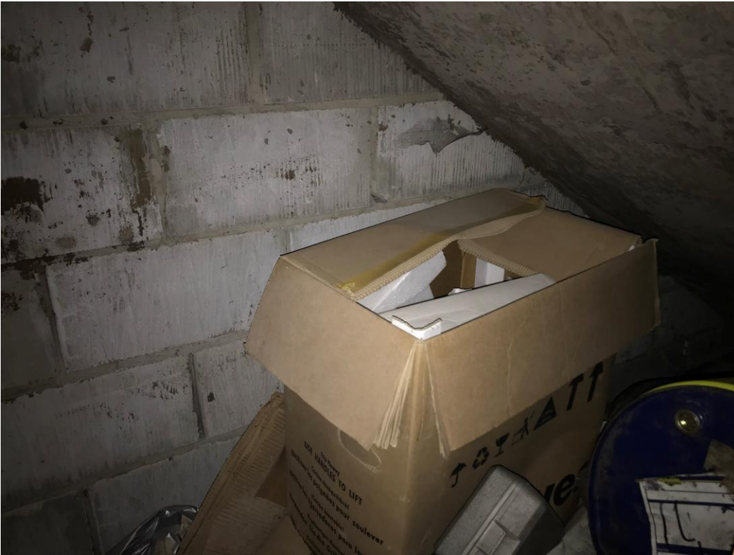
28) Debris to basement level.
