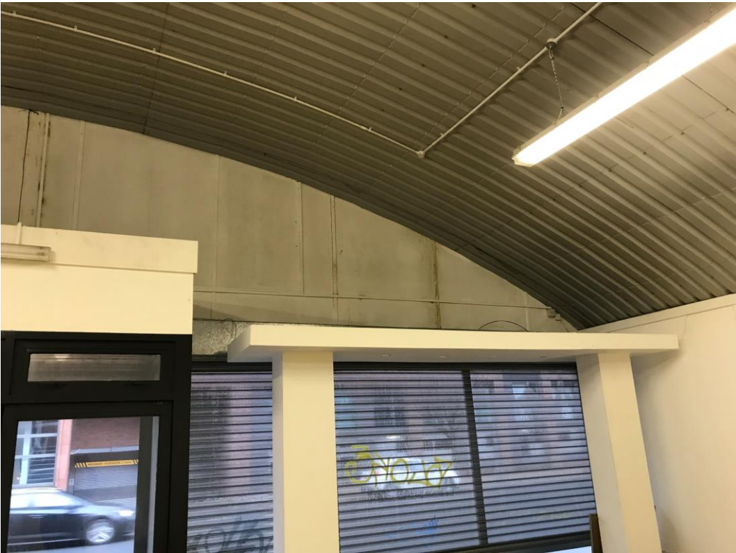
12) Stained wall lining.
