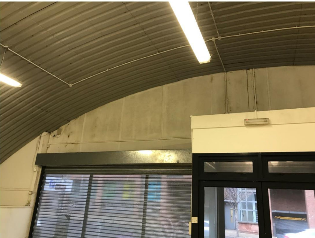
10) Stained wall lining.
