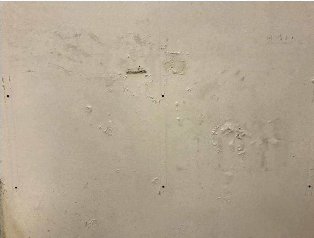
17) Damp affected paint finish.
