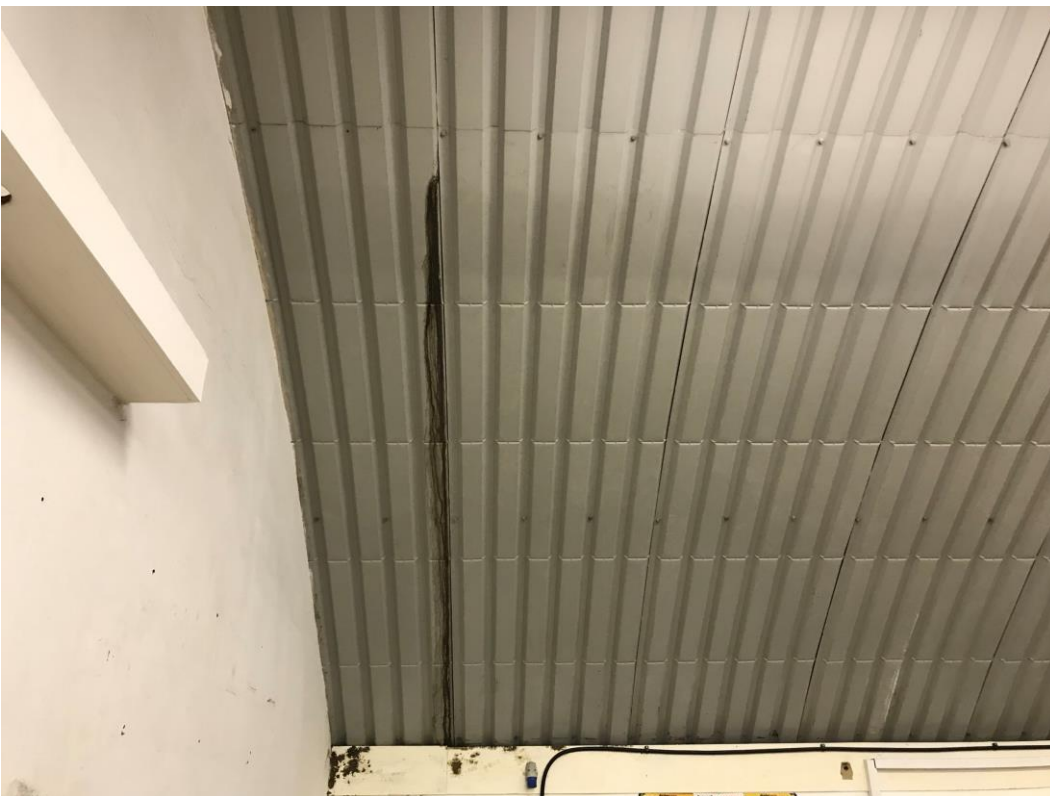
16) Isolated location of leak coming through the lining system.
