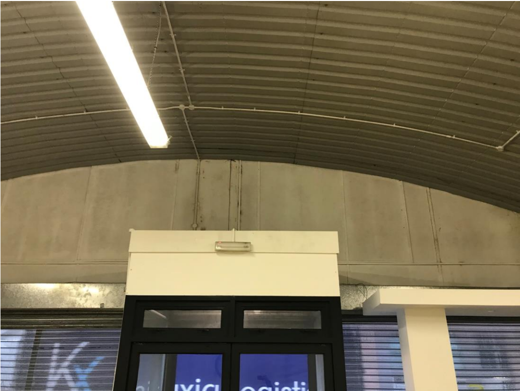
11) Stained wall lining.
