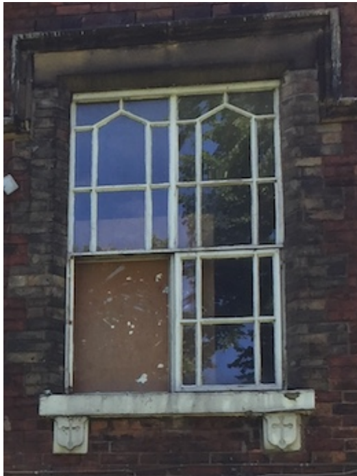
Missing casement at first floor front elevation to be replaced to match existing
