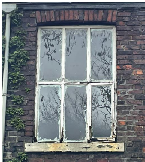
Rotten window frame at first floor rear elevation to be replaced to match existing
