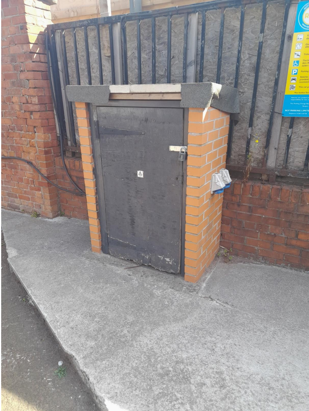
Electrical box on western boundary of site.
