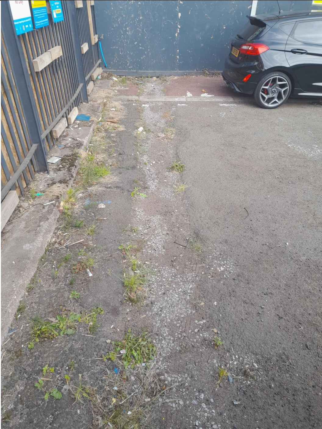
Tarmac scarring noted indicating buried services
