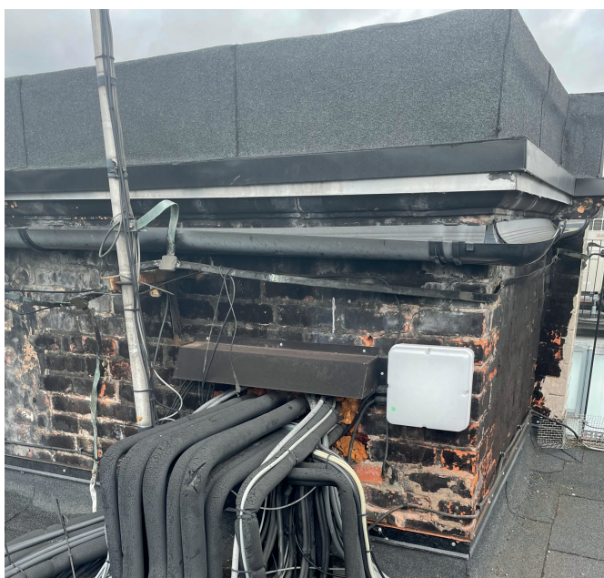
Image 11: Existing cable feeds through historic brickwork to Tootal Building roof.
