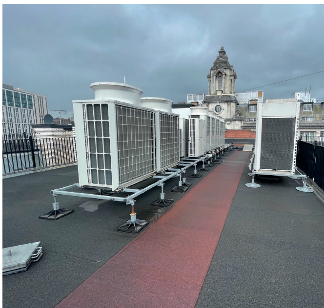
Image 10: Existing air handling units on new roof surface on Tootal Building.
