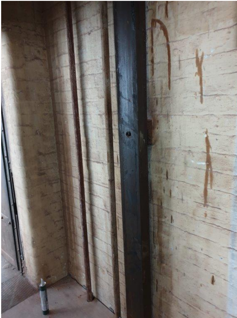
Image 3.6: Within lift core. Hoist operatus.
