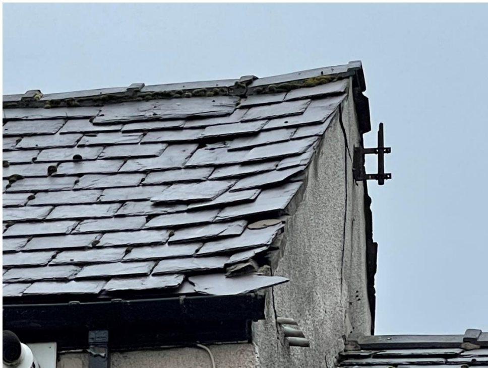
2. Gable end with slipped and missing tiles.
