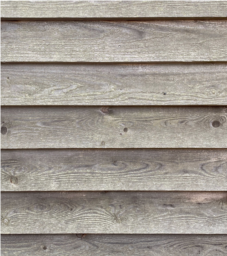
Untreated Douglas fir cladding, 16 years after installation. The cladding shows signs weathering including bleaching, isolated staining, and delignification. The performance is not affected however.
