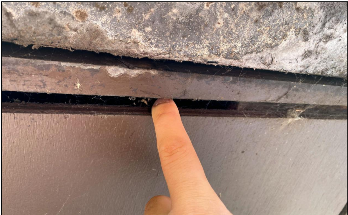
Plate 8: The soffits were generally intact although they were not well sealed and may offer low level Roosting Potential.
