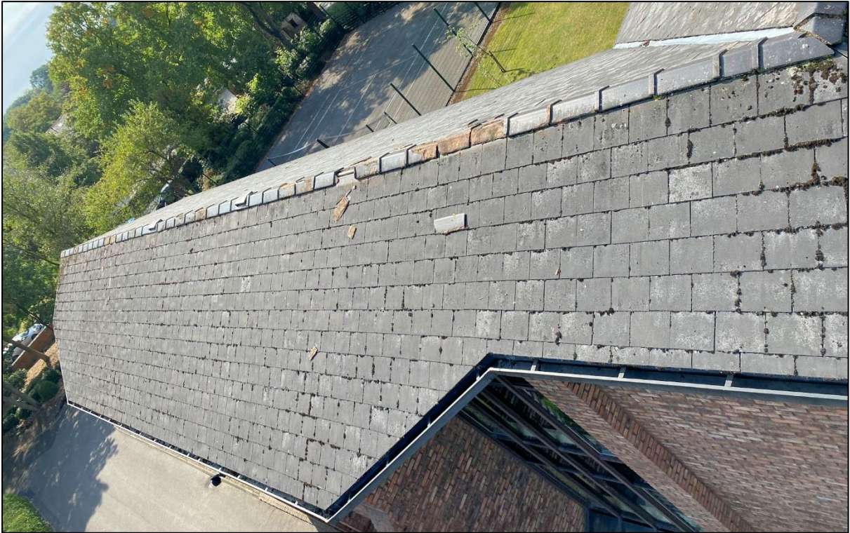
Plate 2: General roof view from MEWP broken and missing ridge tiles were apparent.
