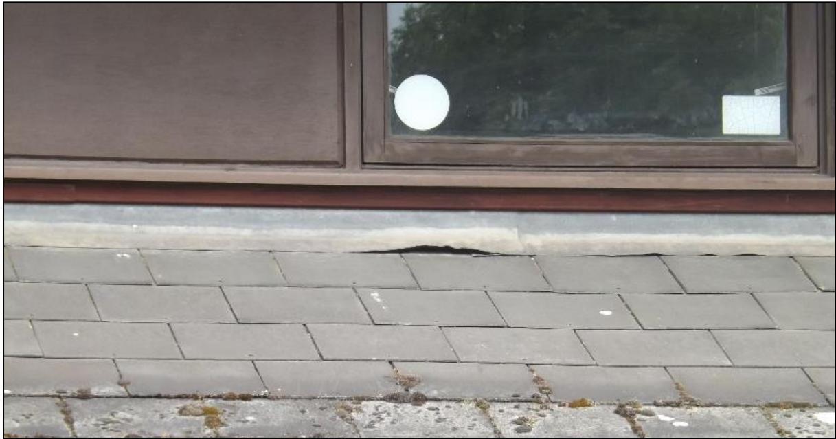
Plate 11: The flashing around window frames was not flush in places, leaving Potential Roosting space underneath.
