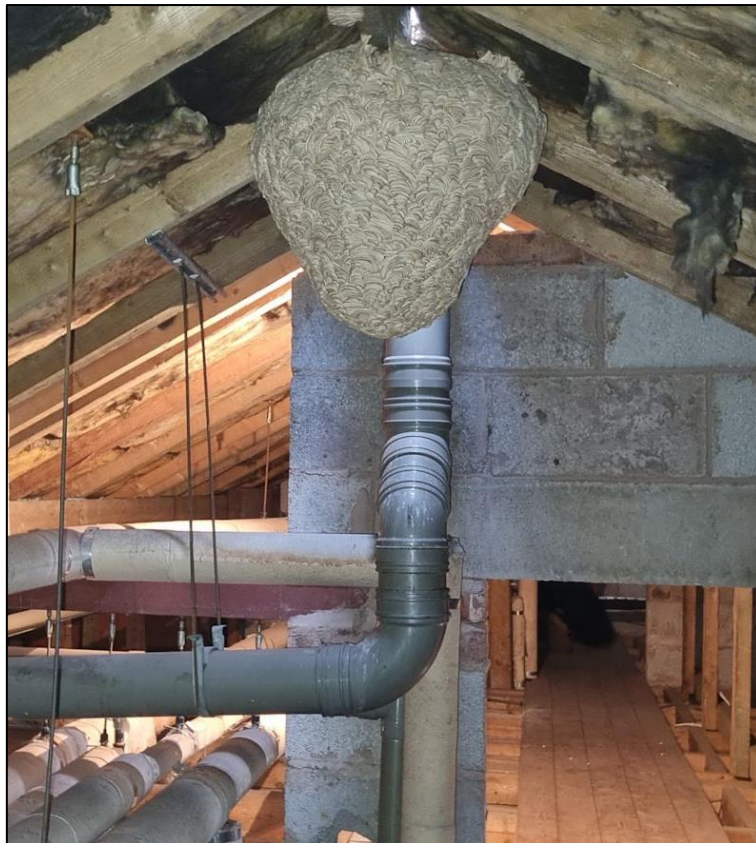
Plate 19: A number of wasp nests were also identified with a substantial nest in a Ewings roof void
