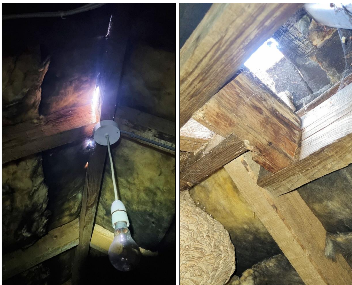
Plate 14: Gaps in the ridges identified externally allowed potential access to the internal voids.
