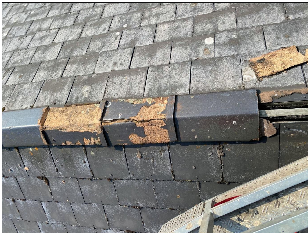
Plate 3: Missing and broken ridge tiles were apparent across the roofs.
