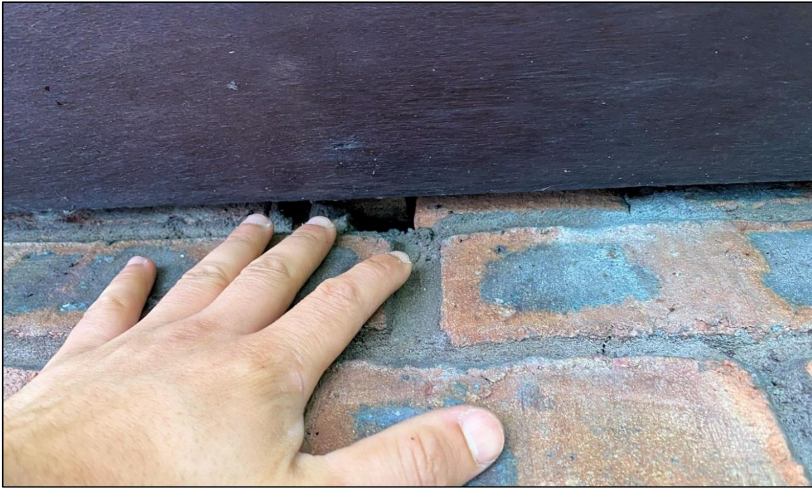
Plate 9: Gaps were apparent around the soffits providing potential access to internal roosting opportunities.
