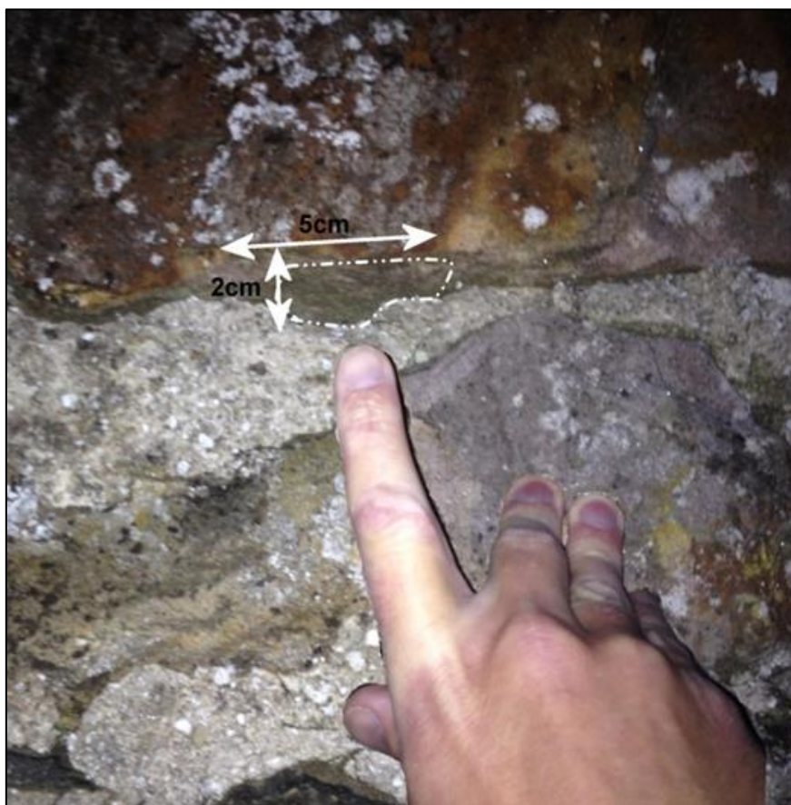
Plate 24: Example of an existing bat roost entrance (2cm by 5cm crevice).
