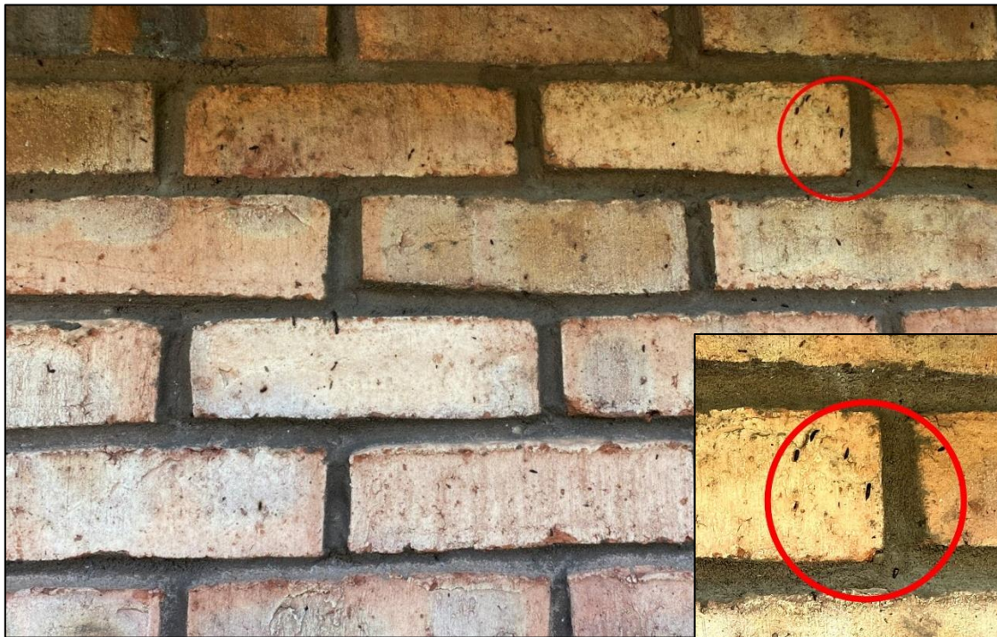
Plate 10: There were numerous bat droppings on a north facing aspect of Ewings (see inset).
