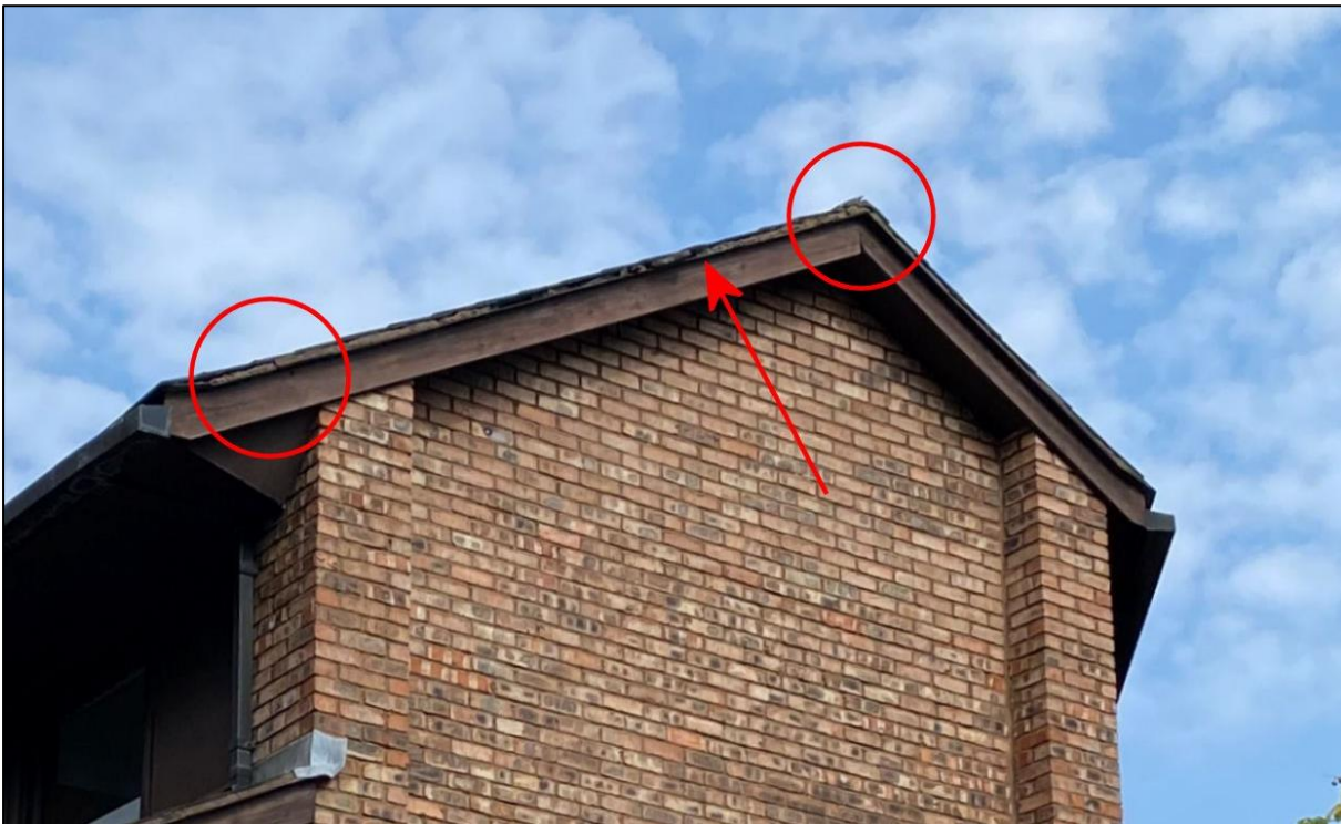
Plate 6: Numerous gaps were apparent in the verges of the buildings.
