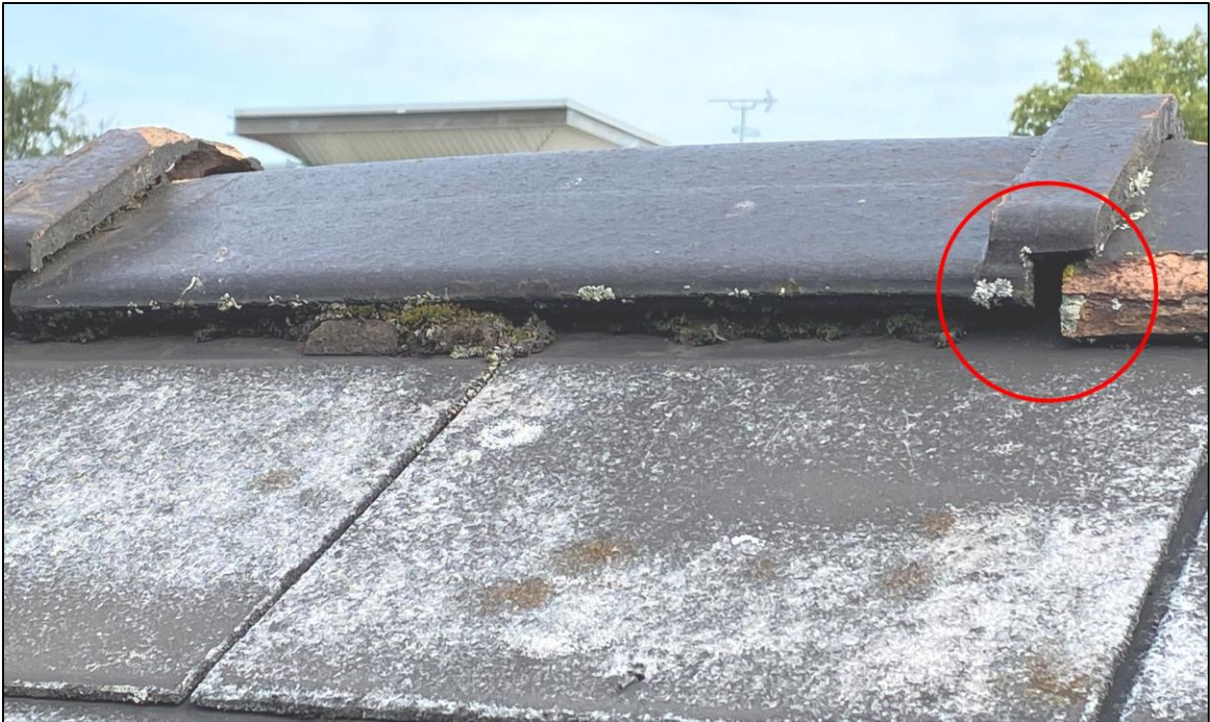
Plate 5: Even where ridge tiles were intact there were significant gaps beneath them.
