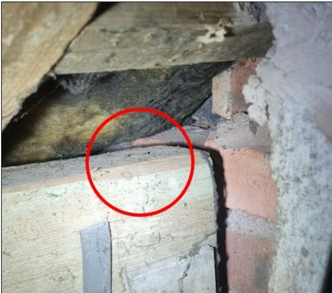
Plate 17: Elsewhere there was further evidence of bat activity in the form of droppings by Ewings' gable wall.
