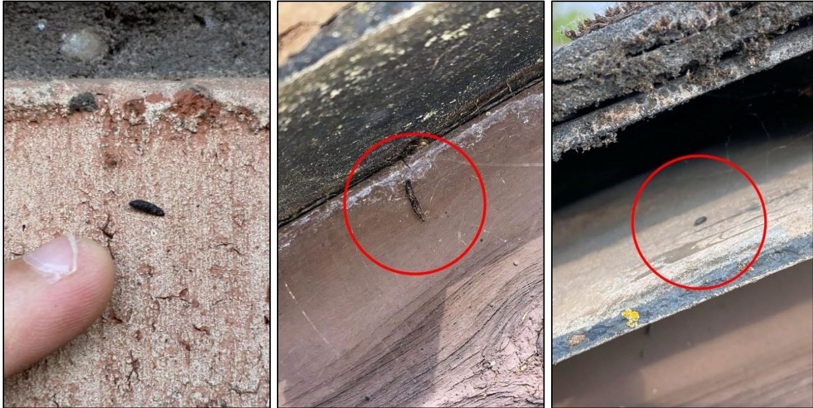
Plate 7: Droppings were identified within and below the verges of the building.
