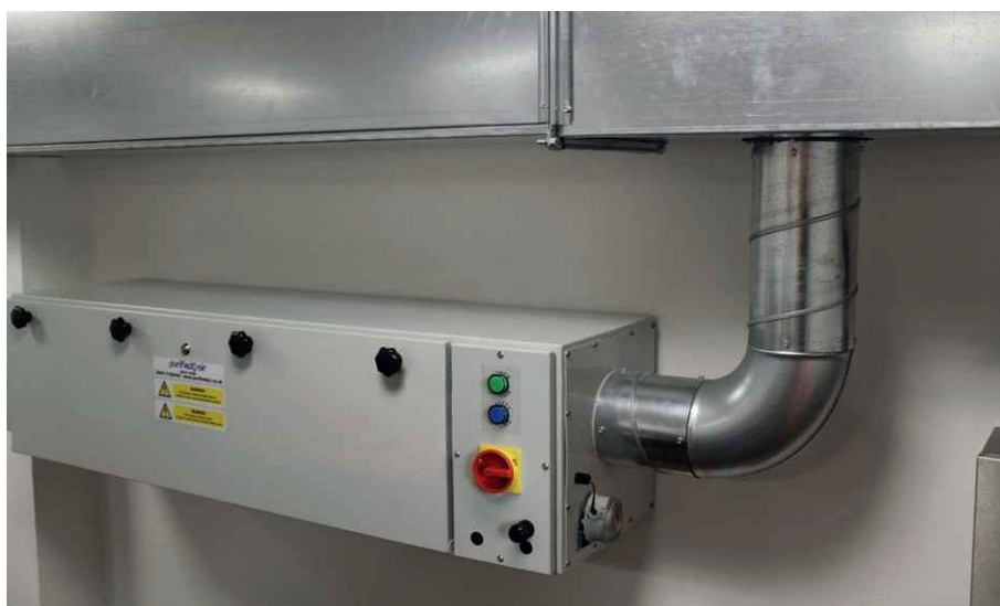
Figure 6 - UV-O 1000 Unit Installed
