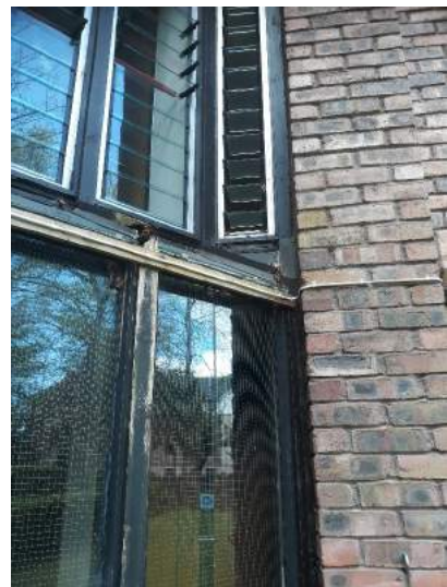
Examples of failed windows
