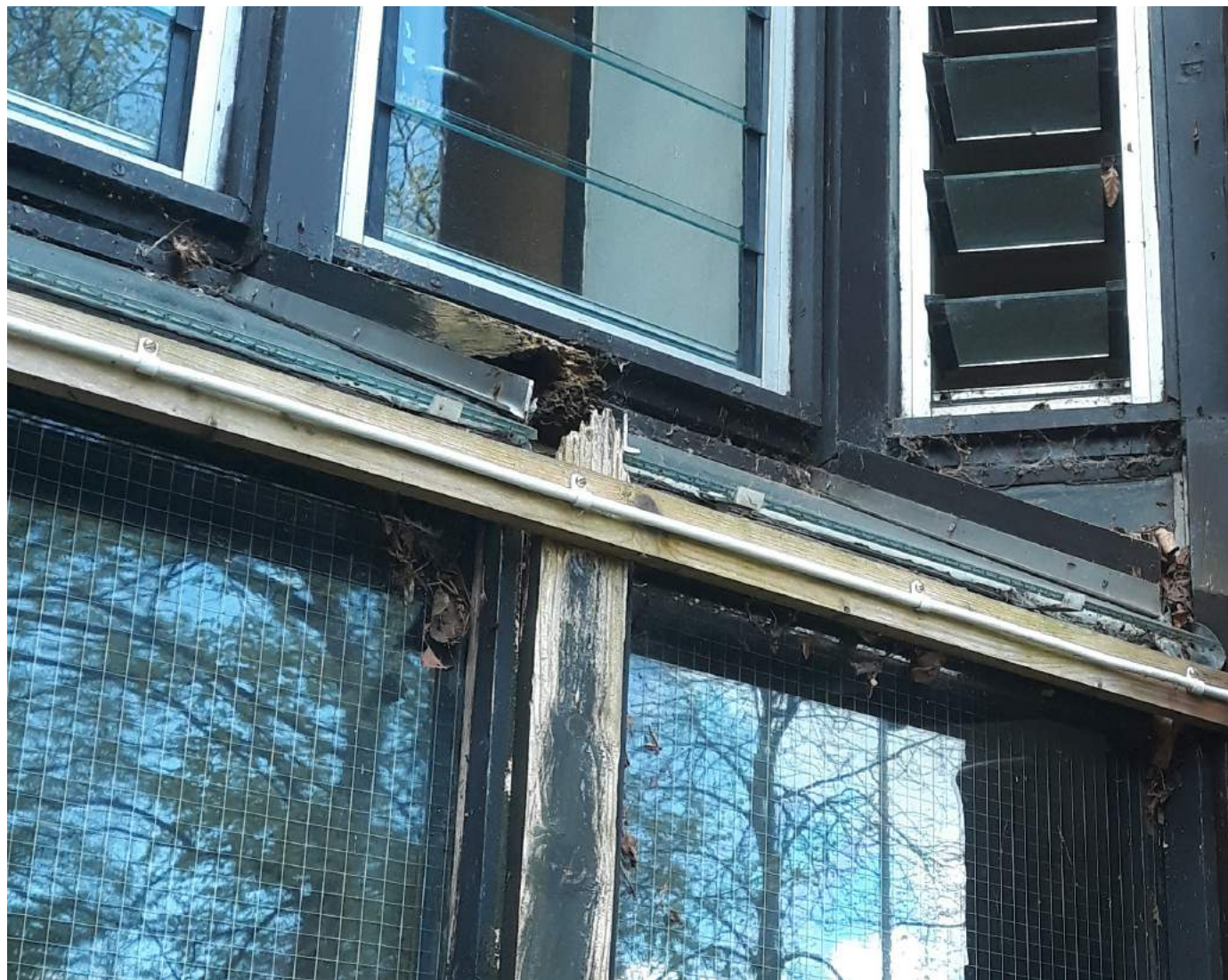
Examples of failed windows
