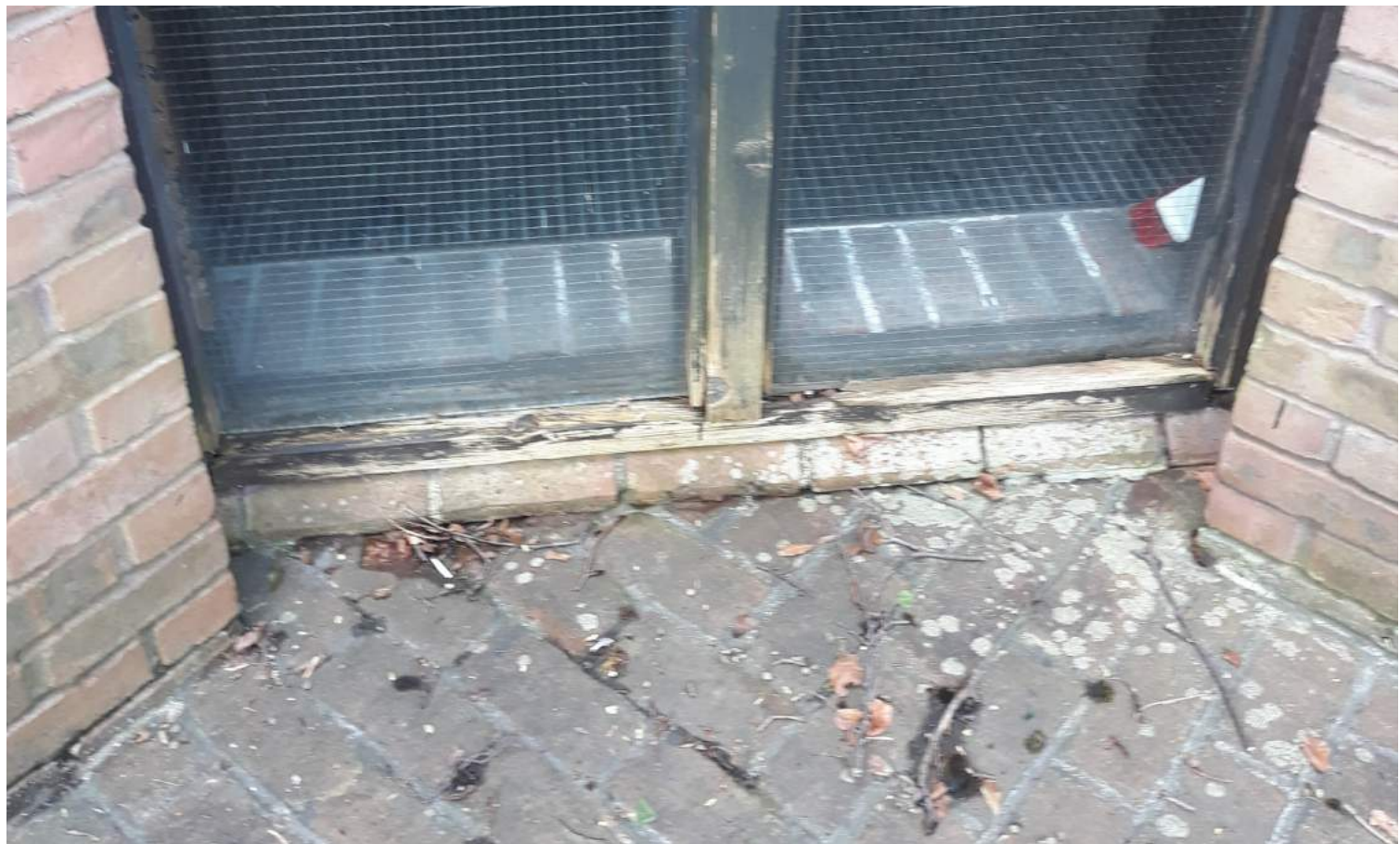
Examples of failed windows
