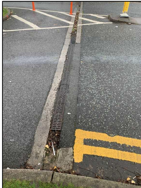
Damaged and blocked drainage system
