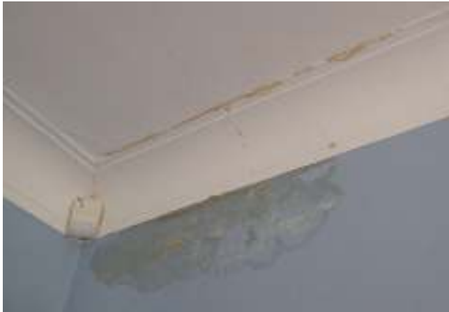
Damage from a leak in a bedroom
